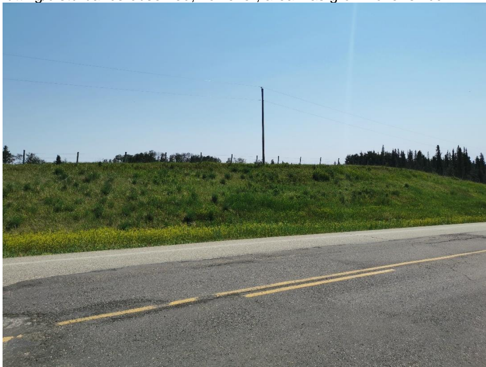
Photo 6 – Looking northeast at backslope slumps just south of the power pole.
