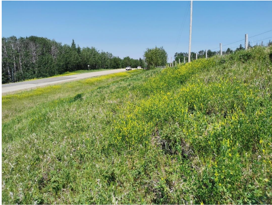
Photo 7 – Looking north at slumping backslope below power pole with open tension cracks.
