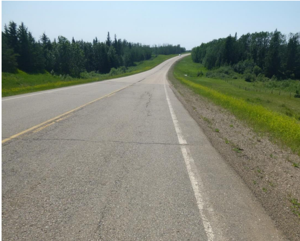
Photo 3 – Looking south at potential extension of slide-related cracks.
