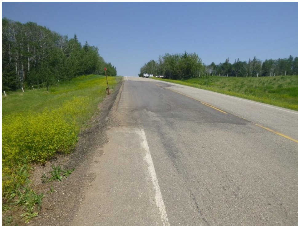
Photo 2 – Looking north at main crack and dip in highway surface.
