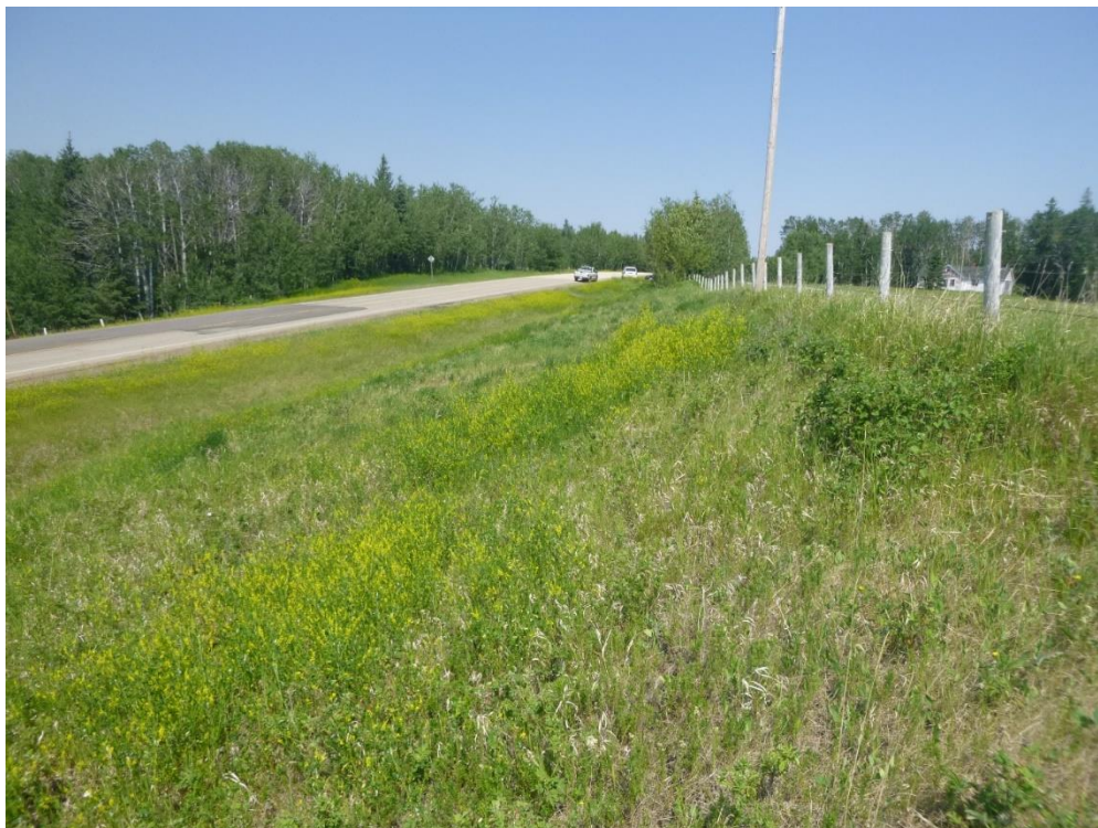
Photo 8 – Looking northwest from the backslope at the subsiding area in the pavement.
