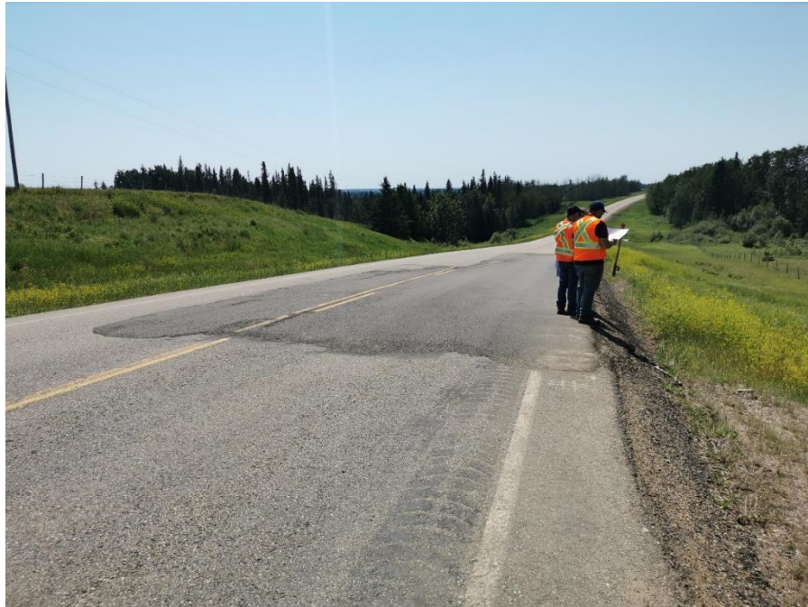
Photo 1 – Looking south at main crack and dip area that was patched. Significant thickness of asphalt visible at the edge of the pavement.
