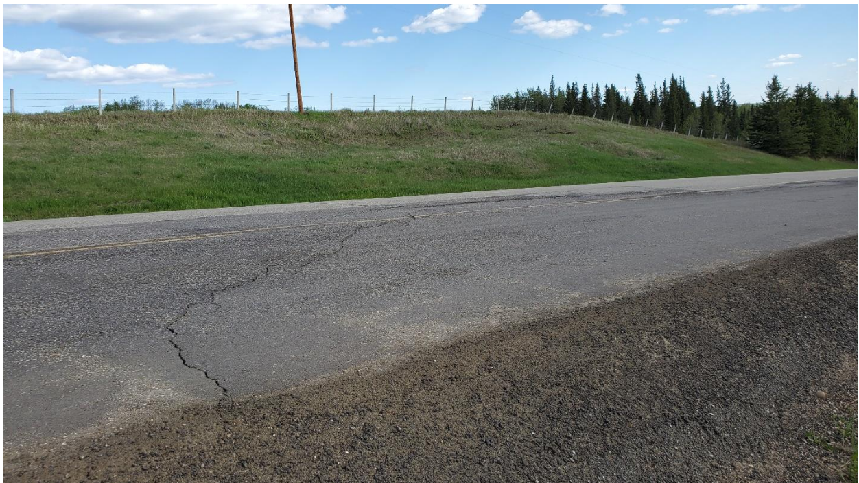
Photo 4 – Looking southeast at north end of crack pattern.
