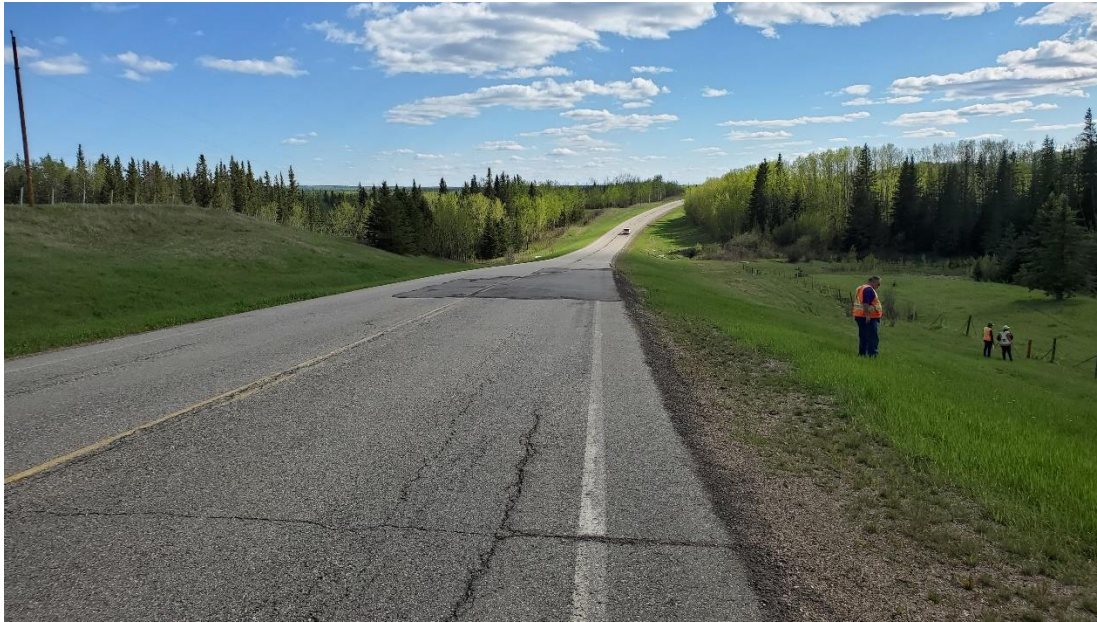
Photo 1 – Looking south at main crack and dip area that was patched. Significant thickness of asphalt visible at the edge of the pavement.
