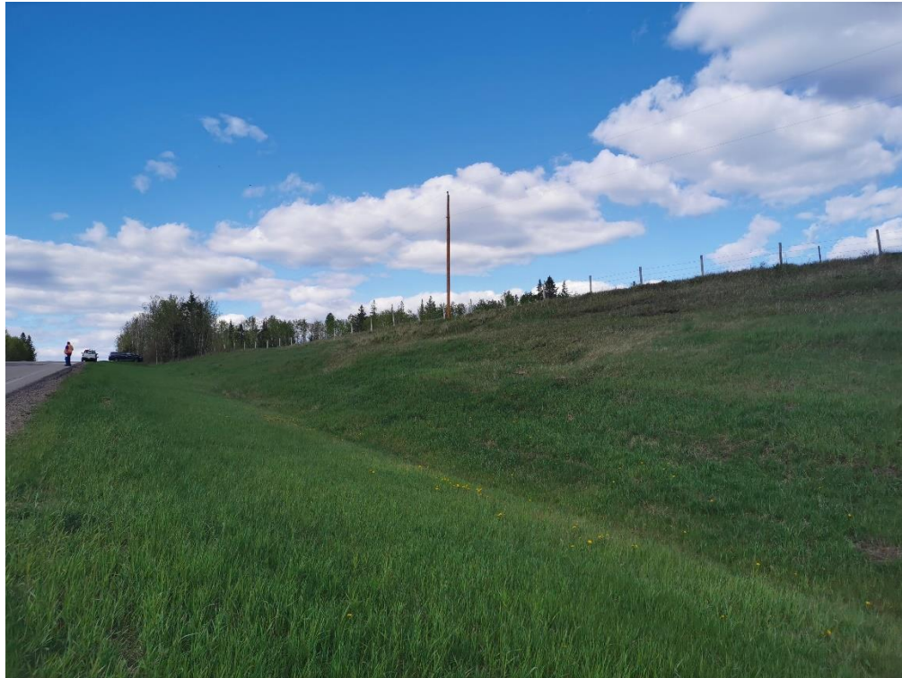
Photo 7 – Looking northeast at backslope slumps just south of the power pole.
