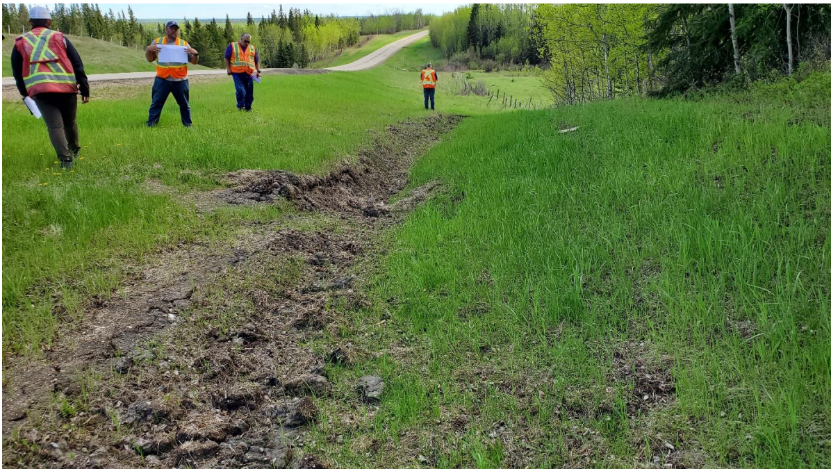
Photo 10 – Looking south at rutting in west ditch at the north end of the site.
