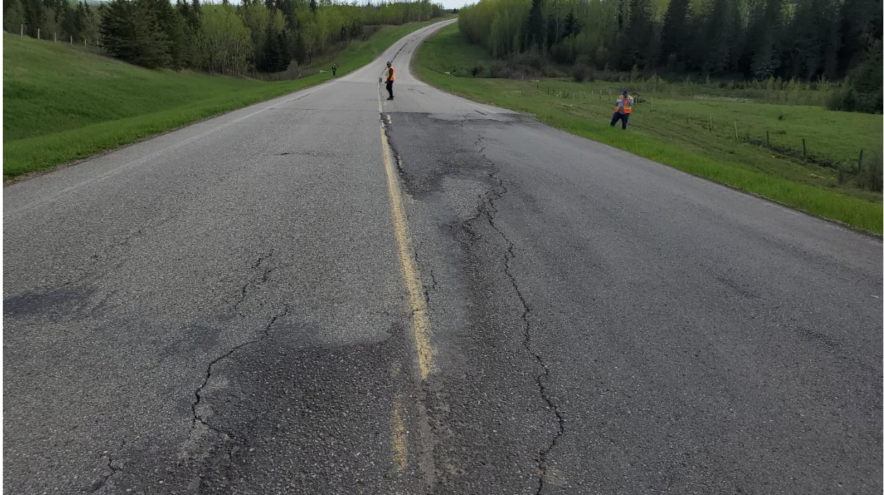
Photo 3 – Looking south at differential across crack near SI02-4 (no longer functional).
