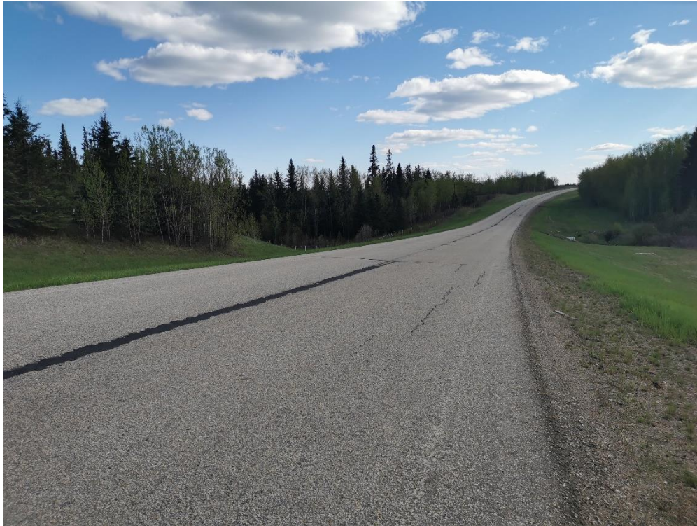
Photo 5 – Looking south at potential extension of slide-related cracks.
