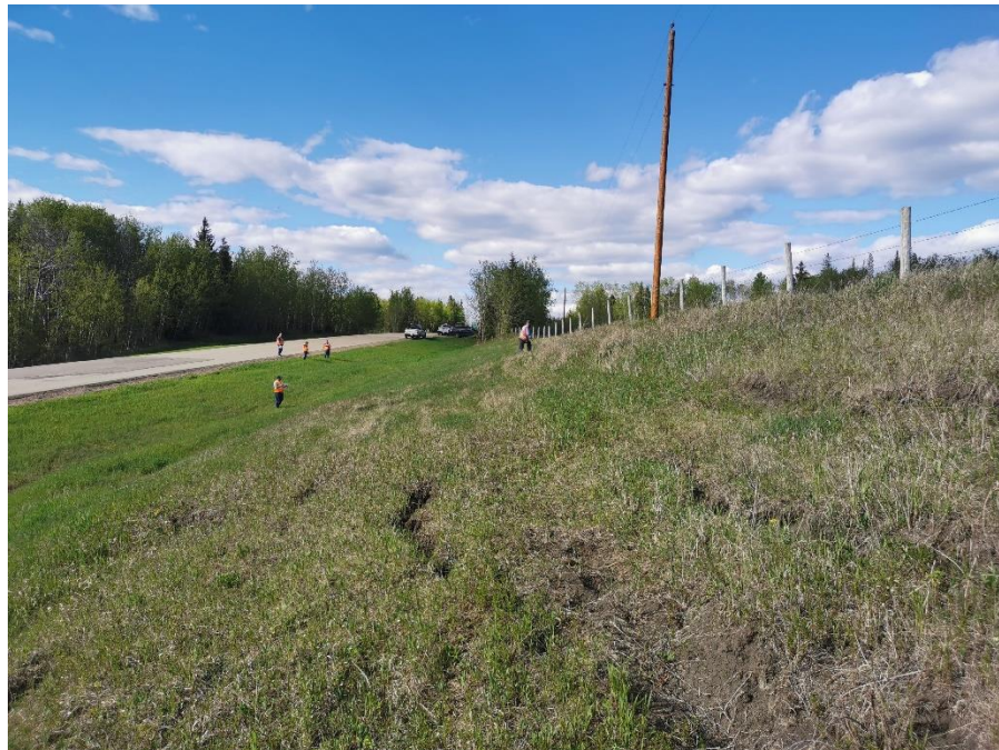
Photo 8 – Looking north at slumping backslope below power pole with open tension cracks.
