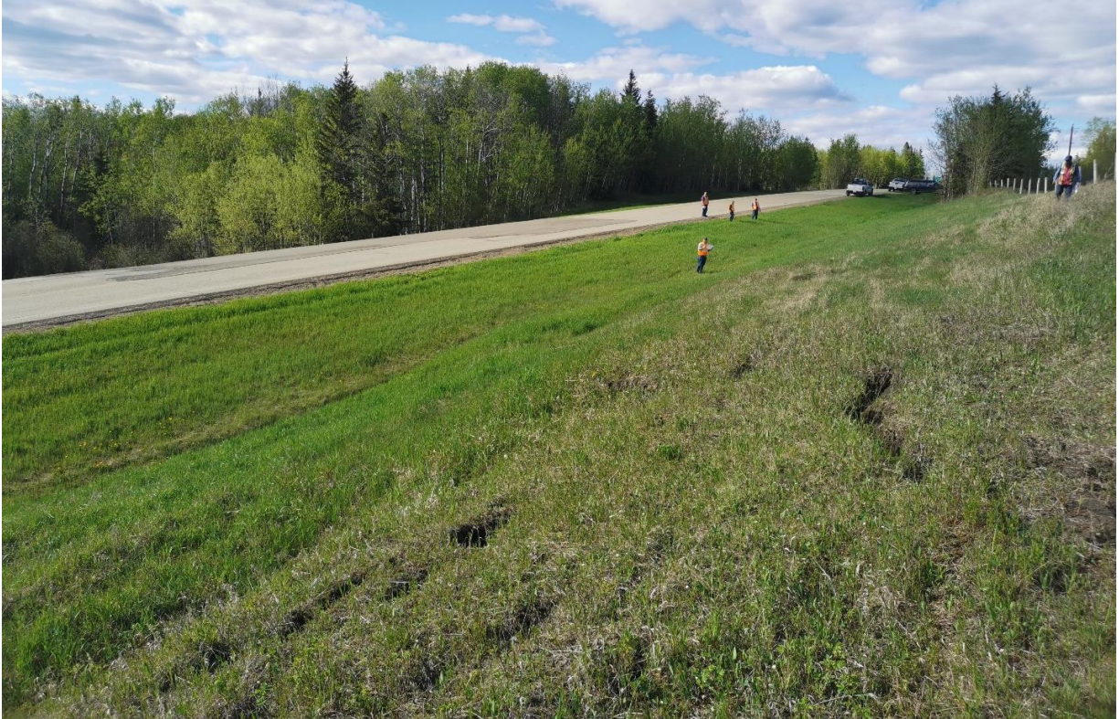
Photo 9 – Looking northwest from the backslope at the subsiding area in the pavement.
