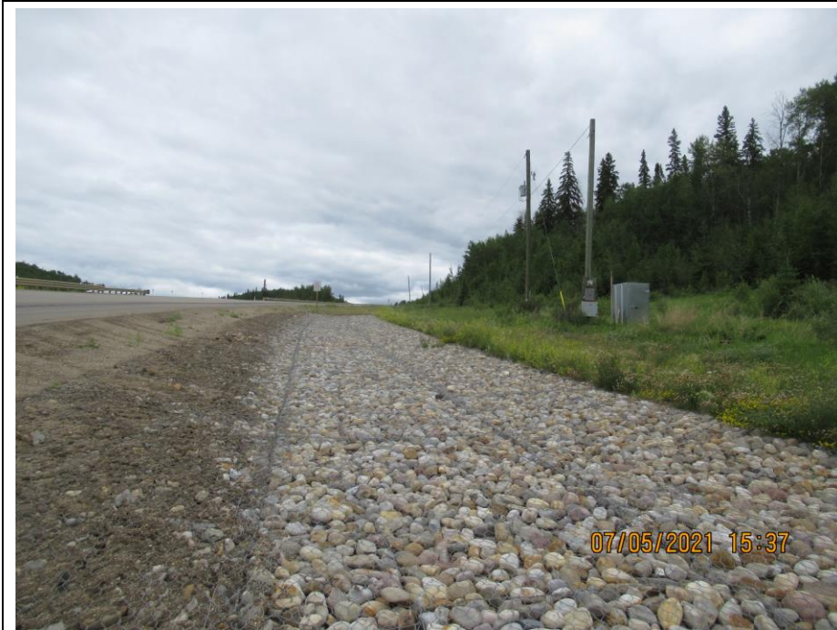
Photo 42-05. View looking east at the gabion mattress installed in the south ditch across the entire site extents to repair previous erosion damage. Minor rill erosion was noted between the road edge and edge of the gabion. No major change within the area east of 33+175 since 2020.
