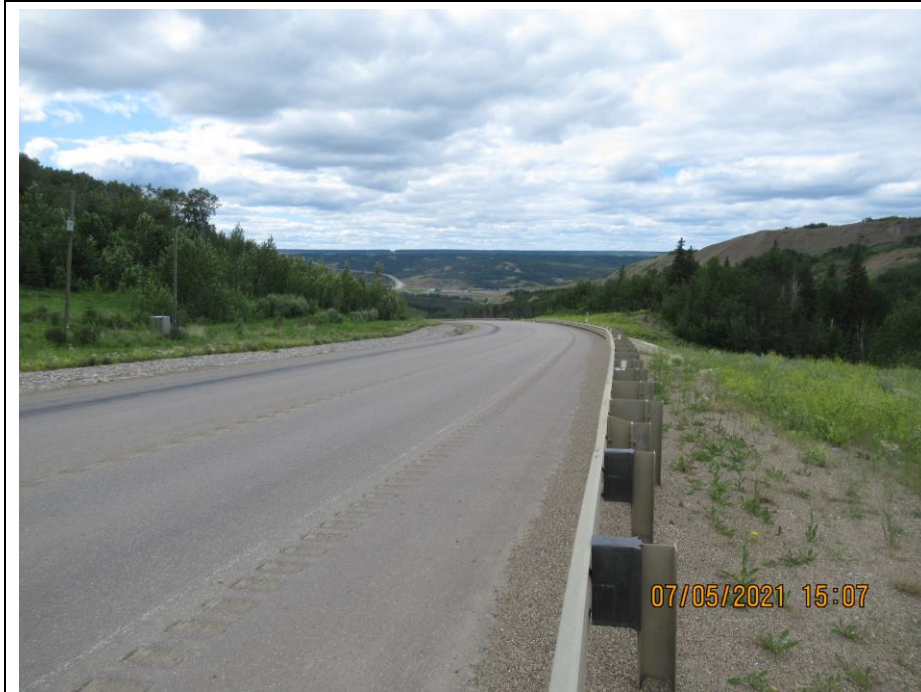
Photo 42-01. Looking west across the repaired slide area. Guardrail and pavement surface in good condition with no major change since previous inspection.
