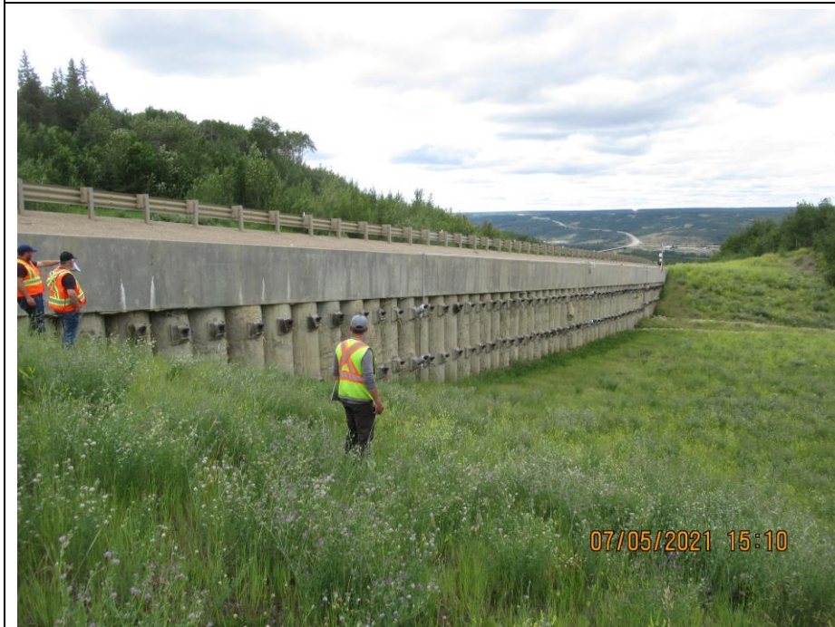
Photo 42-02. Looking west at the new pile wall and regraded slope below. No significant change since 2020.
