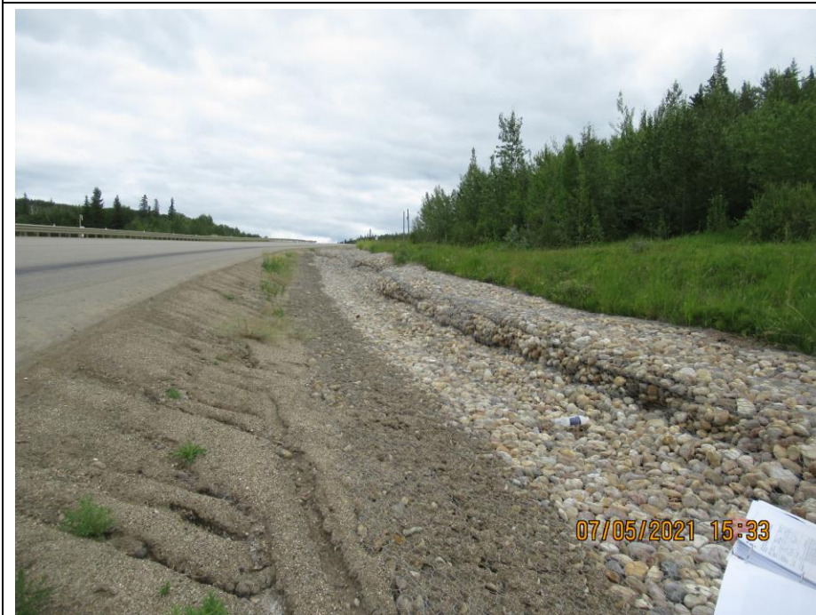
Photo 42-06. View looking east at the gabion mattress installed in the south ditch near 33+125. The toe roll of a landslide that occurred in 2020 has encompassed and deformed the gabion pushing it upwards and towards the highway. The length of gabion affected is approximately 85 m.
