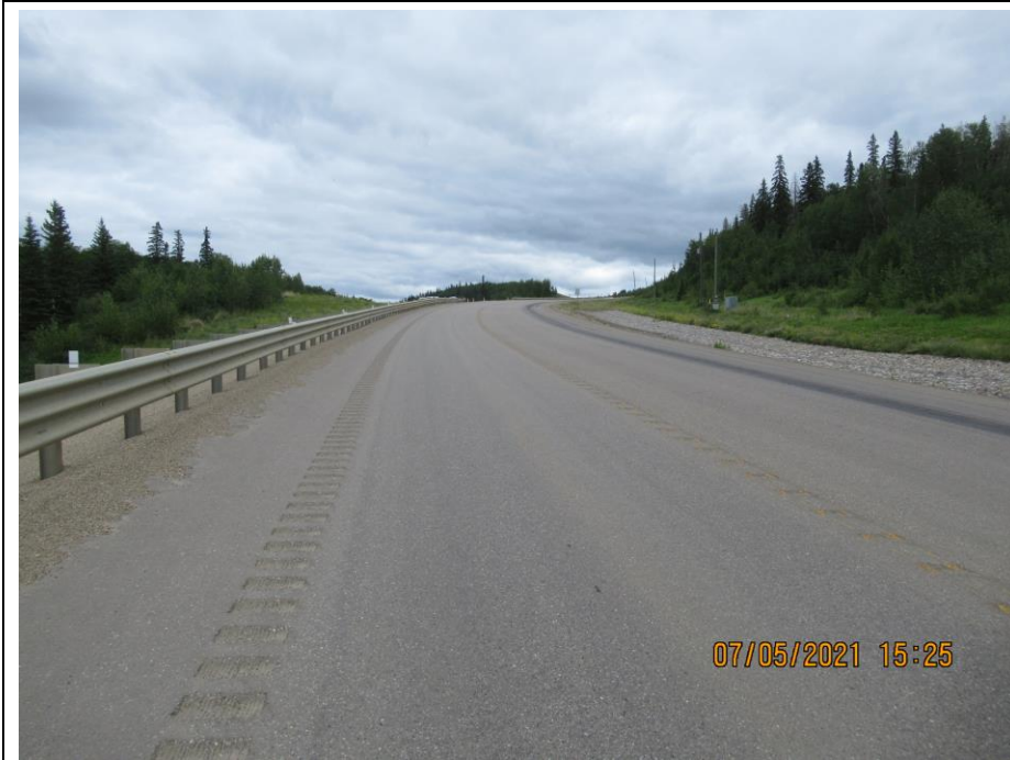
Photo 42-03. Looking east at the replaced highway segment that previously had cracking and settlement across the roadway due to landslide movement (33+210). Road surface was in good condition at time of inspection.
