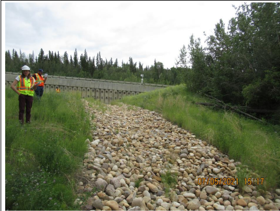
Photo 42-04. Looking south, upslope at one of two drainage swale branches at the west side of the wall.
