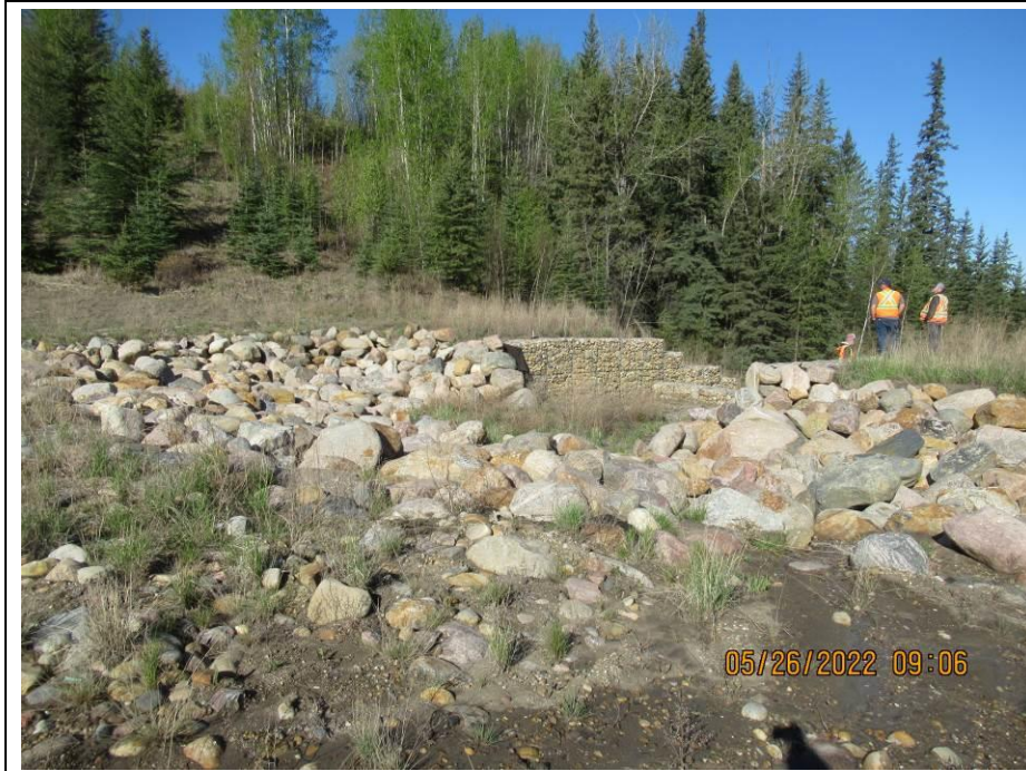
Photo 43-18. View of the riprap berm located near the top of the gabion drop structure (33+650)
