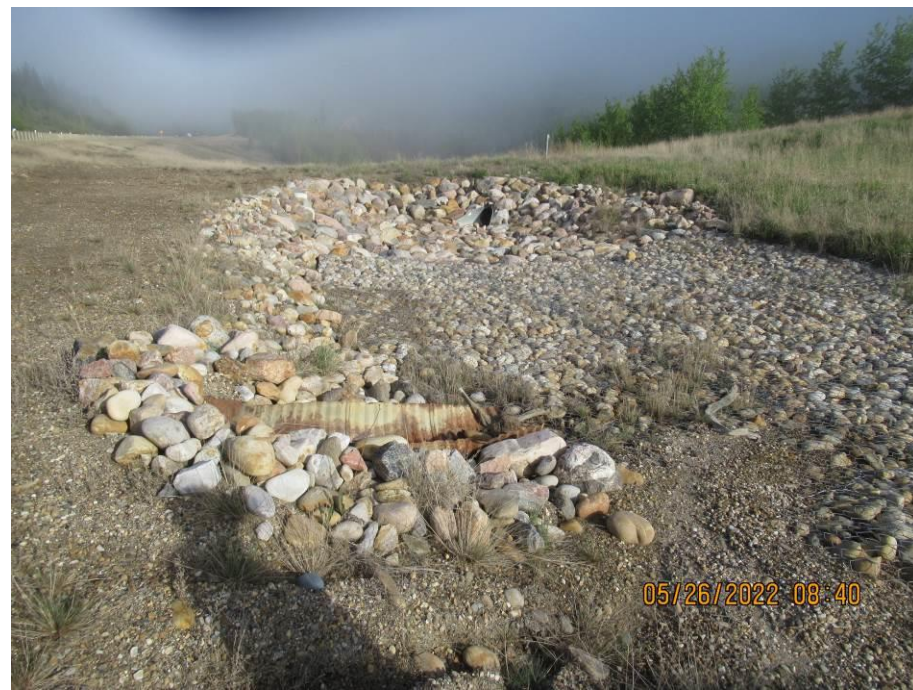
Photo 43-11. View of culvert inlet and riprap protection near 33+900 on north side of road.
