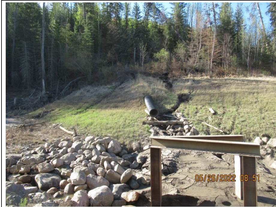
Photo 43-16. Looking south towards the outlet of the CPP down pipe near the culvert inlet (33+800). Rill erosion was noted to be occurring upslope from the pipe outlet due to a leaking joint that requires repair. Increased gully erosion was noted on the right side of the pipe.
