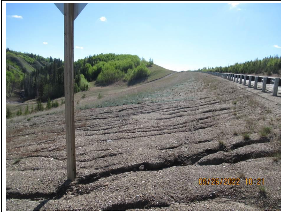
Photo 43-19. View of the minor rill erosion near the top of the embankment of Site B (33+650) where TRM is not installed.
