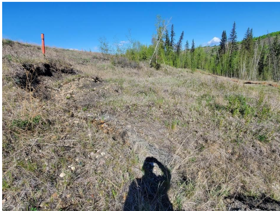
Photo 43-02. Main slide scarp of active shallow failure downslope of the buried pile wall (33+325) first observed in 2017. Area is vegetated and has shown only minor retrogression and expansion since the previous inspection.
