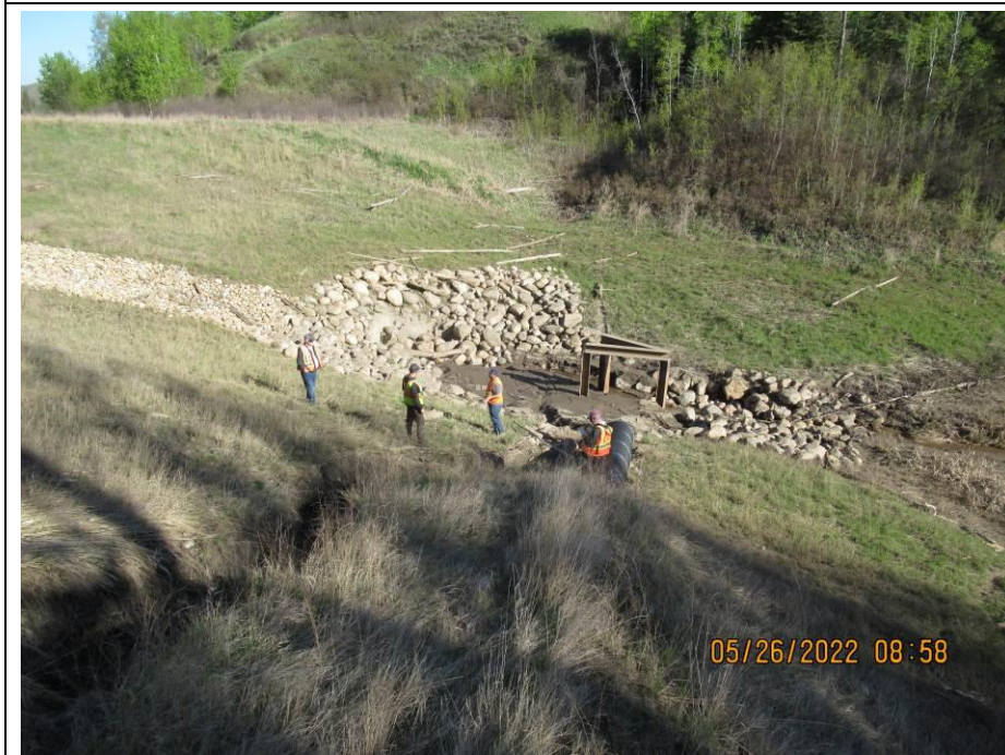
Photo 43-14. Site B culvert inlet with riprap protection and steel H-beam debris deflector. Inlet become severely damaged and blocked with fallen riprap during a high flow event in 2019/2020 (33+800). No major changes from 2021 condition. Increased erosion at gully on left side of photo. Repairs required in this area.
