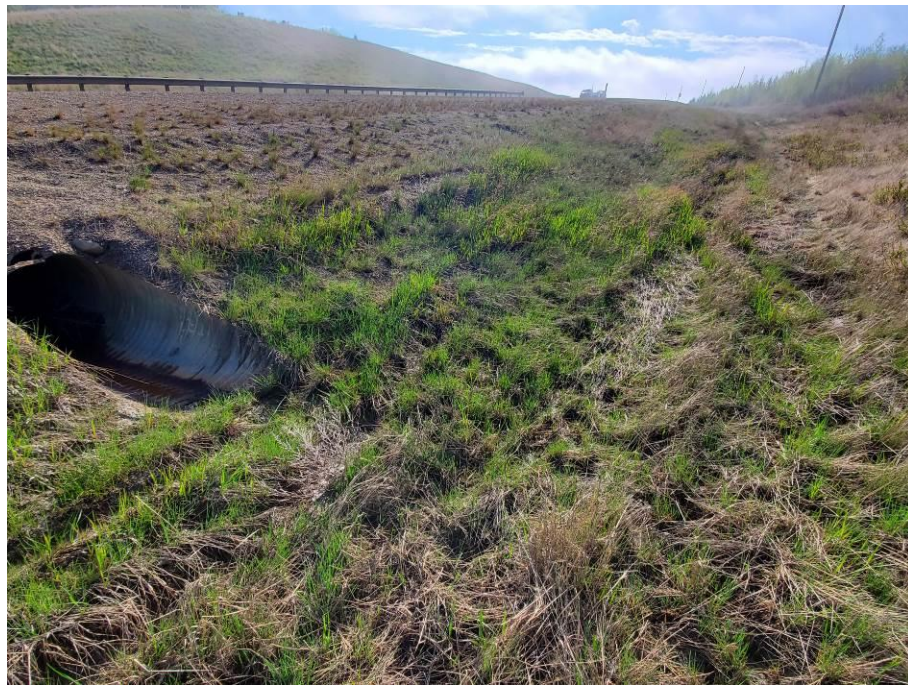
Photo 43-09. South ditch TRM installation at Site B to repair erosion damage and mitigate against future erosion (34+125). Ditch has well established vegetation.
