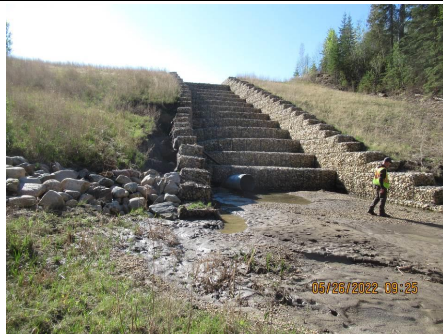
Photo 43-08. View of the gabion drop structure and riprap dissipation bowl at the culvert outlet at Site B. (33+600). Additional erosion and gabion deformation due to piping erosion from leak in the culvert joint (left side).
