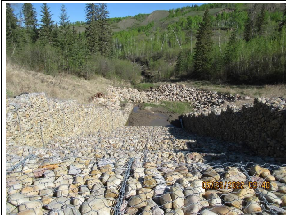
Photo 43-03. Overflow gabion drop structure and dissipation bowl at the previous culvert outlet that had extensive erosion and gullyng below Site A (33+430). Some rill erosion was noted within the fill areas that were still vegetating. Base of drop structure had a large amount of silt buildup. Minor change from 2021 condition.
