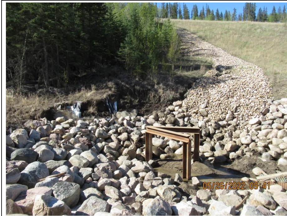
Photo 43-06. Looking south towards the culvert inlet riprap, riprap swale, and debris deflector (33+500). Note south channel bank erosion, silt buildup and erosion within the riprap swale. Slightly worse from the 2021 condition.
