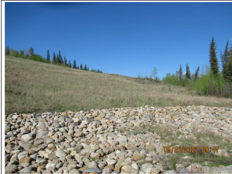
Photo 43-04. Looking southwest at the area of previous slumping associated with culvert erosion below pile wall (33+430). Area has since been graded and finished with straw matting.
