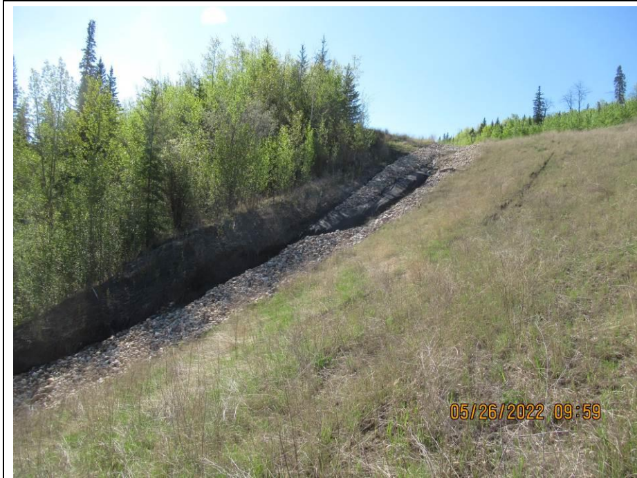
Photo 43-13. Looking south, upslope towards washed out riprap and extensive erosion damage within the riprap swale at the east side of Site A (33+500), likely the result of a high-flow event in 2019/2020. Increased erosion damage since 2021.
