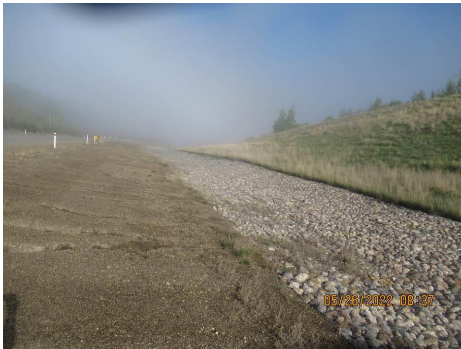
Photo 43-10. Looking west towards the north ditch gabion mattress installation at Site B.
