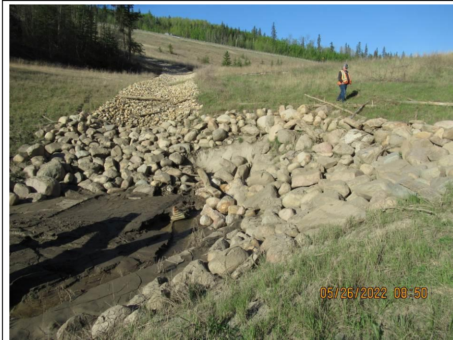
Photo 43-15. Damage around culvert inlet due to a high flow event. Culvert pipe at the inlet was effectively pinched and twisted shut and was filled with woody debris. Riprap above the inlet had collapsed and slid down over it. No change to riprap damage or woody debris buildup. Increased silt buildup relative to 2021 condition. Repairs required in this area (33+800).
