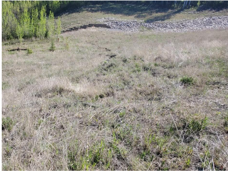
Photo 43-01. At the west edge of Site A near top of the buried pile wall looking northeast towards the overflow area and gabion drop structure. No major change from 2021.
