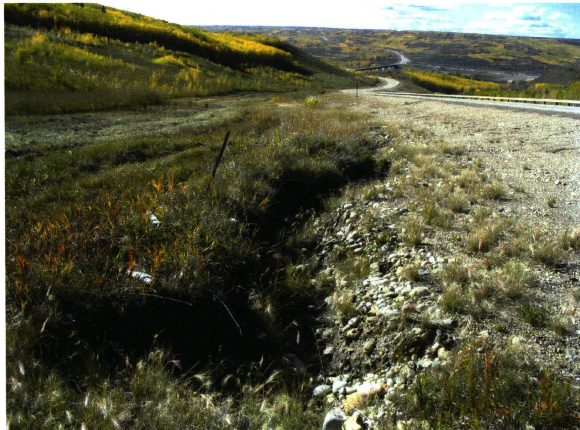
PHOTO 8 LOOKING DOWNSTREAM FROM EAST END OF ERODED DITCH AT ABOUT STA. 12+920
