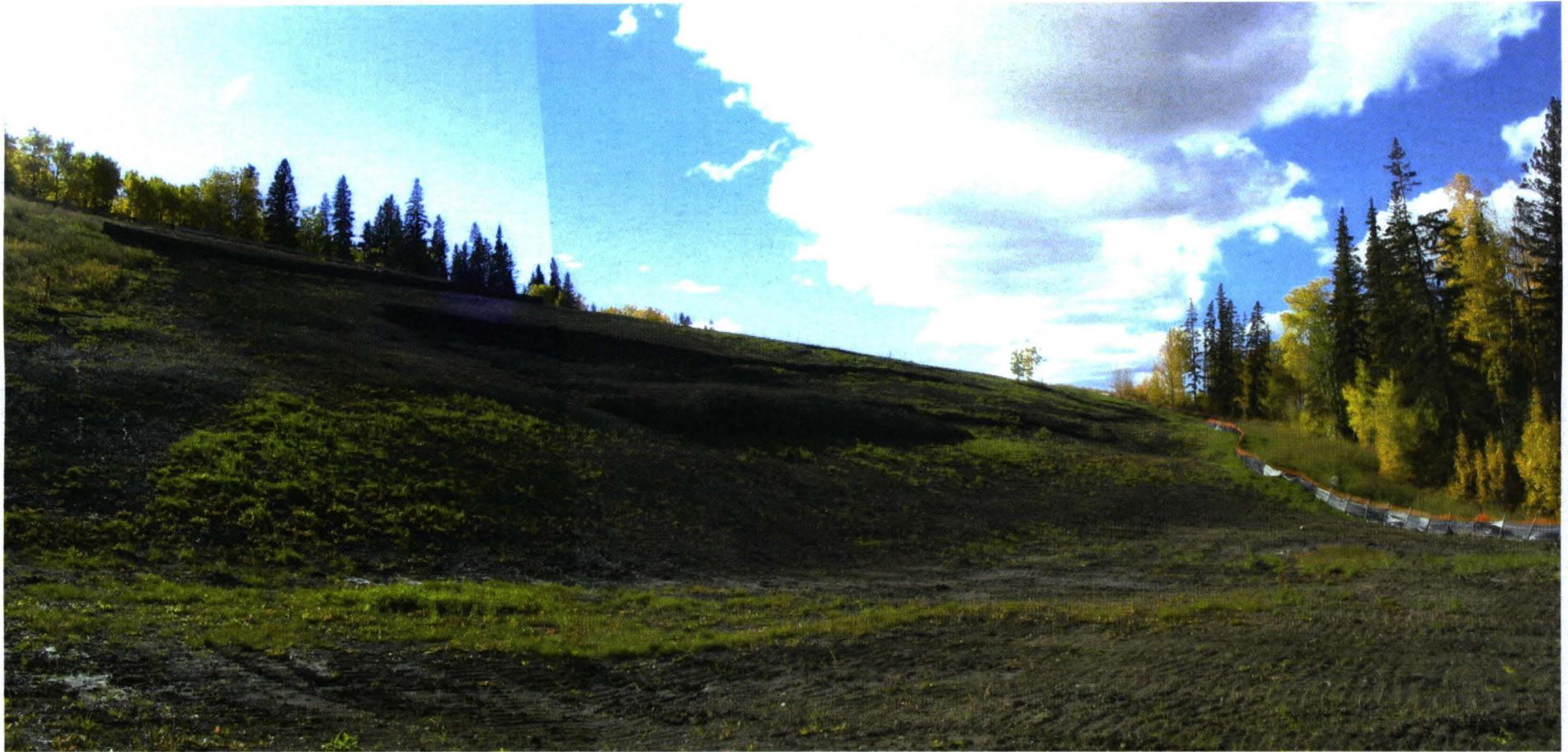
PHOTO 9 LOOKING WEST AT SLIDE IN SLOPE BELOW PILE WALL
