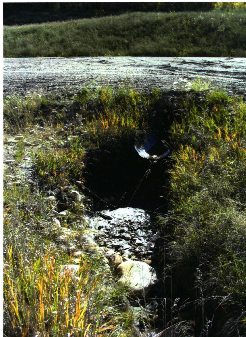
PHOTO 4 SCOUR BELOW OUTLET OF CULVERT
