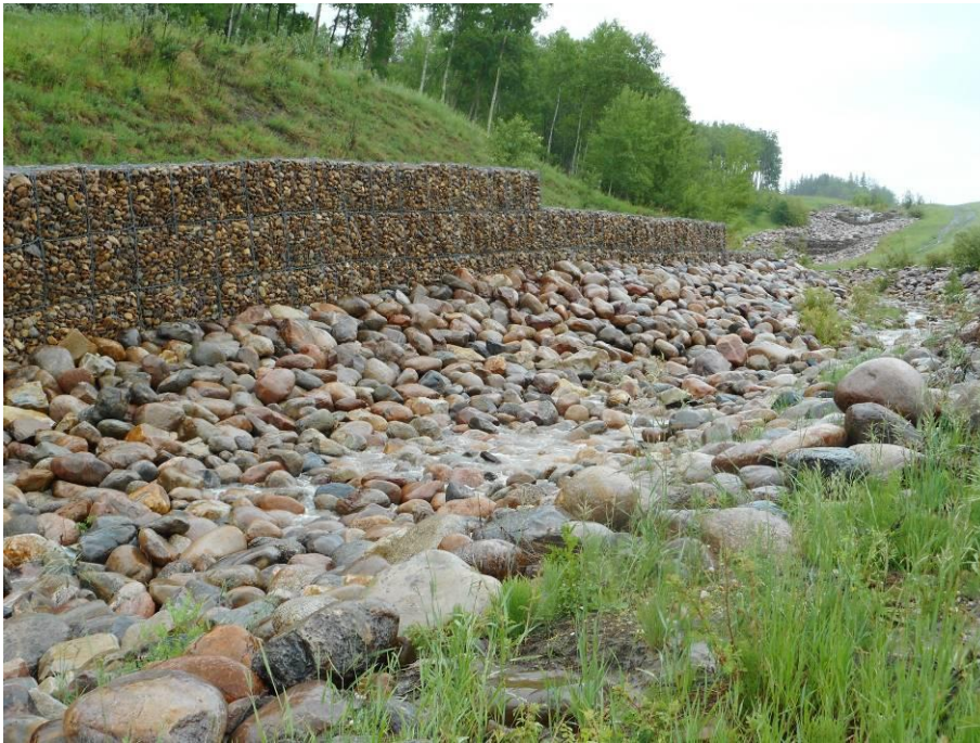
Photo 7-01. Looking at protective gabion wall along north side of channel near end of armoring. Previous area of channel erosion and armour breach has since been repaired (32+290).
