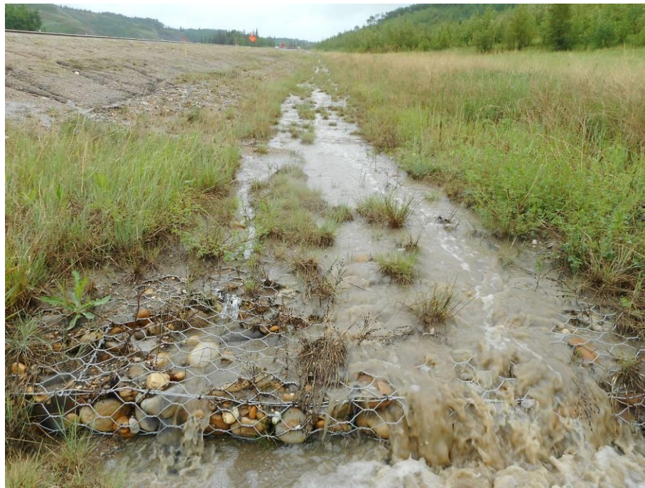
Photo 7-13. Looking upslope the ditch (east) at the 300 mm thick gabion mattress erosion control section (32+450). Section had vegetation growth and was performing well.
