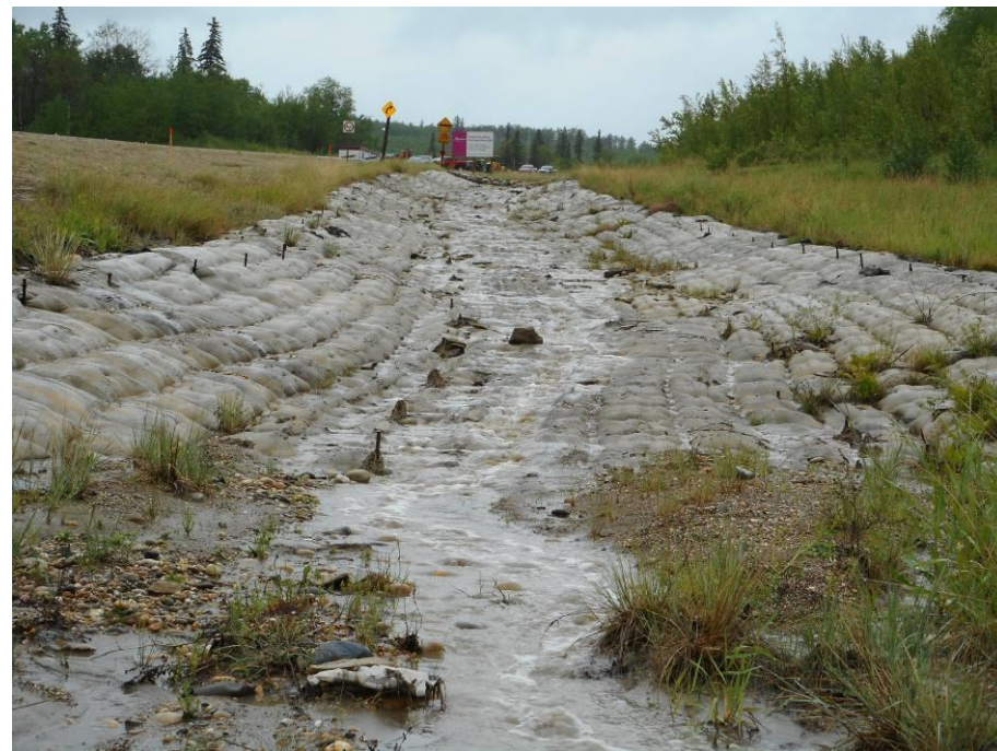
Photo 7-10. Looking upslope the ditch (east) at the pillow concrete erosion control section (32+825). Note rebar protruding.
