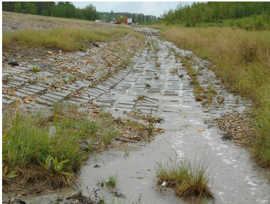
Photo 7-11. Looking up the ditch slope (east) at the cabled concrete erosion control section (32+700). Nearly all exposed cable loops in this segment have been cut.
