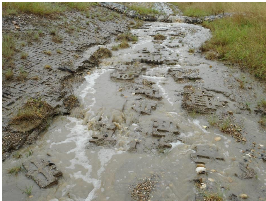
Photo 7-12. Looking upslope (east) at weathered and broken interlocked concrete blocks (100 mm thick Lafarge paving stones) (32+660).
