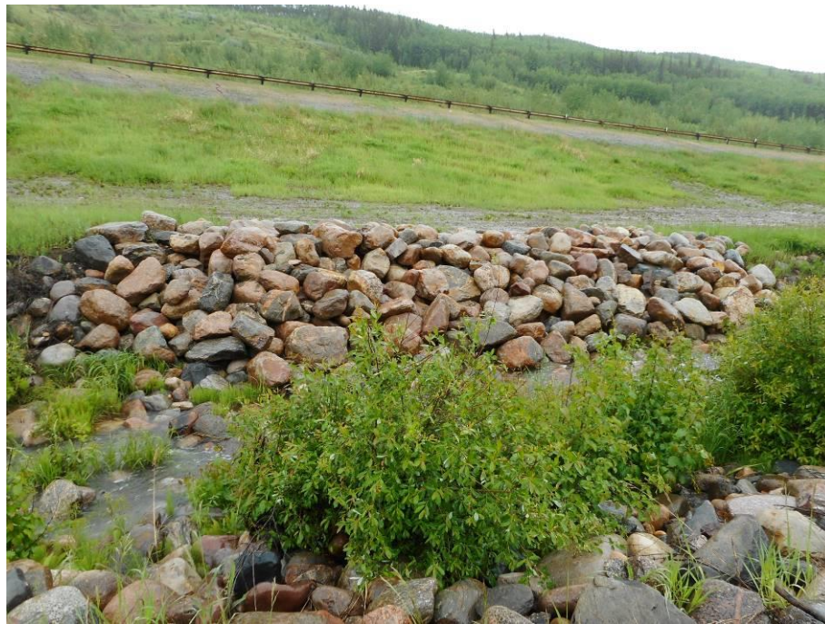
Photo 7-05. Previous area of bank erosion and breach of armour on south side, recently repaired with placement of additional rip rap (32+660).
