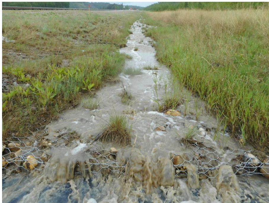
Photo 7-14. Looking upslope the ditch (east) at the geocell filled with gravel (32+350). Section had vegetation growth and was performing well.
