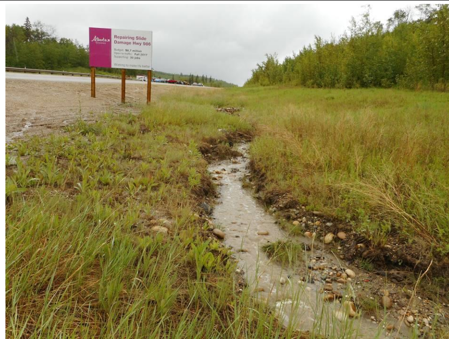
Photo 7-9. Looking up the ditch slope (east) at end of erosion control section (32+900).
