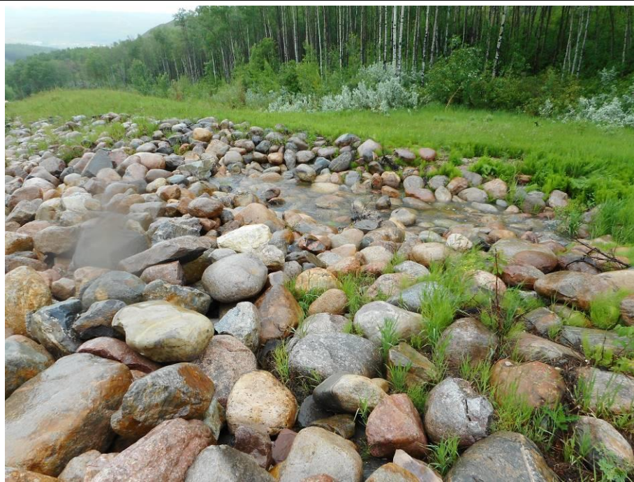
Photo 7-03. Previous area of geotextile exposure and bank erosion at north side gabion drop structure that has been filled in with additional rip rap (32+500).
