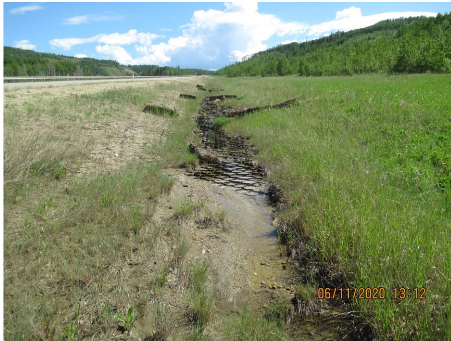
Photo 7-12. Looking upslope the ditch (east) at the geoweb control section (32+400). Section had vegetation growth and was performing well. Some minor rill damage was noted on the north side of the ditch.
