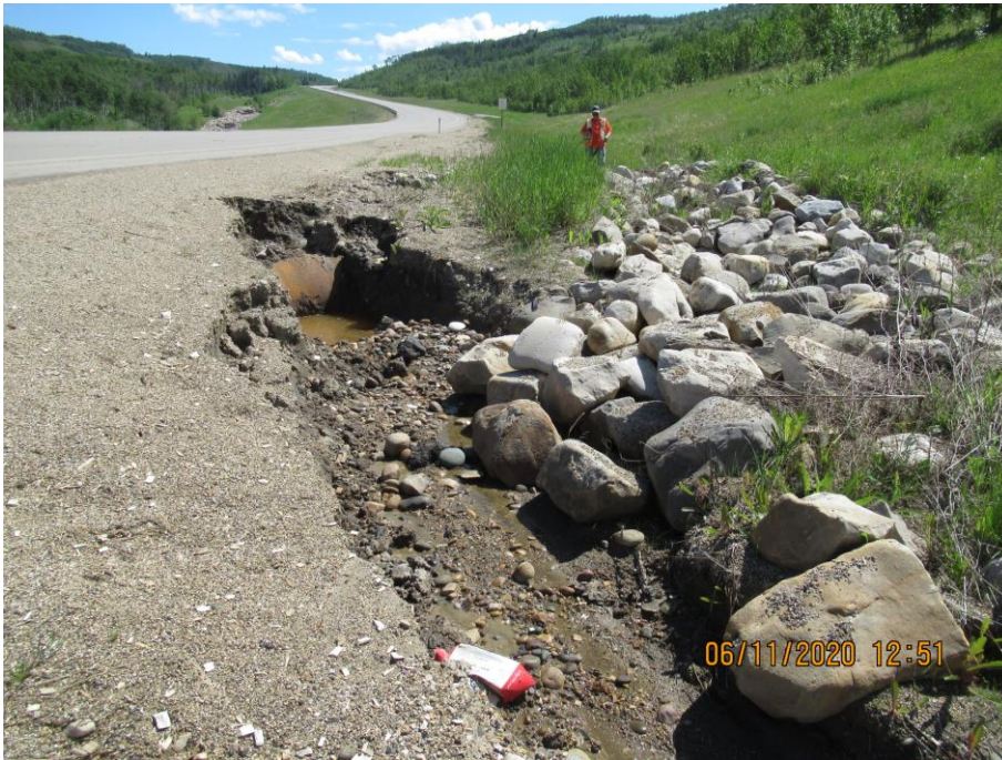
Photo 7-8. New erosion / washout around the culvert intake structure at the west end of the erosion control test ditch (32+050).
