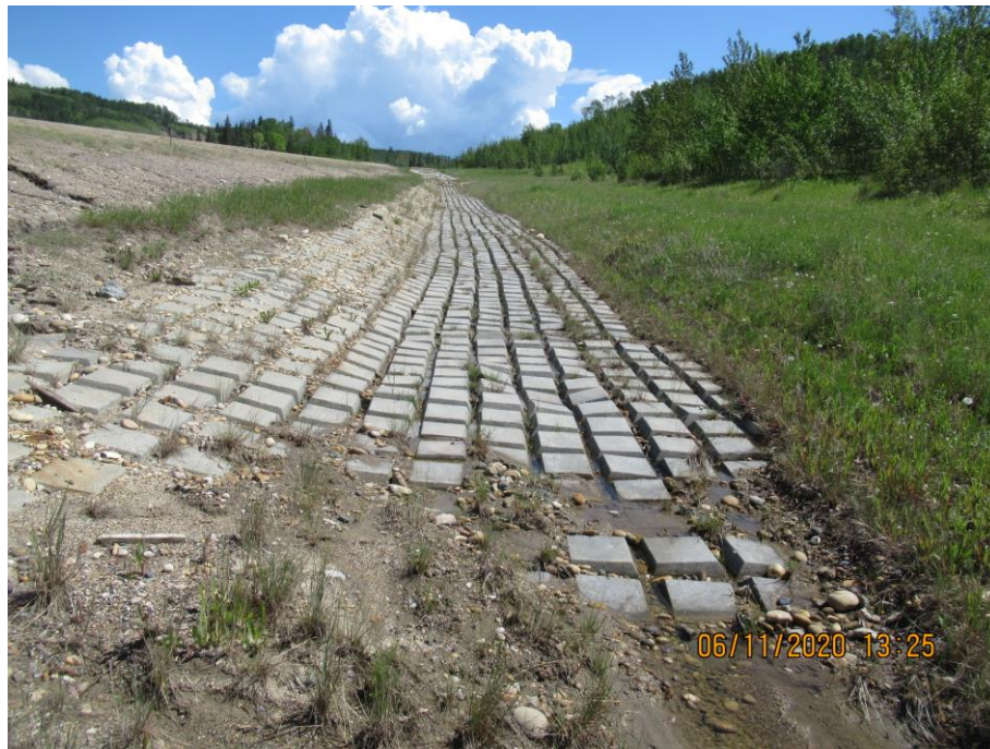
Photo 7-15. Looking east towards cabled concrete section (32+700). Section was performing well. Minor erosion damage was noted on the north side of the ditch
