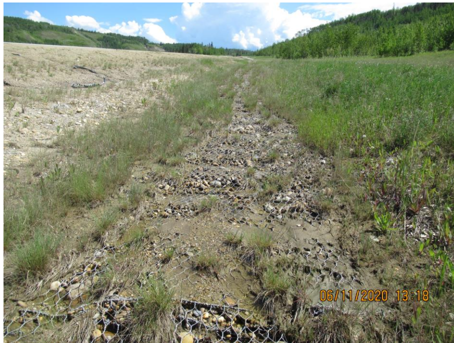
Photo 7-13. Looking upslope the ditch (east) at the gabion mattress section (32+500). Section had vegetation growth and was performing well.
