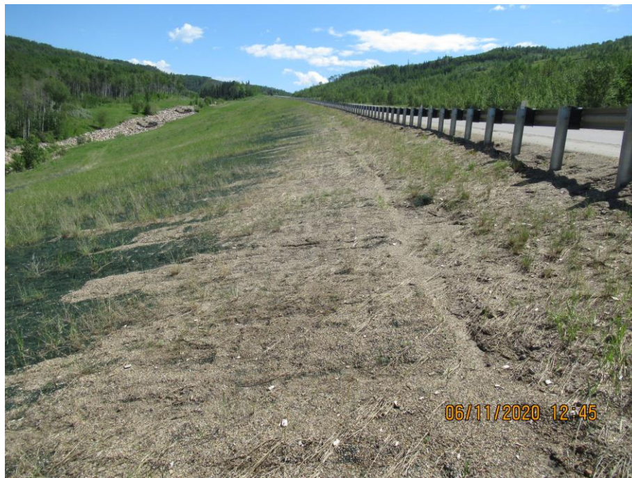
Photo 7-02. Looking east towards area with previous rill erosion that was repaired in 2018 with backfill and TRM (32+300). Overall area was in good condition.
