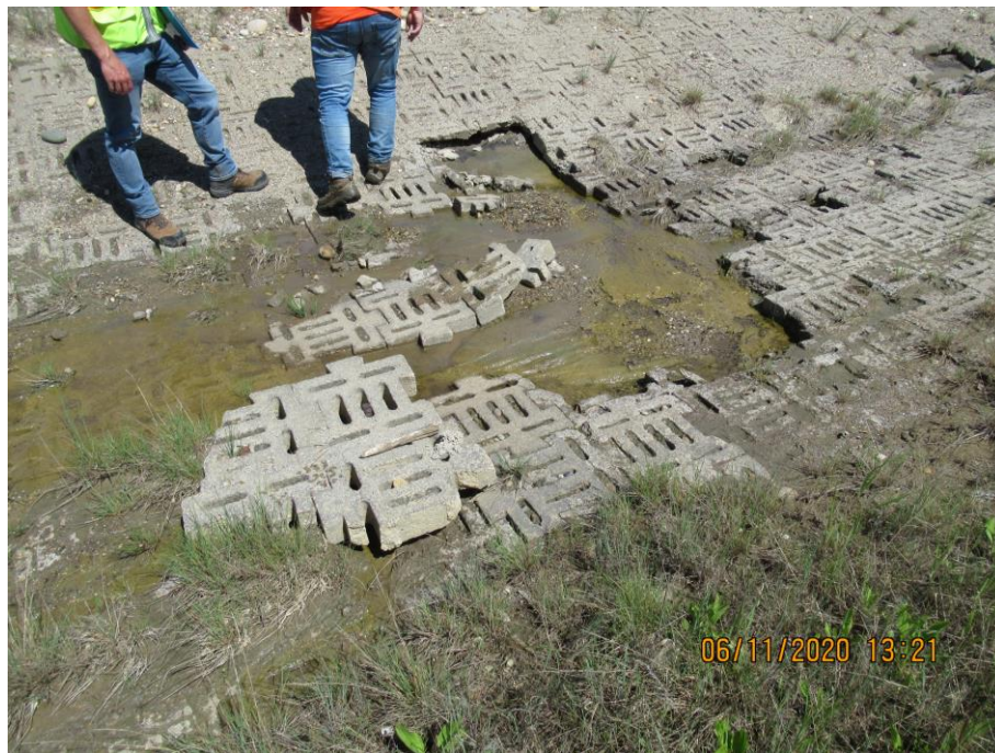
Photo 7-14. View of the damage within the interlocked concrete block (i.e. Lafarge paving stones) paving stone section (32+600). Blocks have deteriorated and broken up in numerous locations and have been undermined by erosion exposing geotextile fabric beneath. Overall section is performing poorly.
