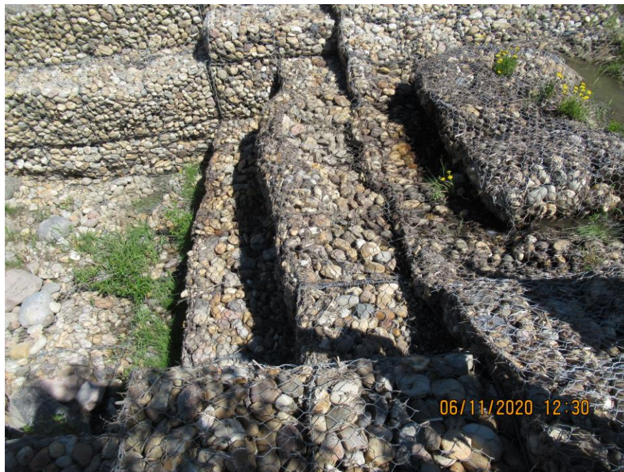
Photo 7-04. Close-up view of the internal upper gabion drop structure (32+540). Baskets in the channel centre have some bagging and broken wire. Maintenance recommended to prevent further damage / loss of gabion rock. Otherwise structure is intact and functioning as intended.
