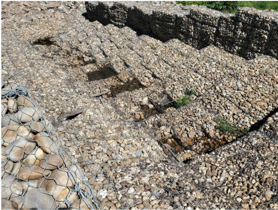
Photo 7-07. View of the lower segment of the gabion channel bend and drop structure (31+800). Gabions within the middle of the channel showing some bagging and wire damage that will require eventual maintenance to prevent further basket damage. Overall structure was intact and functioning as intended.
