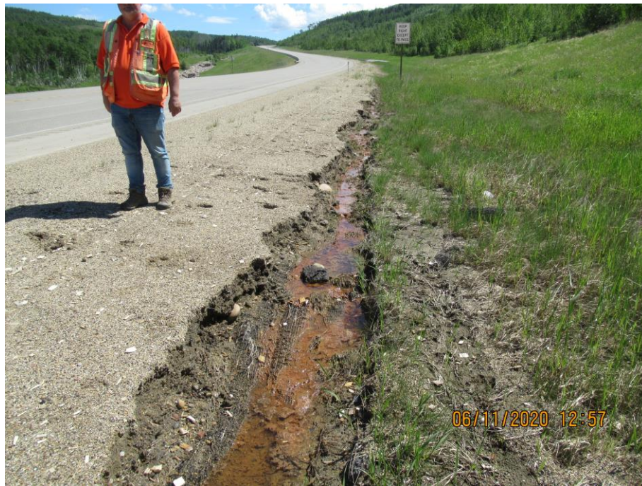
Photo 7-9. New channelized erosion through vegetated sediment buildup on the north side of the ditch within the rolled erosion control product (turf reinforced matting) test section (32+100).
