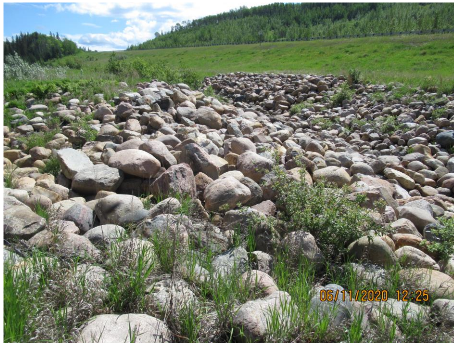
Photo 7-05. Previous areas of bank erosion and breach of armour on south side, repaired with placement of additional rip rap which was still intact (32+650).
