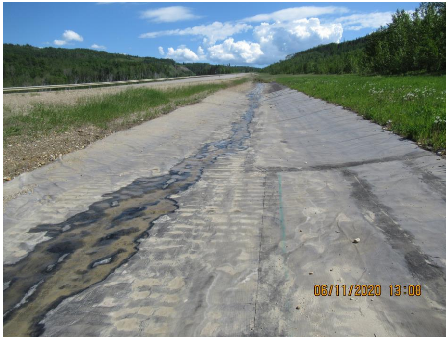
Photo 7-11. Looking upslope (east) at the Coletanche geomembrane erosion control section (32+250). Membrane was recently patched, the erosion underneath was backfilled and overall appeared to be performing well.
