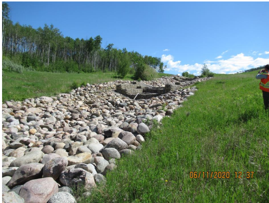
Photo 7-03. Looking east, upslope from below two gabion drop structures. Overall the armoured channel was in good condition and recently repaired areas of rip-rap replacement/bank erosion were intact (32+450).
