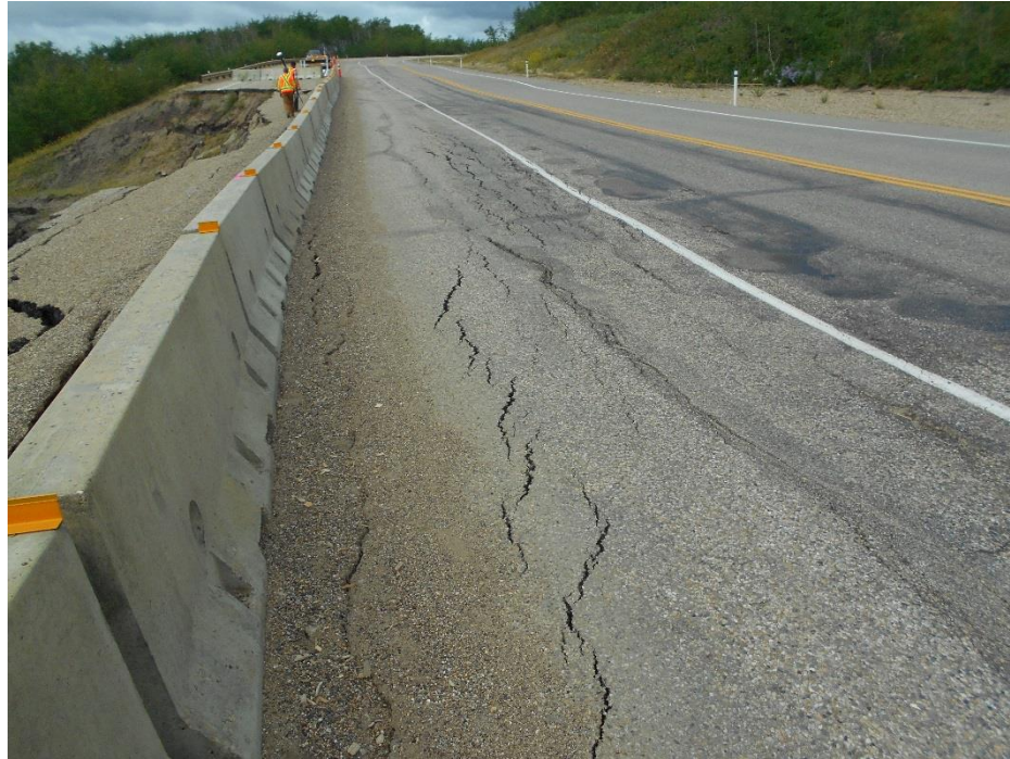
Photo 71-03. Tension cracks developing just behind the jersey barrier.
