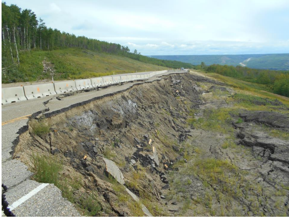
Photo 71-01. Looking east at current back scarp along the highway south shoulder. The backscarp is about 6.0 to 6.5 m in height.
