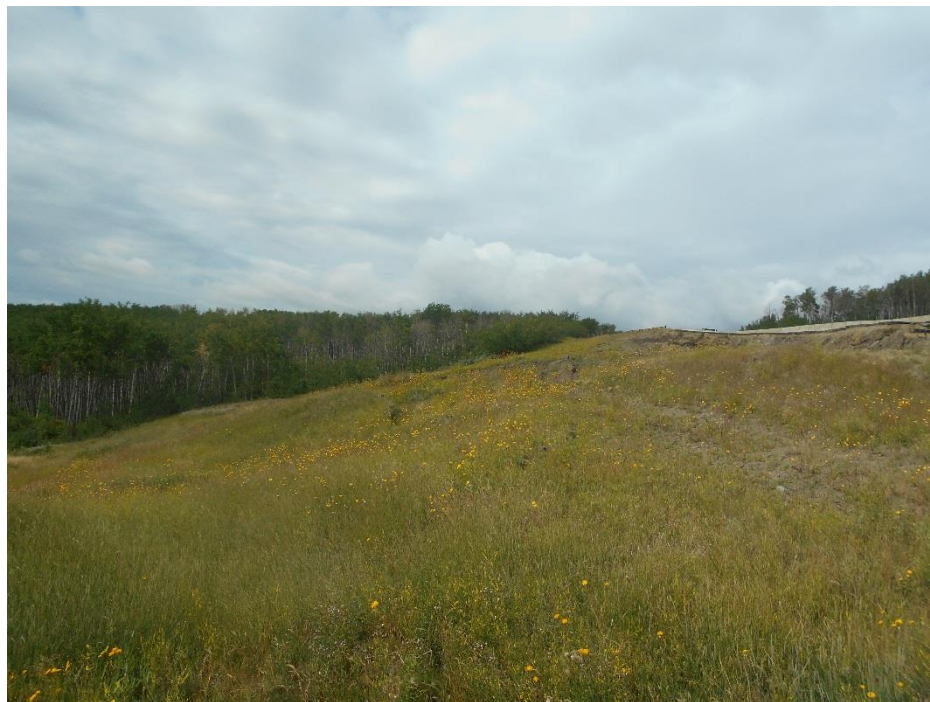
Photo 71-04. Landslide looking west. Slight bulging is developing mainly above the culvert outlet.
