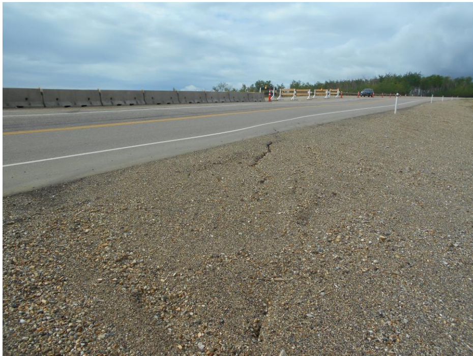
Photo 71-02. Tension crack developing just behind the highway north shoulder.
