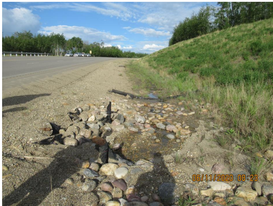
Photo 71-4. View toward the west looking upslope in the north ditch at the culvert inlets (26+650). One of the two culverts has been blocked due to silt buildup.
