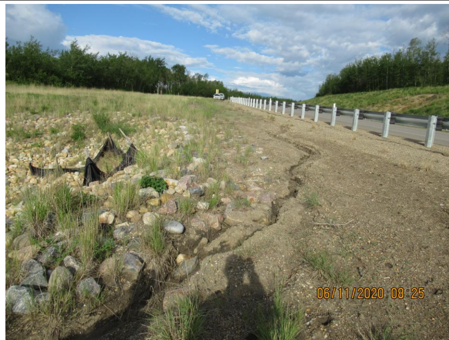
Photo 71-5. West of the wall on the south side of the road (26+650), water runoff from the road currently flows around the armored swale in an erosion rill. Slightly worse from the 2019 condition.
