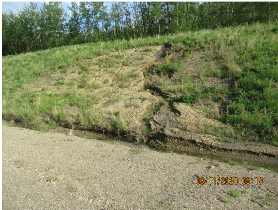
Photo 71-3. Backslope area upslope of the highway above the pile wall near the west end of the site looking towards the northwest (26+550). Granular fill within the backslope has eroded and partially washed out. Increased erosion within backslope and ditch since 2019. Geordige ditch barriers have been outflanked in some sections.
