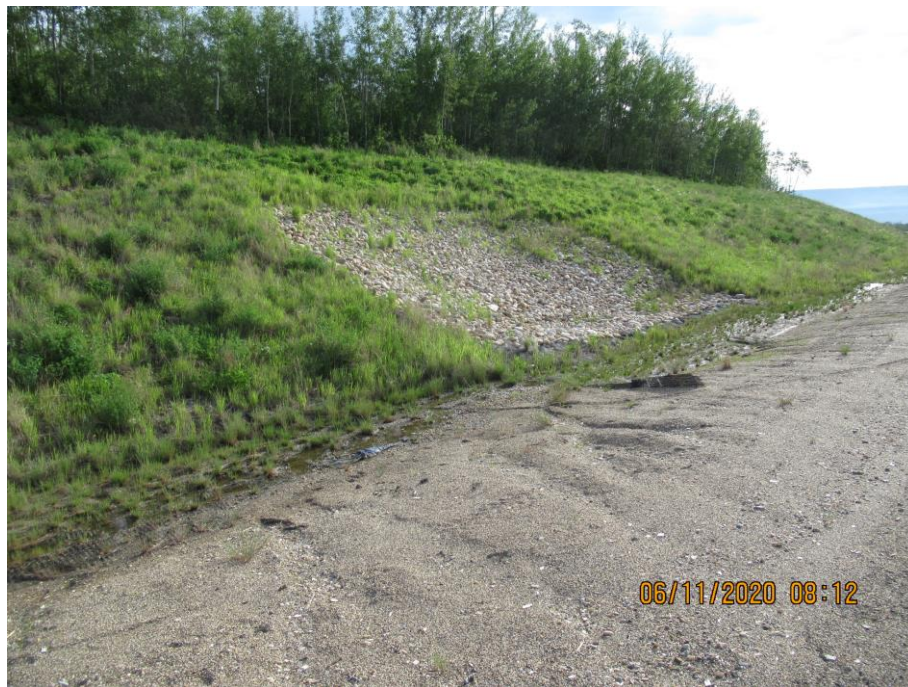
Photo 71-2. Second area of granular backslope repair on north side of road. Minor ditch erosion but overall slope was in good condition (26+500).
