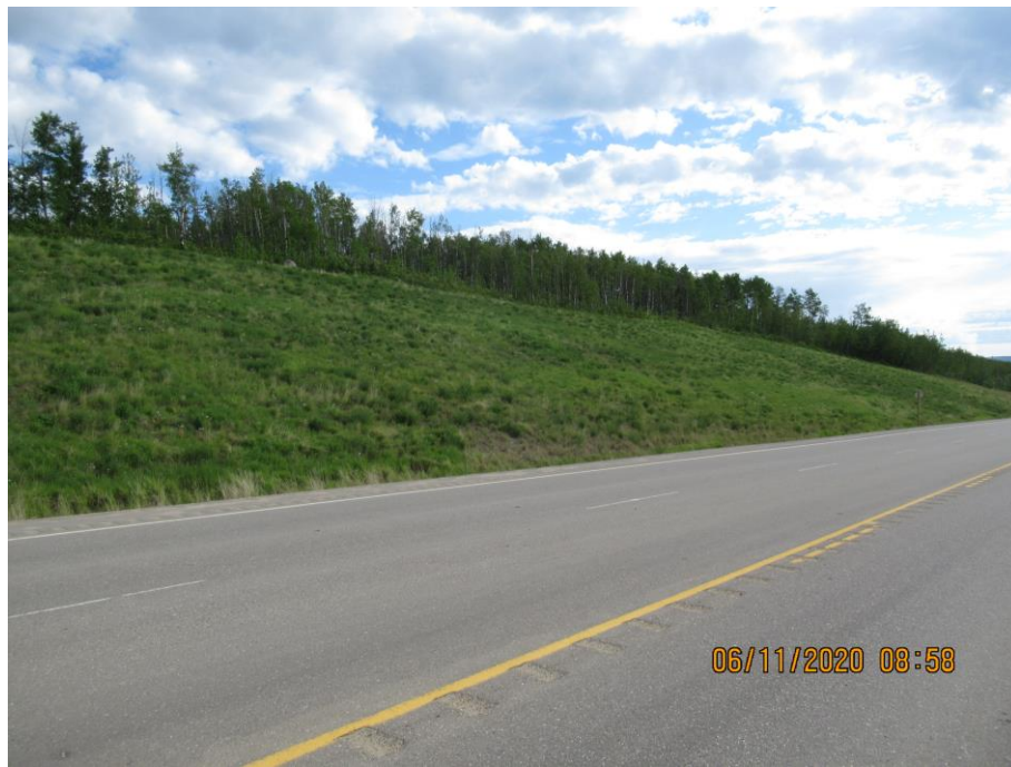
Photo 71-12. Looking northeast towards the backslope area across from the pile wall (26+800). Slope had good vegetation coverage and no issues were observed.
