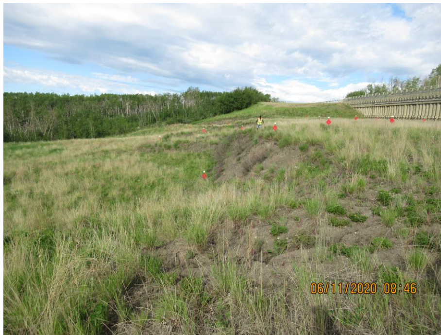
Photo 71-8. Looking towards the west at the downslope area below the wall at the main scarp where landslide movement has continued since the pile wall was constructed. Scarps and cracking has typically followed along previously observed slide extents prior to the regrading and wall construction.
