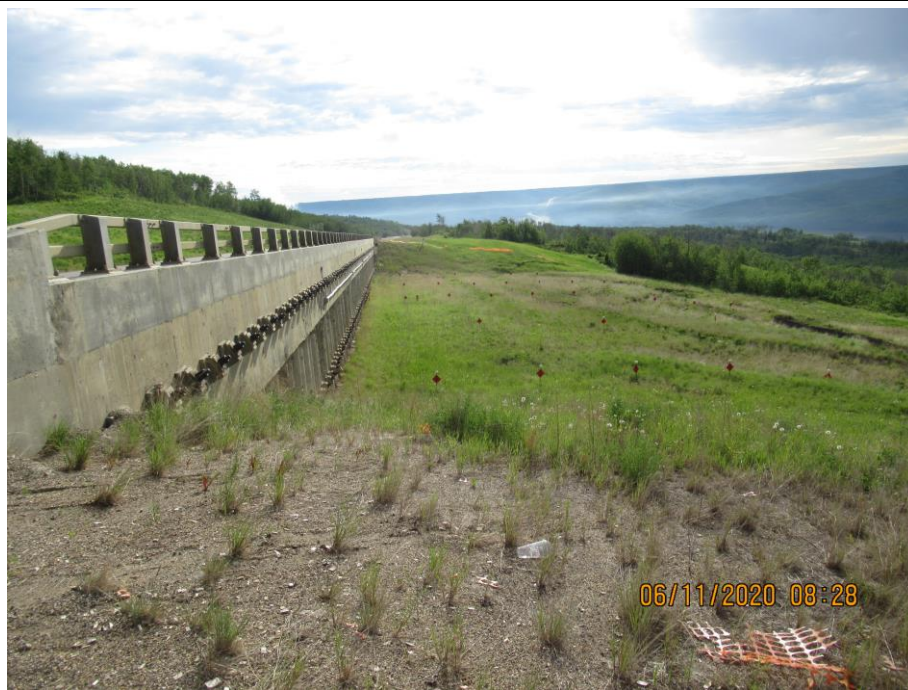
Photo 71-7. At the west end of the pile wall looking towards the east downslope of the wall.
