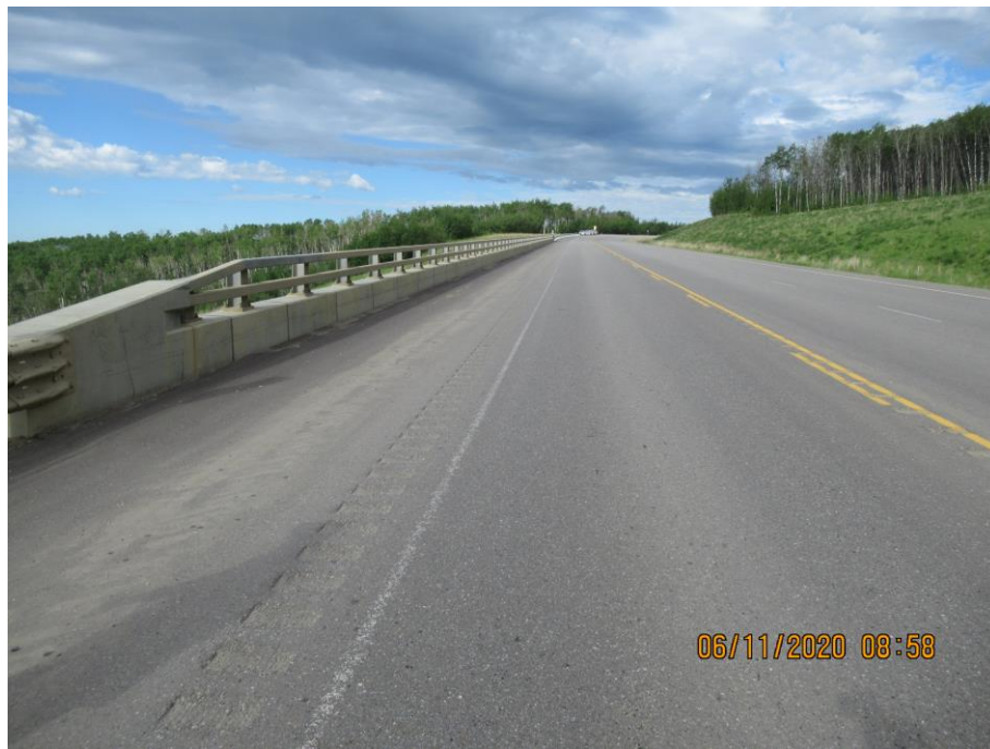
Photo 71-10. Looking west along the highway above the pile wall. Pavement was in good condition. Previous buildup of sand and gravel below the guardrail at the east end of the wall was cleaned/washed out.
