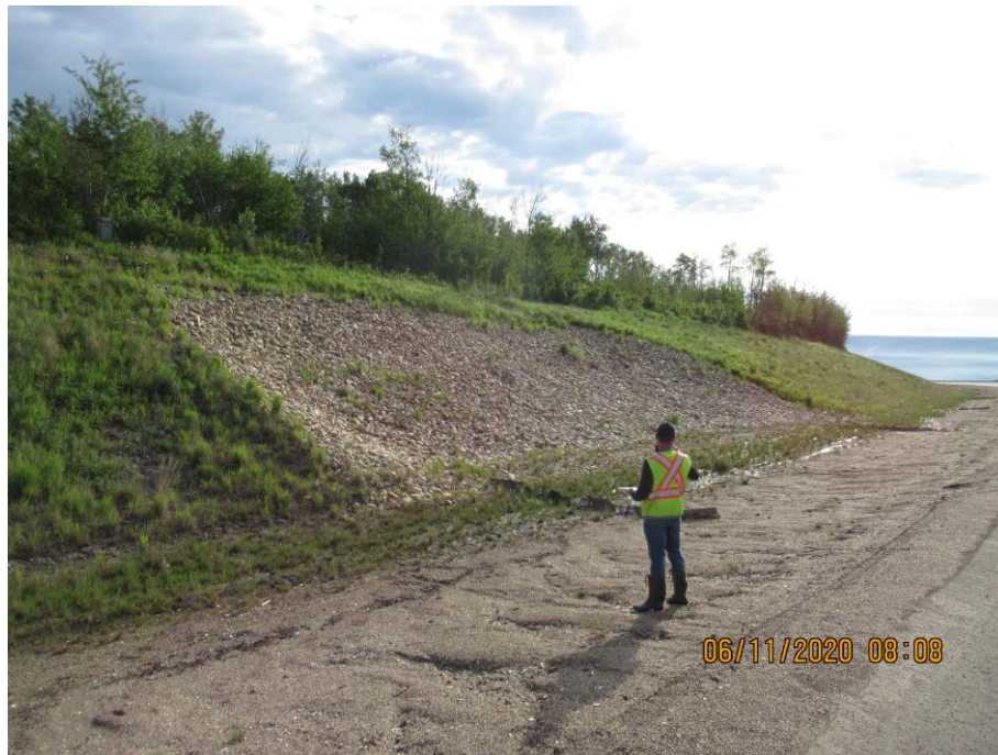
Photo 71-1. Granular backslope repair on north side of road was in good condition (26+350).
