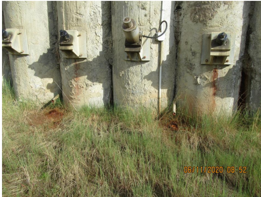
Photo 71-9. Weep holes at the east end of the wall had active seepage and area was wet.
