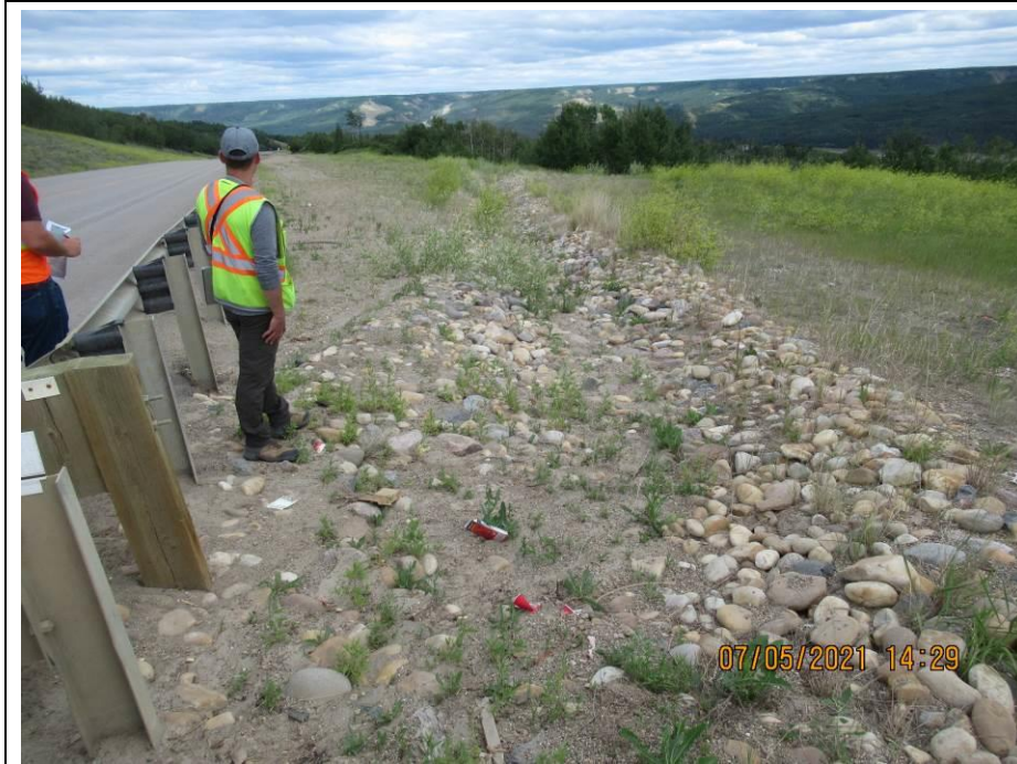
Photo 71-11. Looking towards the east at the east end of the pile wall at the armoured drainage swale. Minor rill erosion was observed between the swale and road edge in areas of poor vegetation. Some increased sediment buildup in the swale but no major change from 2020 condition.
