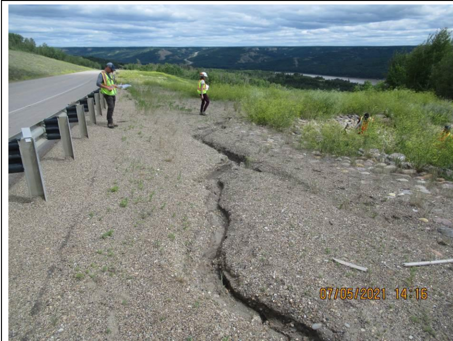
Photo 71-5. West of the wall on the south side of the road (26+650), water runoff from the road currently flows around the armored swale in an erosion rill. No major change from the 2020 condition.
