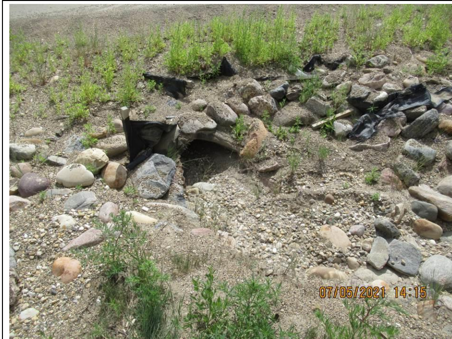
Photo 71-4. View toward the north ditch culvert inlets (26+650). One culvert has been fully blocked due to silt buildup and the other is about \frac{3}{4} full.
