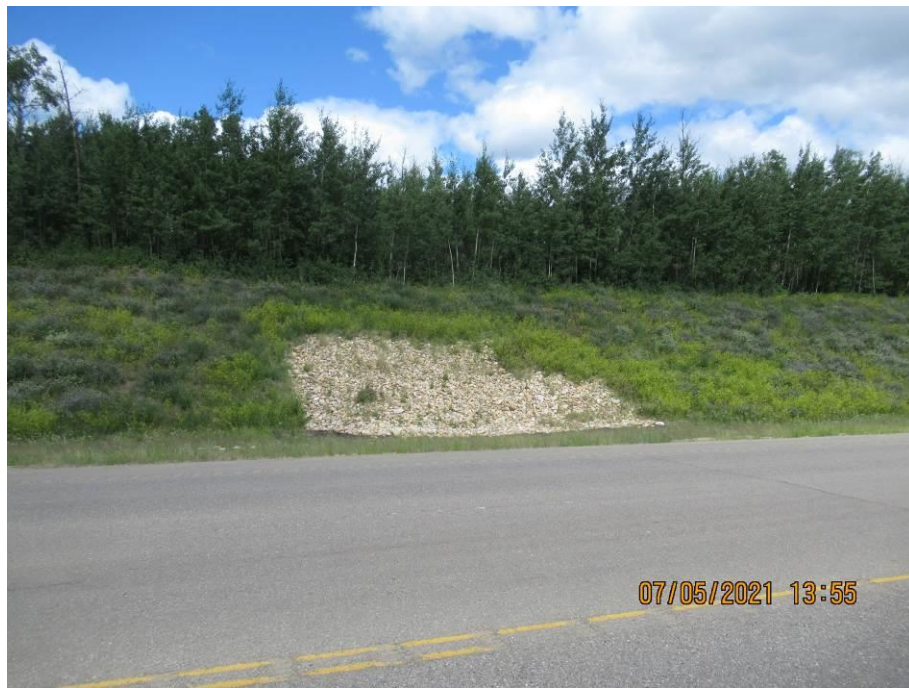
Photo 71-2. Second area of granular backslope repair on north side of road. Overall slope was in good condition and vegetation was filling in (26+500).
