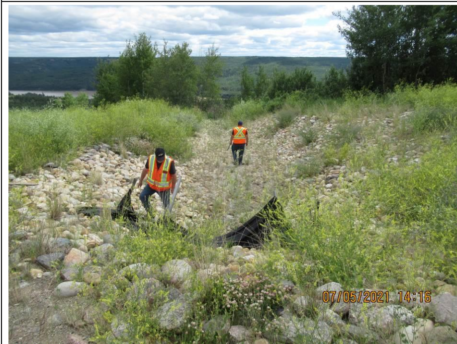
Photo 71-6. View of the armored swale at the culvert outlets (26+650). No issues were noted at the time of inspection.
