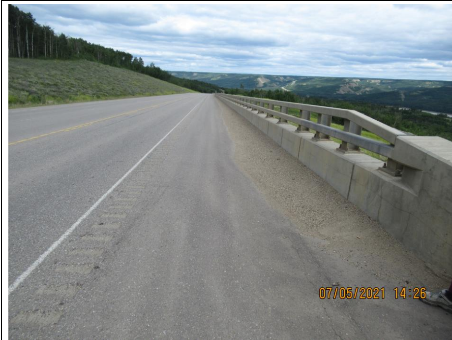
Photo 71-10. Looking east along the highway above the pile wall. Pavement was in good condition. Minor buildup of sand and gravel at the base of the guardrail along the top of the wall.
