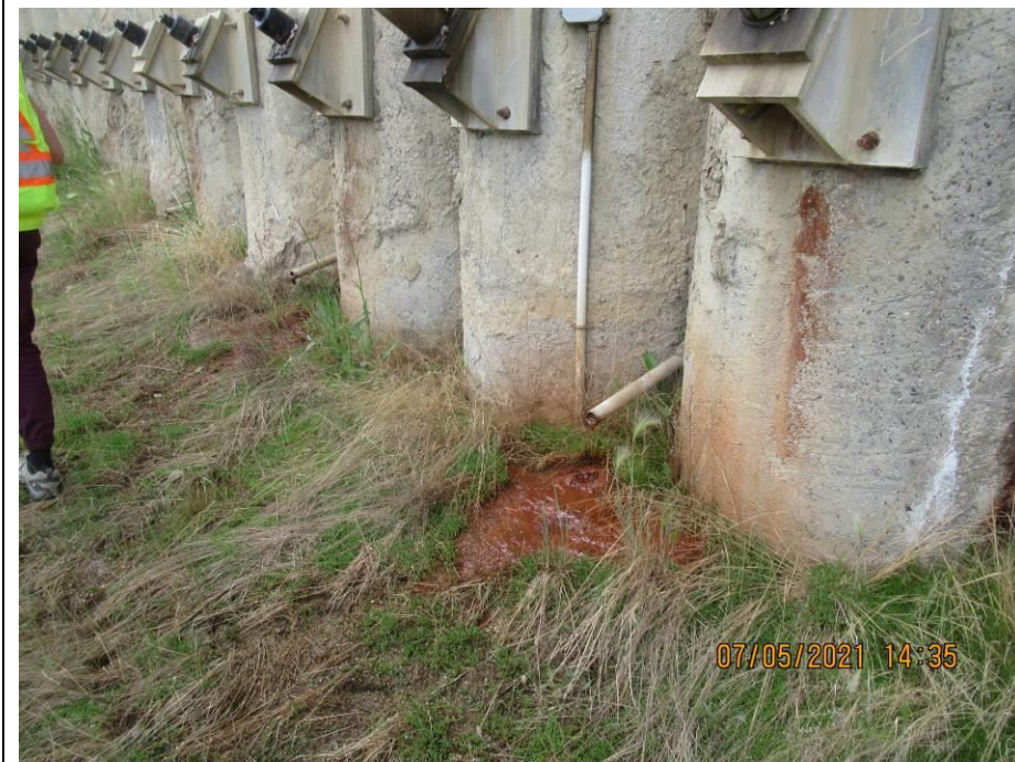
Photo 71-9. Weep holes at the east end of the wall had active seepage and area was wet.
