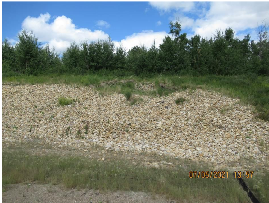
Photo 71-1. A shallow earth slide developed within the swale at the top of the granular backslope repair on north side of road since the previous inspection (26+350). There was a slight toe bulge at the mid-slope under the riprap.
