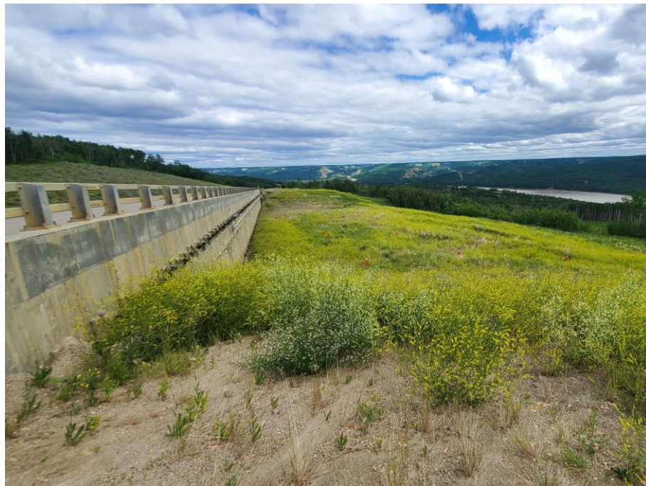
Photo 71-7. At the west end of the pile wall looking towards the east downslope of the wall. Vegetation is well established below the wall.
