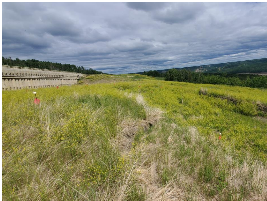
Photo 71-8. Looking towards the east at the downslope area below the wall at the main scarp where landslide movement has continued since the pile wall was constructed. Scarps have typically followed along previously observed slide extents prior to the regrading and wall construction.
