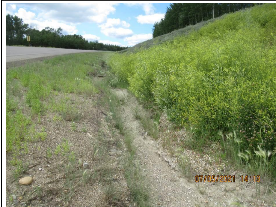
Photo 71-3. Backslope area upslope of the highway above the pile wall near the west end of the site looking towards the northwest (26+550). Granular fill had eroded and partially washed out but has since had increased vegetation growth. Ditch erosion is slightly worse. Georidge ditch barriers have been outflanked in some sections.
