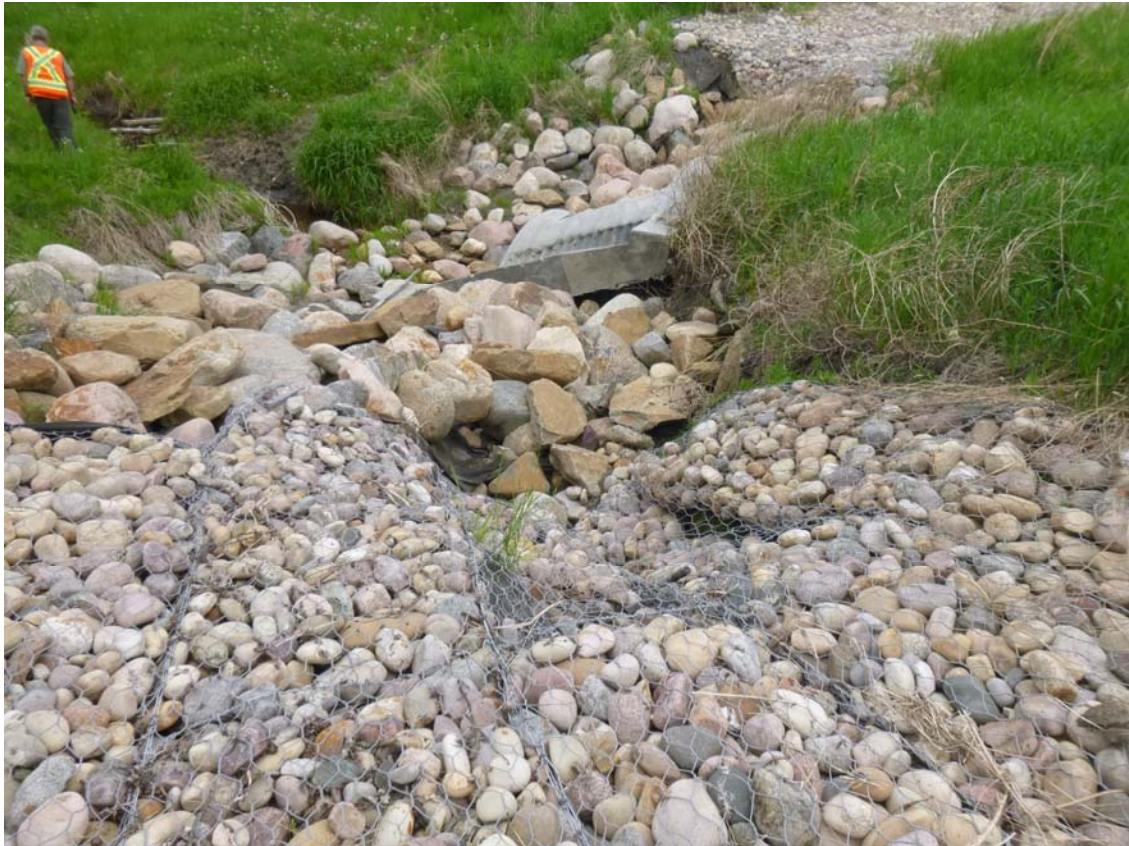
Photo 5 - Looking at the west gabion/riprap transition leading to the culvert inlet. More undermining/erosion has occurred since last year, causing subsidence to the last 2 m length of gabion baskets, and undermining the concrete collar of the culvert inlet.
