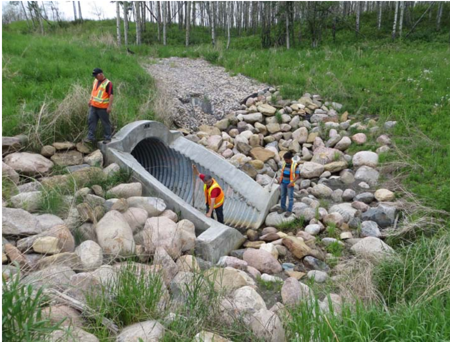
Photo 3 - Looking northwest at the culvert inlet and gabion/riprap transition areas. Note the erosion at the transitions between the gabion and riprap areas on both sides of the culvert.
