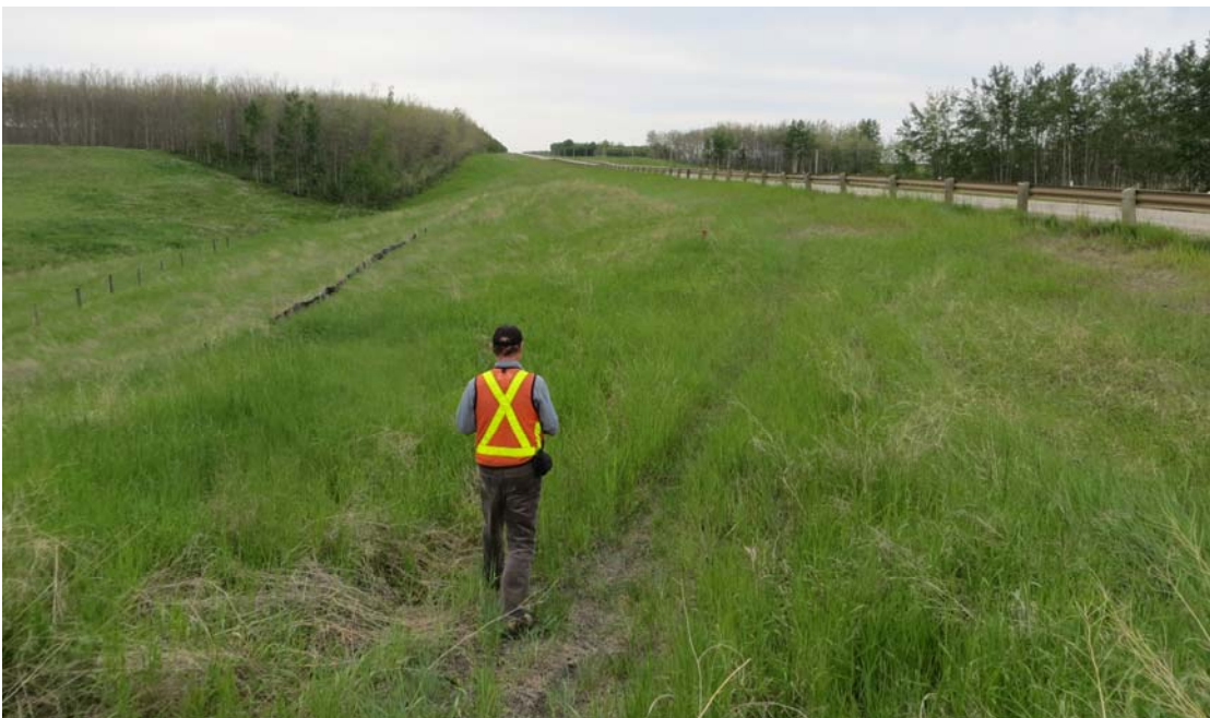
Photo 14 - Looking west parallel to the highway along the well vegetated downstream embankment.
