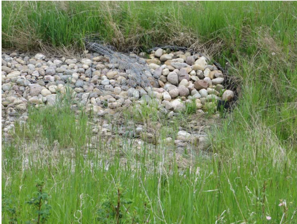
Photo 1 - Looking at a torn gabion mattress wire at the beginning of the west flank on the north side of the highway.
