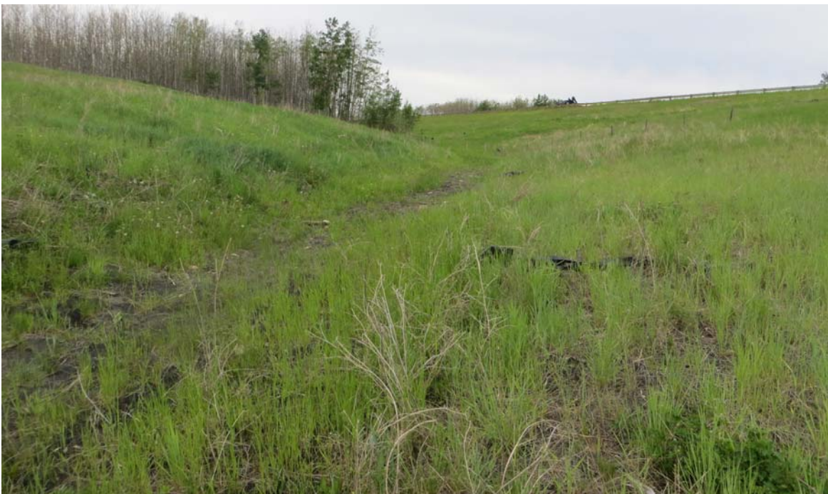
Photo 10 - Looking northwest at the west flank of the beginning of the erosion control soil covering (ECSC) liner south of the highway. Note that the surface runoff erosion observed last year off of the outside edge of the ECSC liner has diminished and is now OK.
