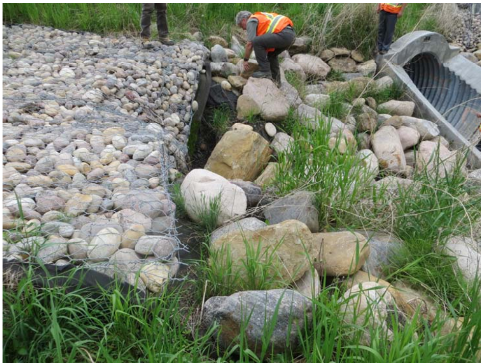
Photo 4 - Looking at the east gabion/riprap transition leading to the culvert inlet. Some more separation and undermining/erosion has occurred since last year, causing distress to the last 1m length of gabion baskets.
