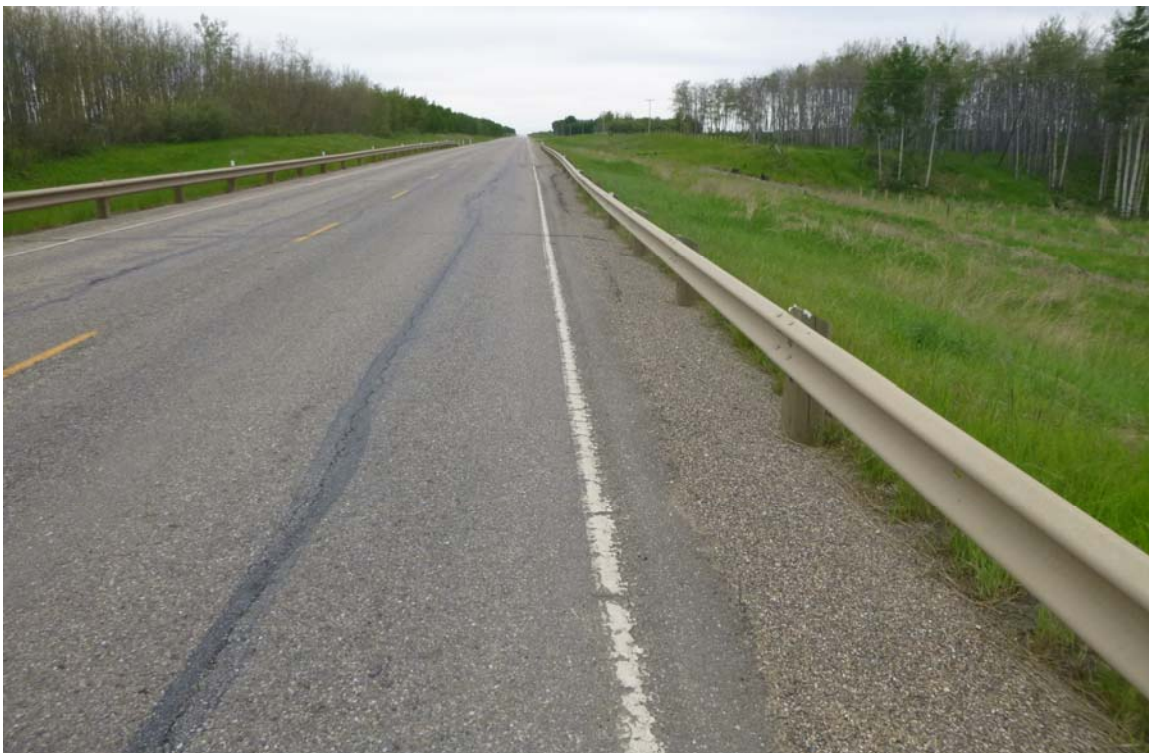
Photo 8 – Looking west along the highway where the north embankment slide has affected the road. The crack along the OWP through the old patch has increased to 30 mm differential this year, and a new crack about 100 mm wide exists along the north edge.
