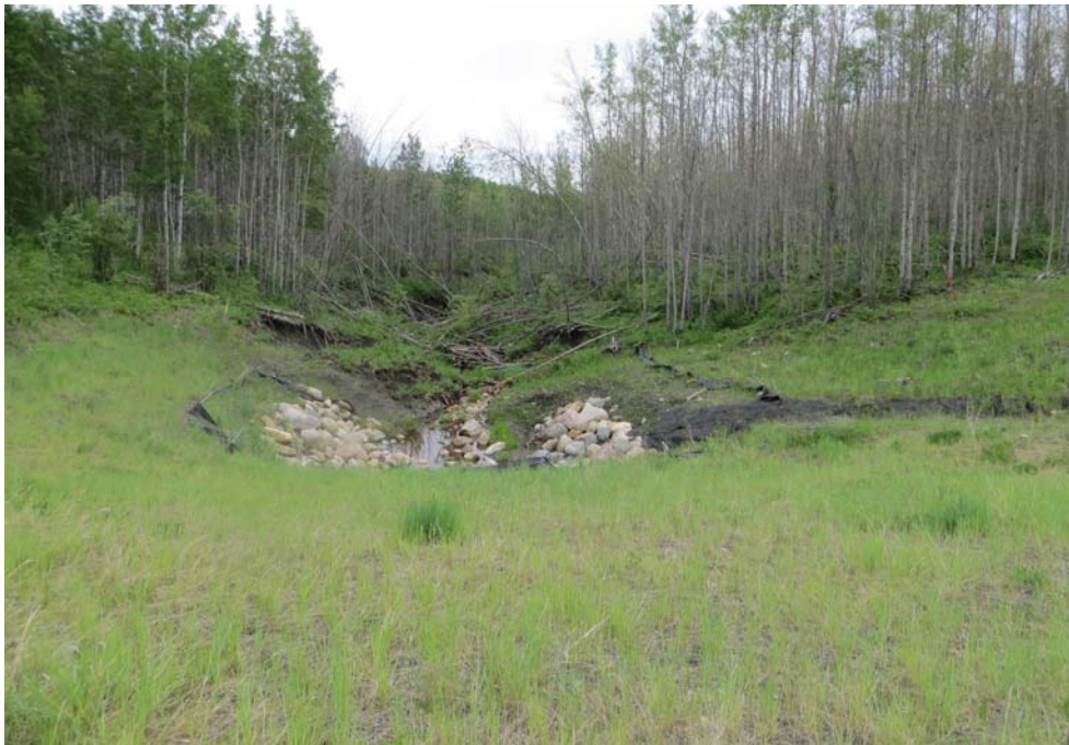
Photo 12 – Looking south at the culvert outlet area. Note the additional slumping on both sides of the drainage channel further downstream of the riprapped area.
