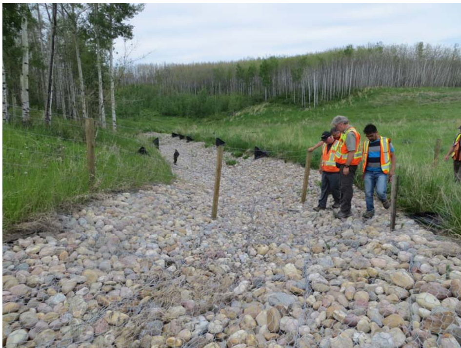
Photo 2 - Looking northeast at the toe of the upstream slope and south gabion leading to the culvert inlet of the north embankment.
