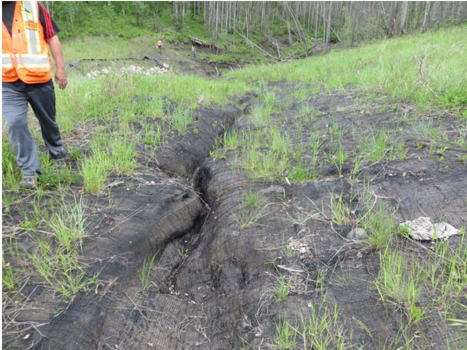
Photo 11 - Looking southeast along the ECSC liner towards the culvert outlet. Note that the erosion control liner has settled neatly overtop of the erosion gully that formed underneath the liner, and now appears to be functioning properly (unchanged from last year).
