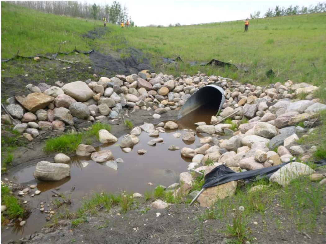
Photo 13 - Looking northwest at the culvert outlet area and downstream embankment slope. Note some of the smaller riprap has washed further downslope.
