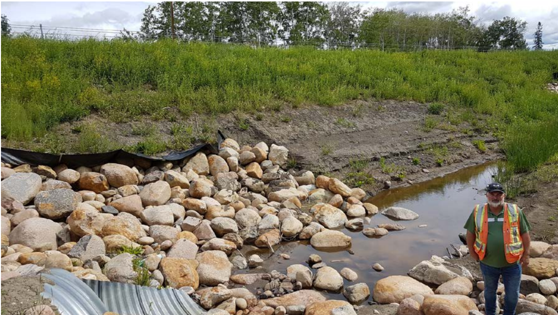
Photo 4 – Looking west at bare area at culvert outlet where possible tension cracks may be forming. Subdrain outlet is just on the far side of the culvert outlet.
