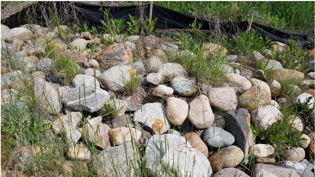
Photo 8 – Looking at riprap placed over bare ground (no non-woven fabric below) at east end of north ditch at the outlet of BF72371.
