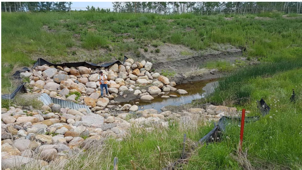
Photo 4 – Looking west at bare area at culvert outlet where possible tension cracks may be forming. Subdrain outlet is just on the far side of the culvert outlet. Note the eroded bare spot just beyond the riprap.
