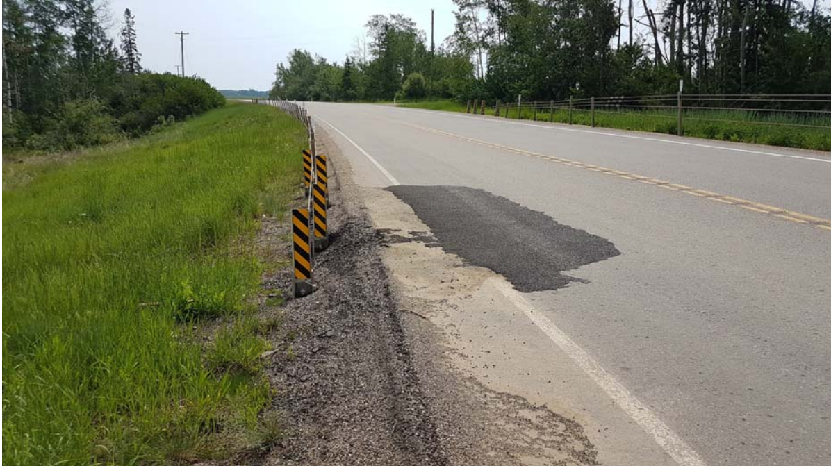
Photo 7 – Looking east at voids around HTSCB posts and settlement cracking of the pavement at west end of the north barrier located by the outlet of BF72371 culvert. Note that two patches have been required in this area.
