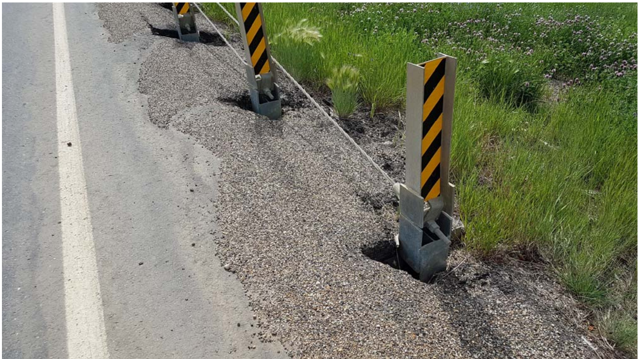
Photo 2 – Looking at voids around HTSCB on south side of highway at the west end.
