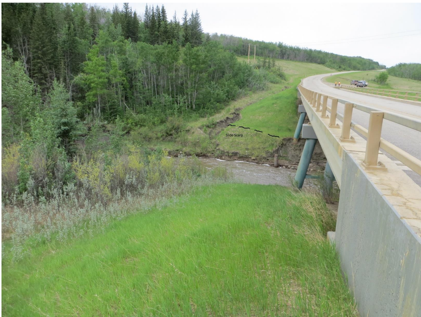
Site 2 Erosion (7 to 20% Ditch Grades)
