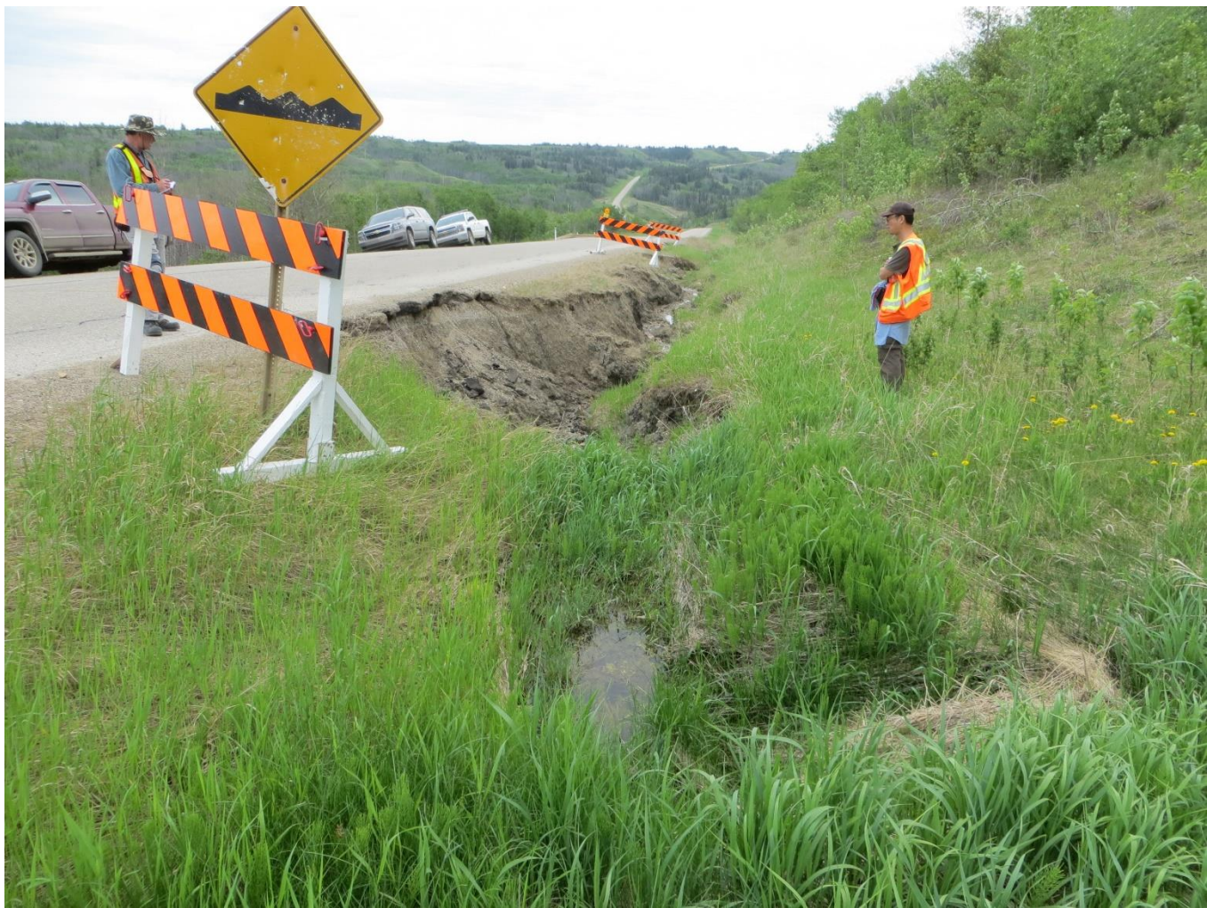
Site 1 Erosion (6 to 8% Ditch Grades)
