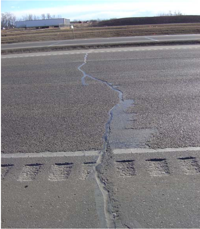
Sealant is performing very well
