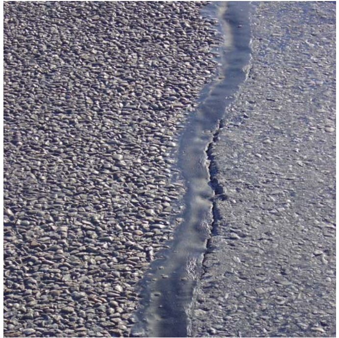
Sidewall adhesion failure
