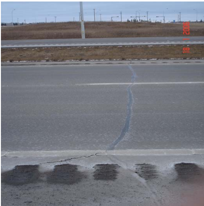
Sealant working as intended (providing a good seal)
