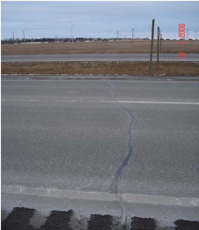
Transverse crack (SBL)
