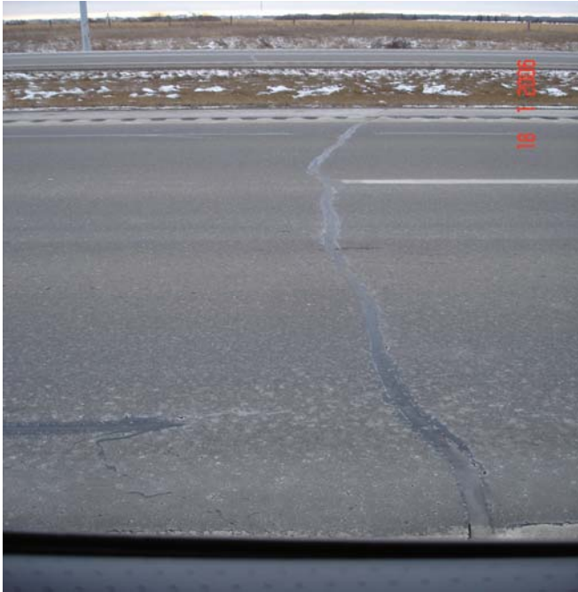
Transverse crack in good shape (NBL)
