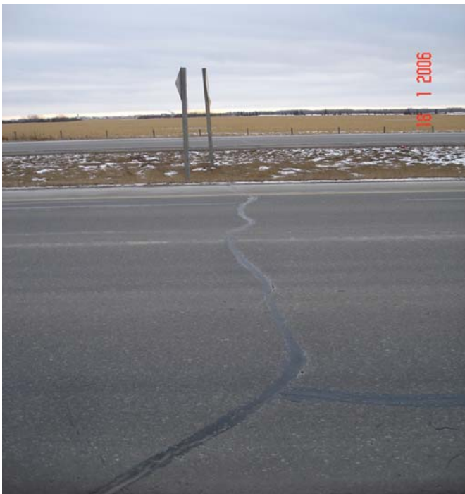
Transverse crack providing an excellent seal (NBL)
