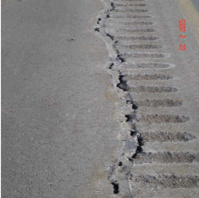
Longitudinal crack, pavement opened up along shoulder
