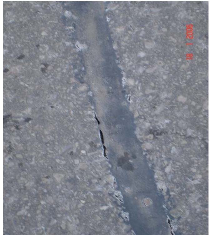
Small amount of adhesion failure
