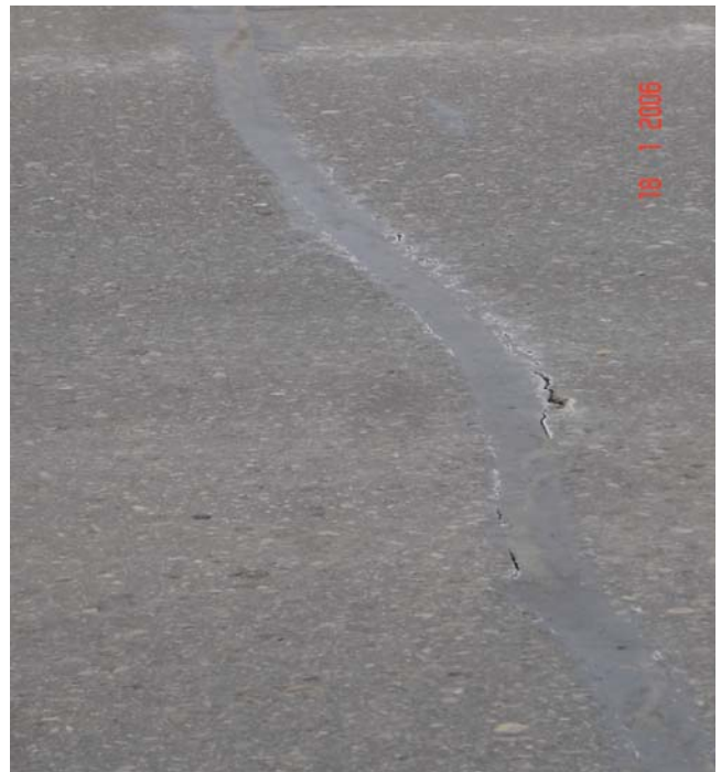
Close-up, small amount of side wall adhesion problem
