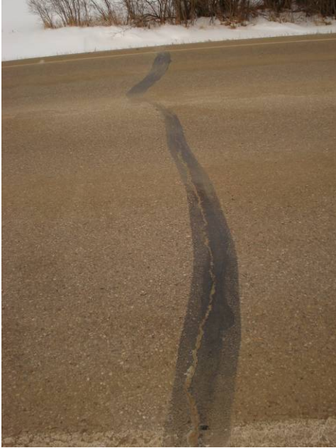
Transverse crack, treated with Deery #3723 sealant
