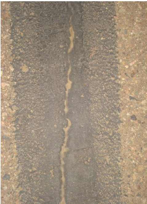
Crack completely filled, no signs of distress
