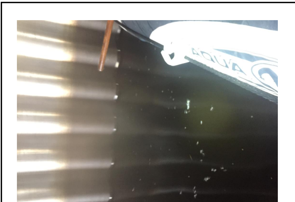
Water staining on the side of the pipe.
