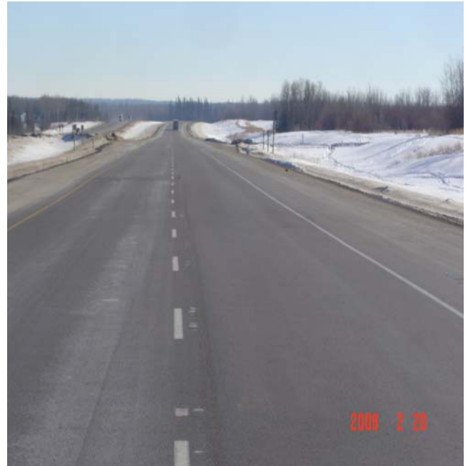
Normal waterborne paint system on newer pavement, durability is poor.
