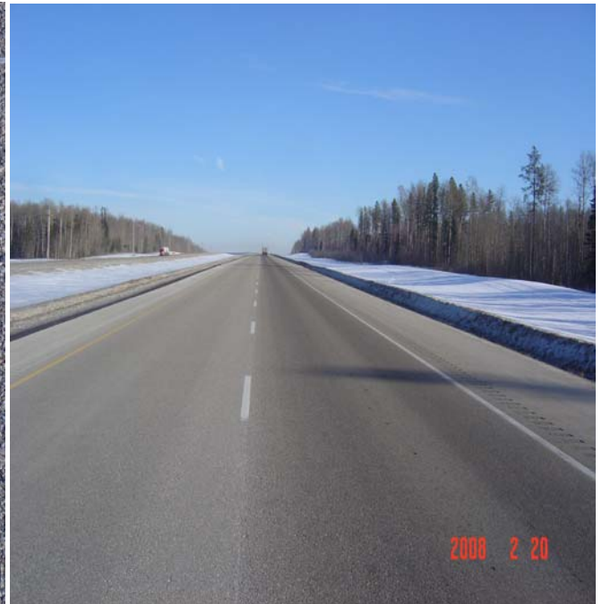
Looking south, HD-21A paint looks good, however not as good as the last section. There is more bead loss on white & yellow edge lines, however durability is fine. The HD-21A May provide one more year of service.
