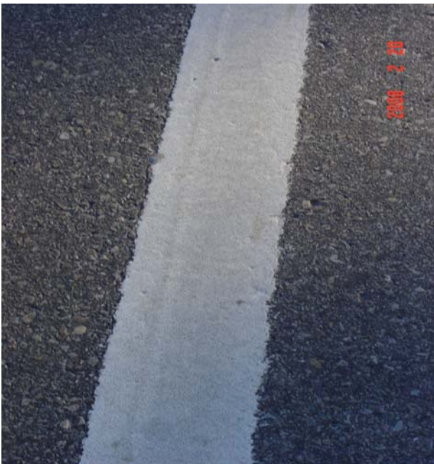
White edge line: paint is in excellent shape Retro readings: 101, 113, 94, 98, 93, 90, 97, 100, 104 Average: 99 Mcd
