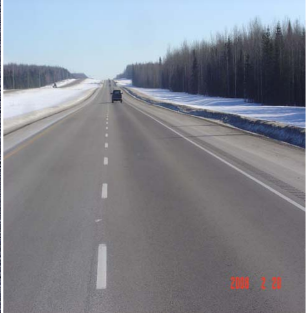
Looking south, paint in good condition. It appears that there is no need to repaint this section in 2008.
