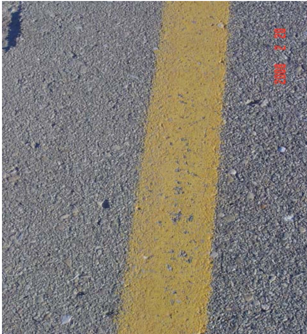
Yellow edge line: some loss of paint and chipping Retro readings: 42, 44, 45, 44, 47, 46, 47, 51, 46, 46, 56 Average: 47 Mcd
