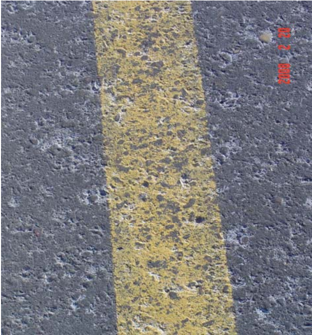
Yellow edge line: paint is faded and chipped. Retro readings: 59, 49, 46, 51, 54, 51, 48, 55, 57, 49, 59 Average: 52 Mcd
