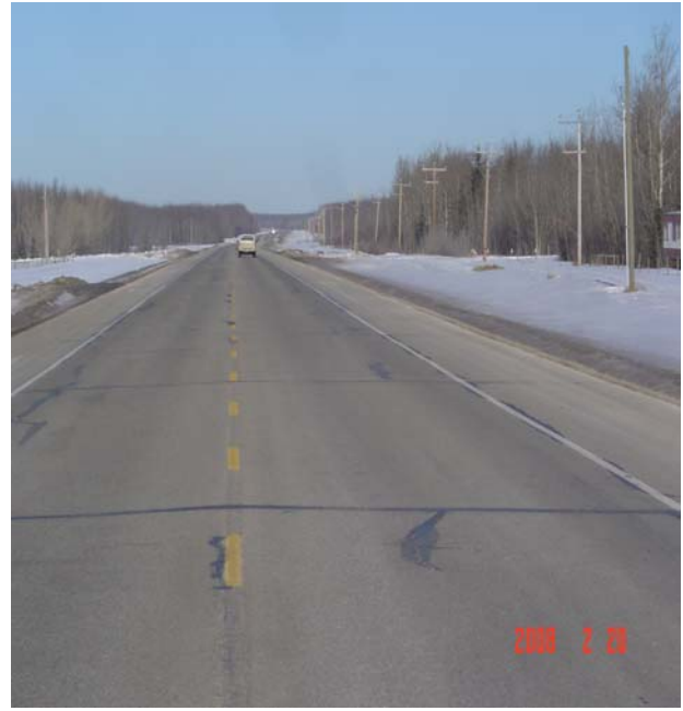
Overall look of alkyd paint system Alkyd appearance is good.
