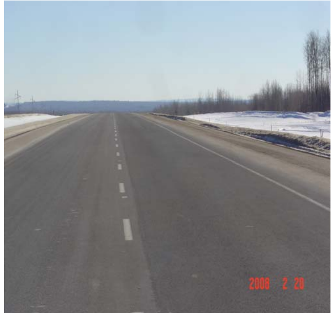
Normal waterborne paint system on newer pavement, edge lines are poor, skip line is good.
