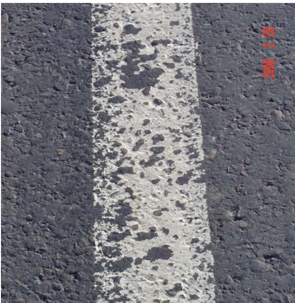
White edge line: paint is chipped, loss of glass beads. Retro readings: 90, 75, 40, 50, 71, 97, 84, 74, 87, 86, 97, 72 Average: 77 Mcd
