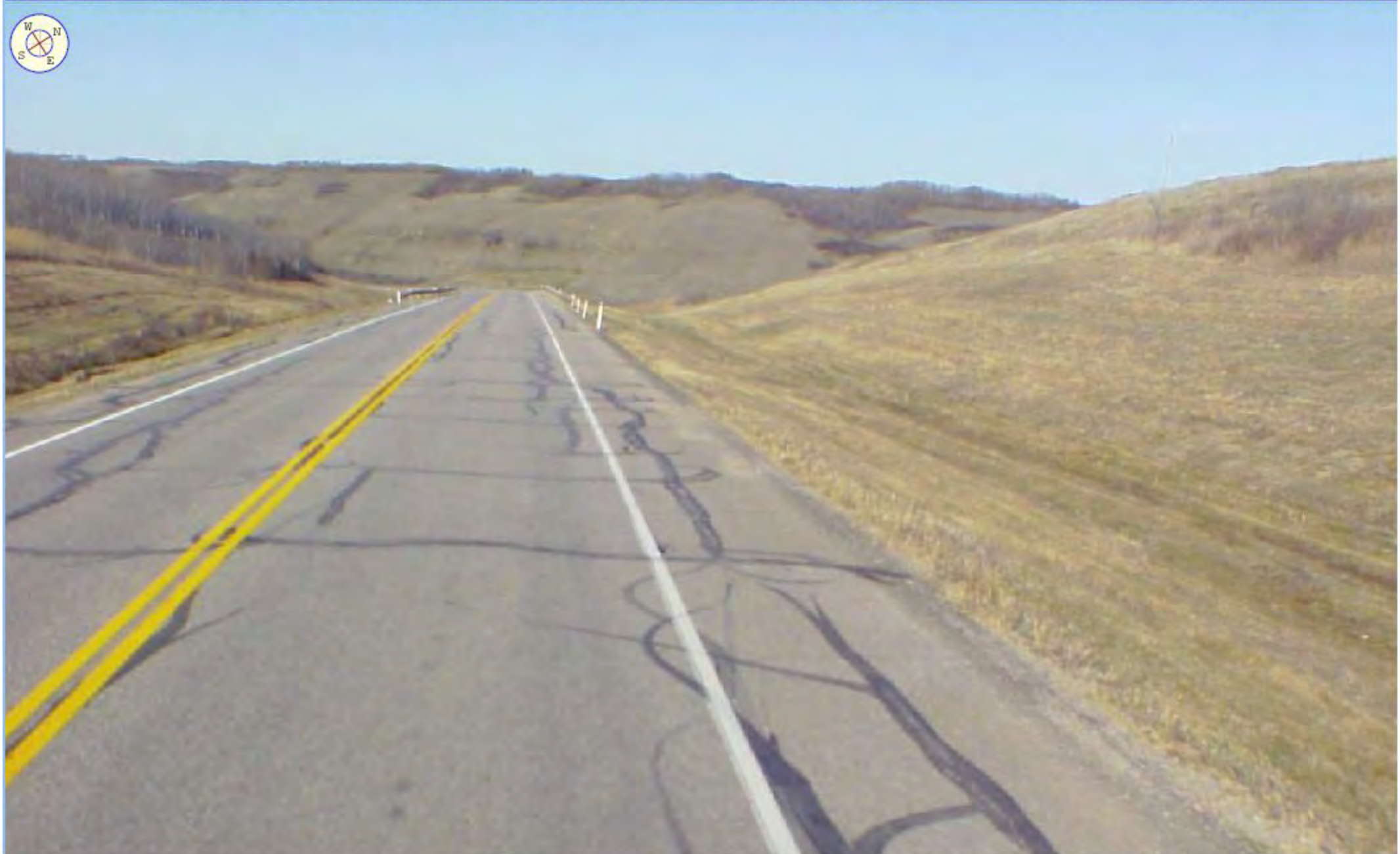
Hwy 14:16 km 48.6 Multiflow Dewatering Project, North Ditch west view before construction, 9 June 2013
