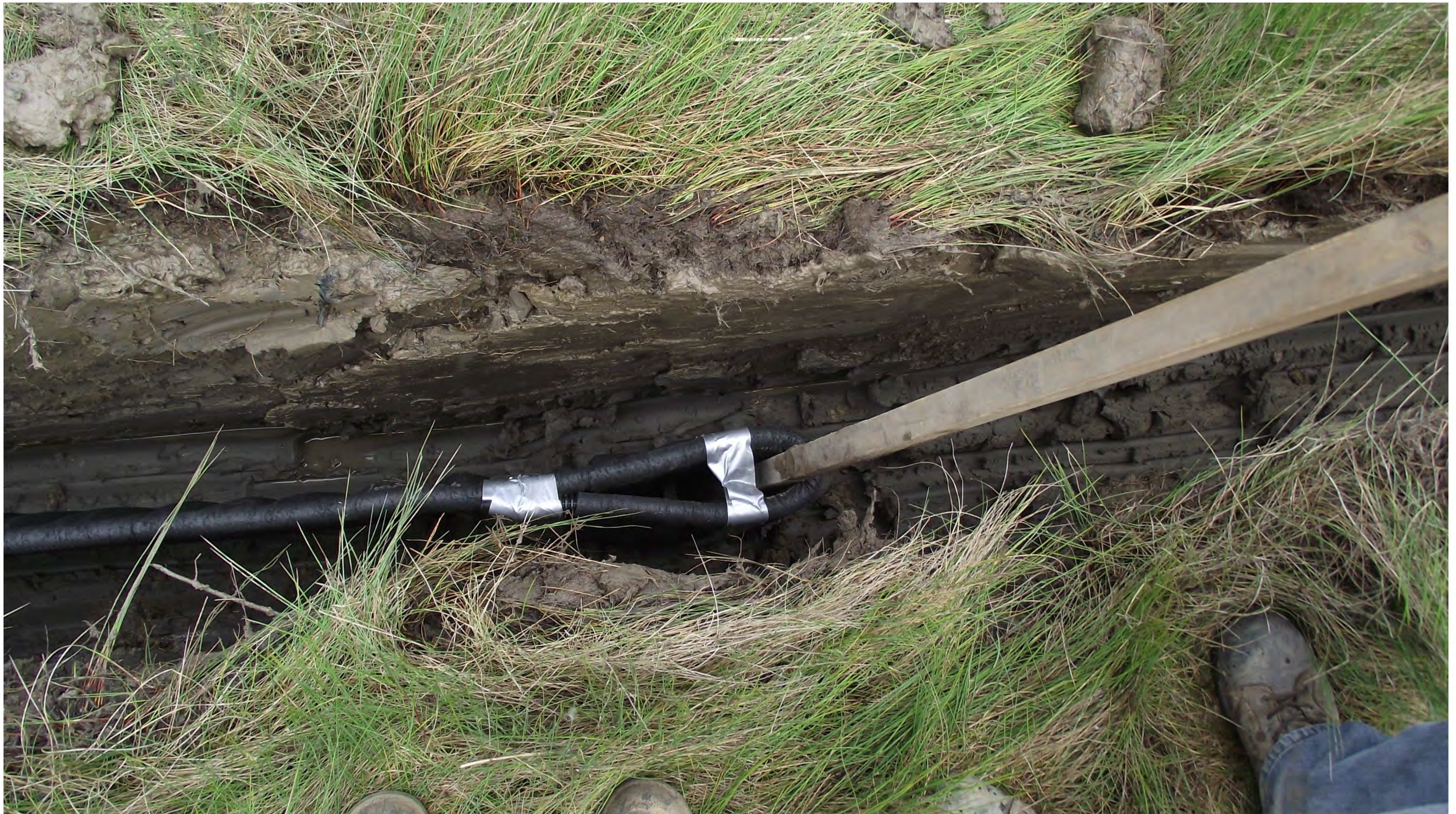
Hwy 14:16, km. 48.6, Multiflow installation south ditch, setting terminal end 200 metres from outfall, 9 June, 2011
