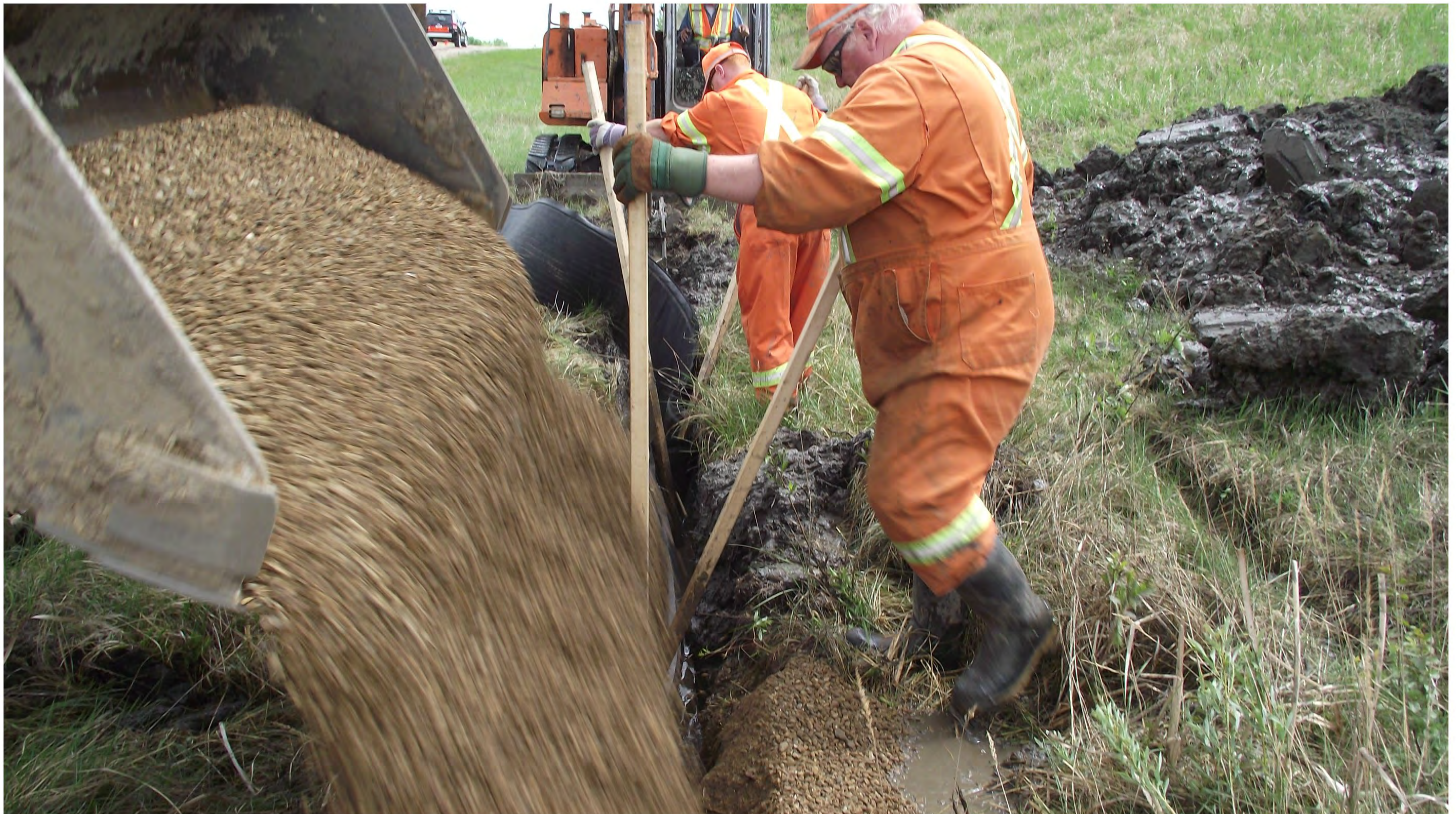
Hwy 14:16, km. 48.6, Multiflow installation south ditch, adding washed pea gravel to ditch (note 2x2 stakes are holding Multiflow vertical and centered in trench), 9 June, 2011
