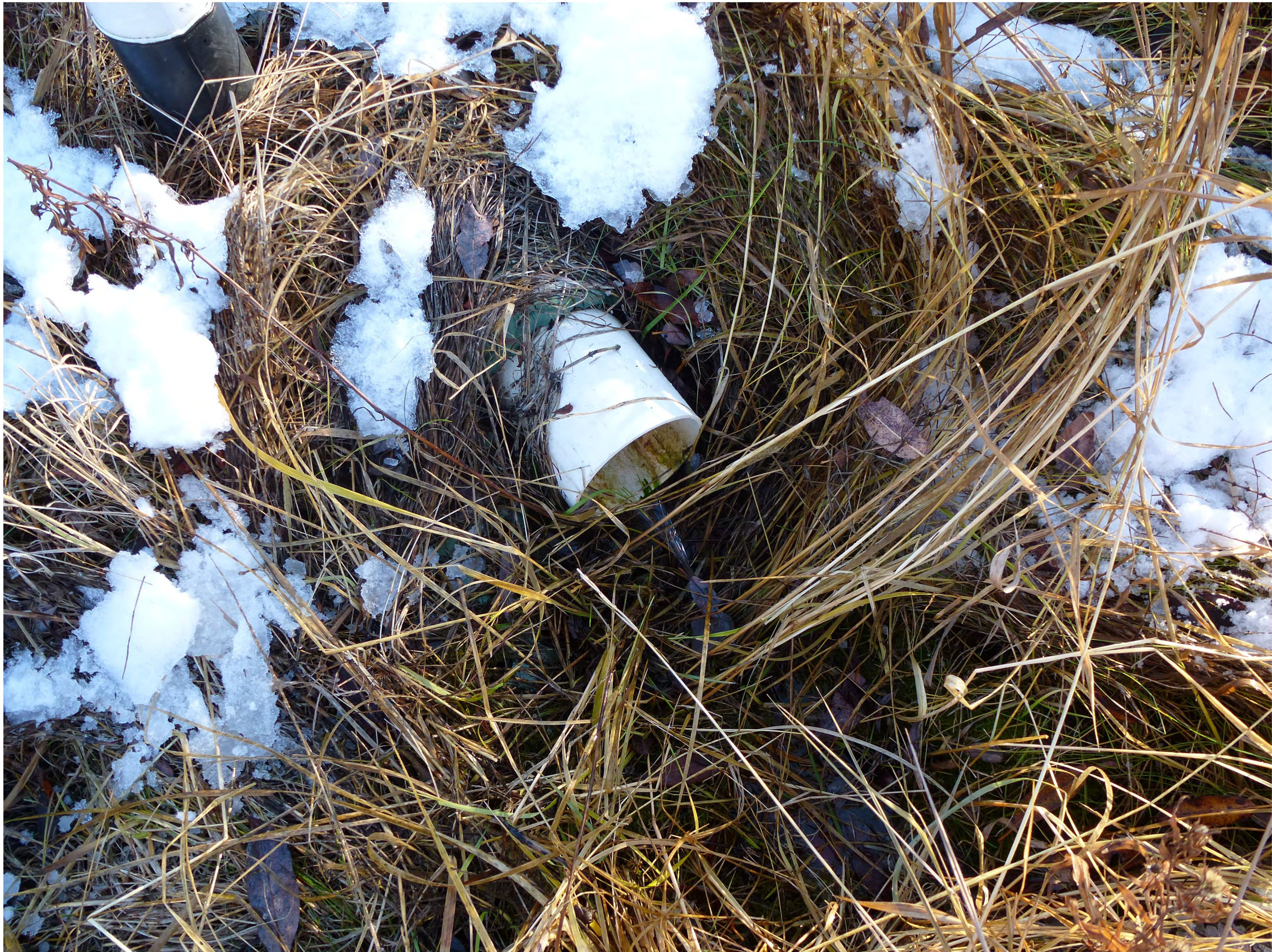
Hwy 14:16, km. 48.6, Multiflow installation inspection of 100mm outflow pipe, south ditch, 5 November, 2014
