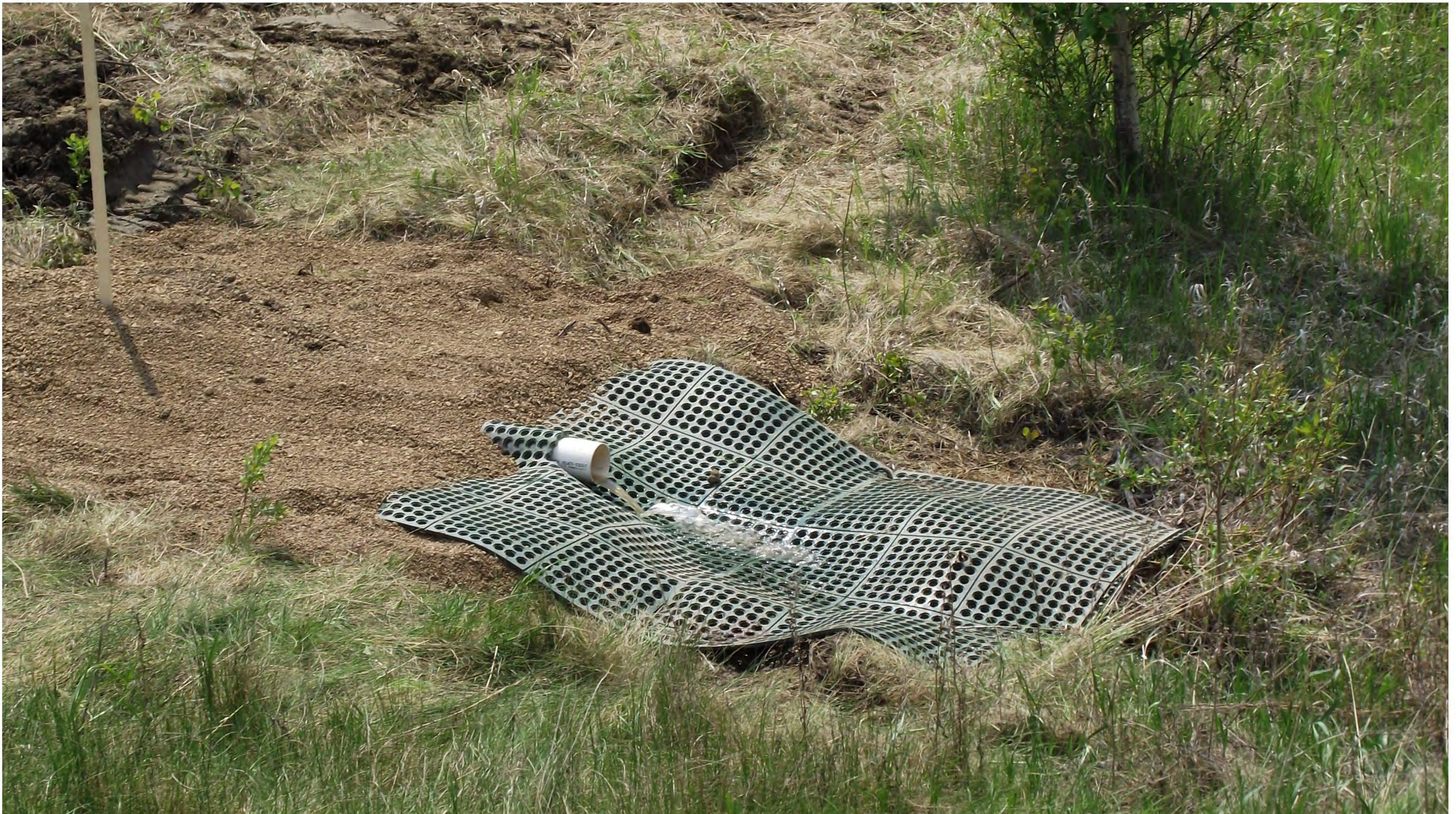
Hwy 14:16, km. 48.6, Multiflow installation south ditch, 100mm outfall and Shoremax protection, 9 June, 2011
