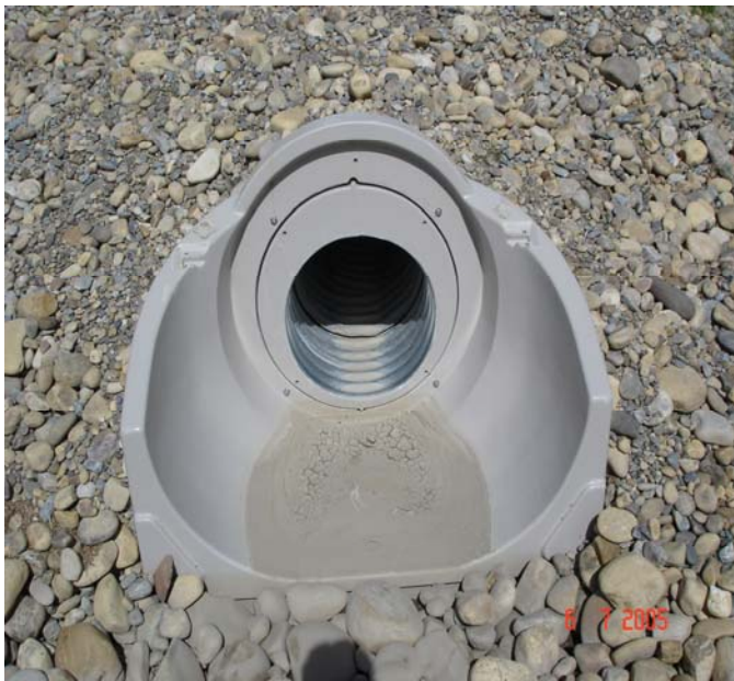
End treatment no grate
