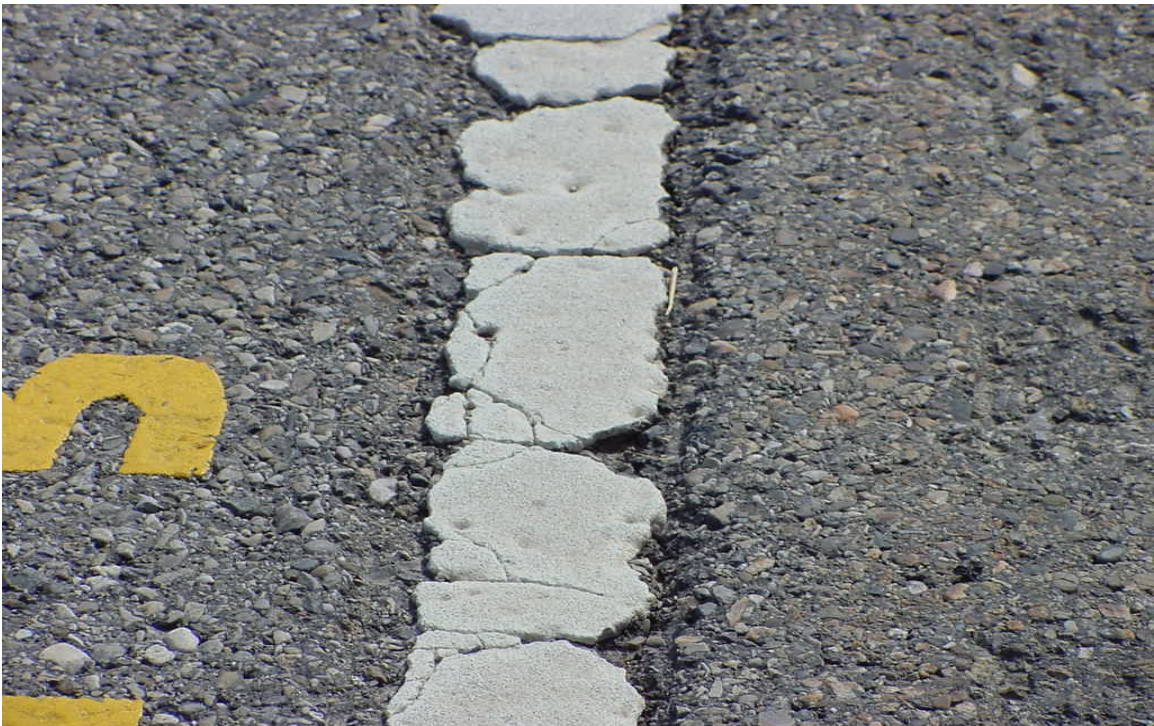
Line marking is in poor condition with some sections debonding.
