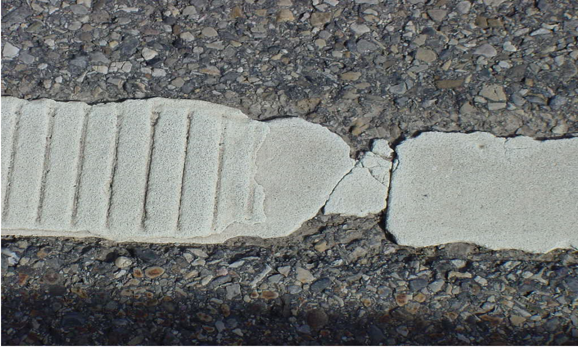
The thinner (un-grooved) layer is not performing very well (Line marking supplied by other manufacturer). The majority of this section is in poor condition with no bead retention.
