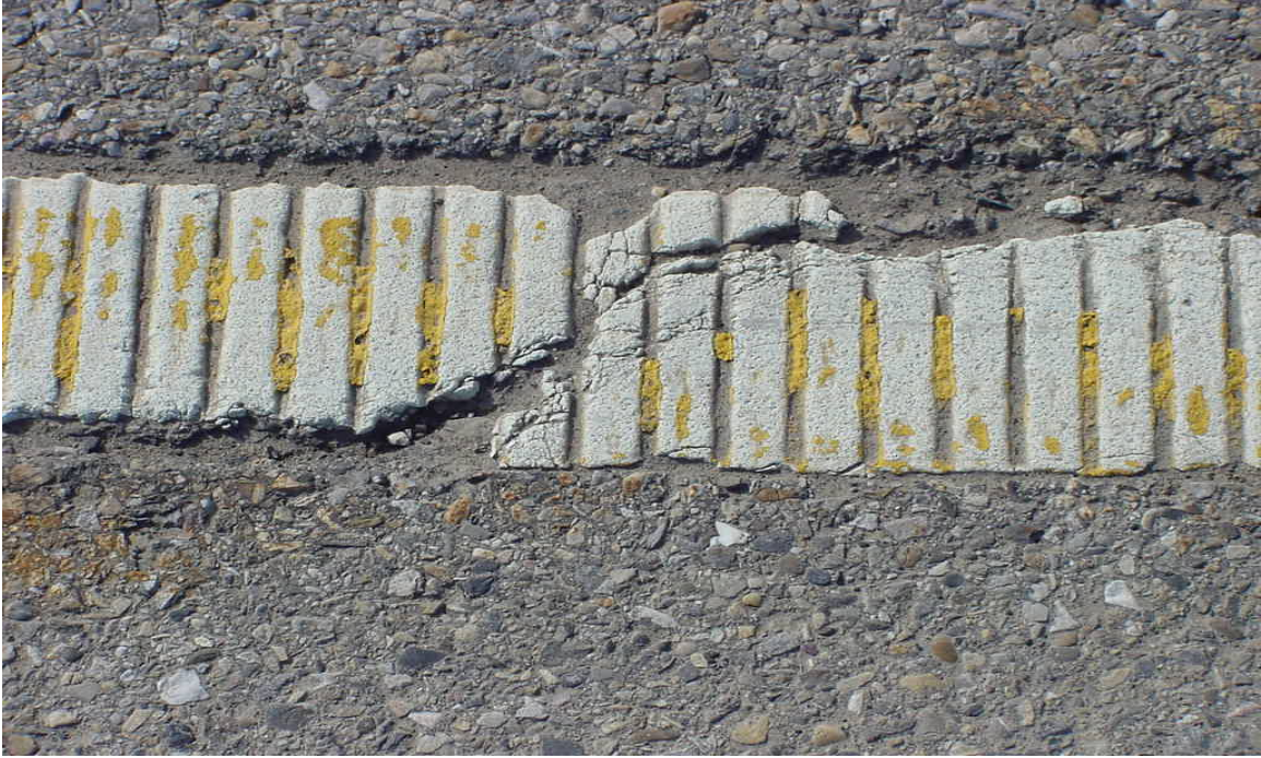
A section of Rainline that is damaged. This section appears to have been painted with yellow paint.
