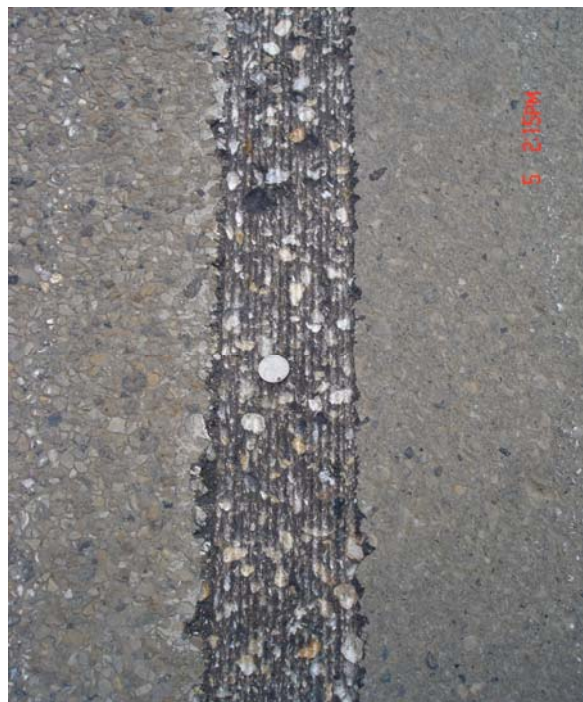
Close-up, jagged edge of seal coat
