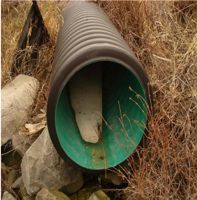
Soleno culvert (600mm diameter)
