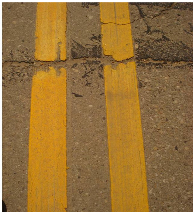
Close-up, snow plow damage
