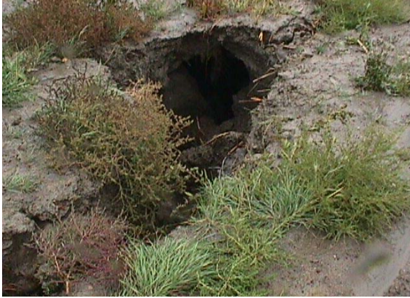
Subterranean erosion channel is formed below the east ditch in Hwy 837:02
