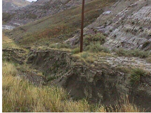
Deep erosion gully is formed in the west ditch in Hwy 841:02
