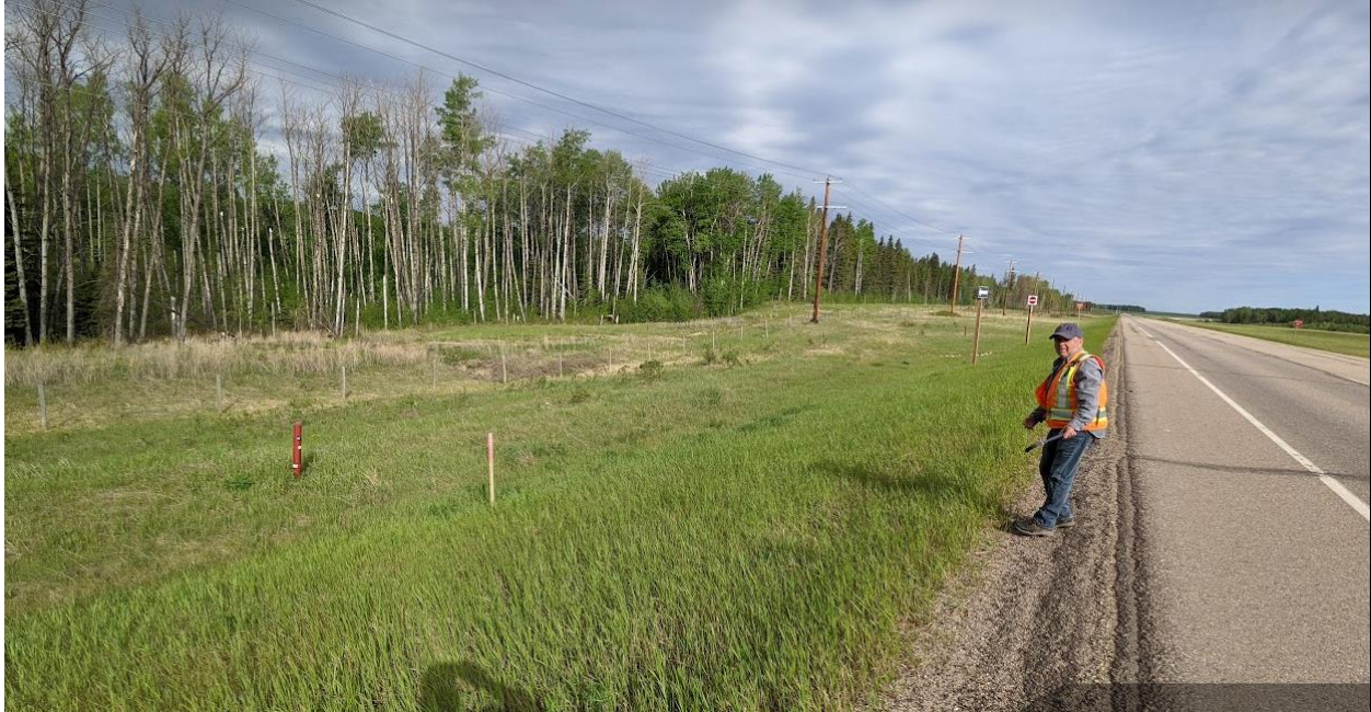
Photo No. 7 – Looking north at highway southbound lanes; landslide is not currently impacting the highway surface; head scarp crack is about 6.5 m away from the edge of pavement
