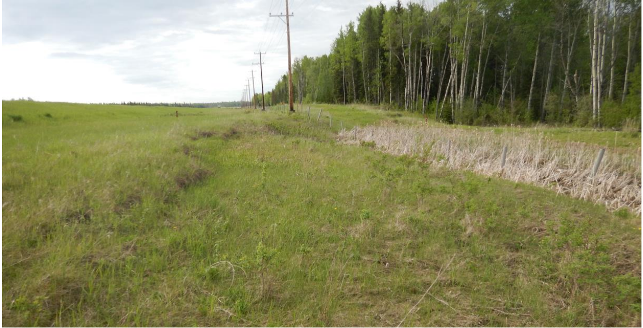
Photo No.3 – Looking south at the southern flank of the landslide (700 mm wide, 600-800 mm deep); water ponding along the ditch between the trail and the fence (note cattails in this area)
