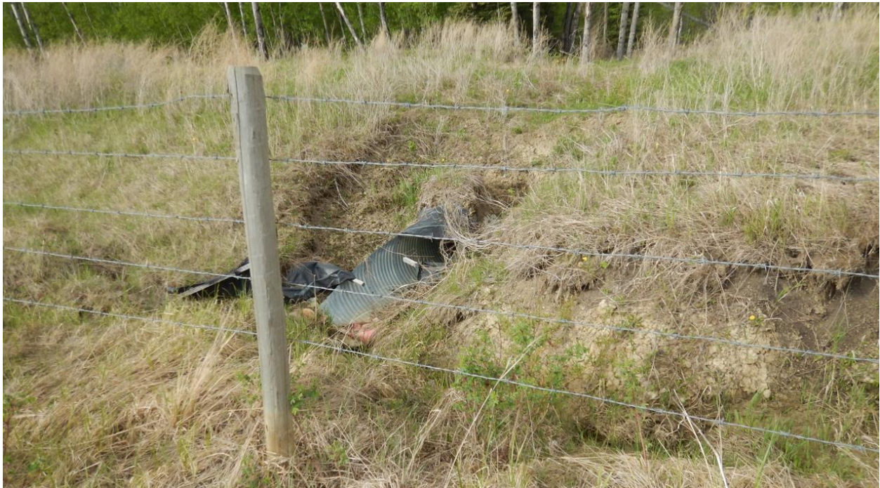
Photo No.2 – Sinkhole above the 800 mm diameter culvert; looking at the culvert inlet
