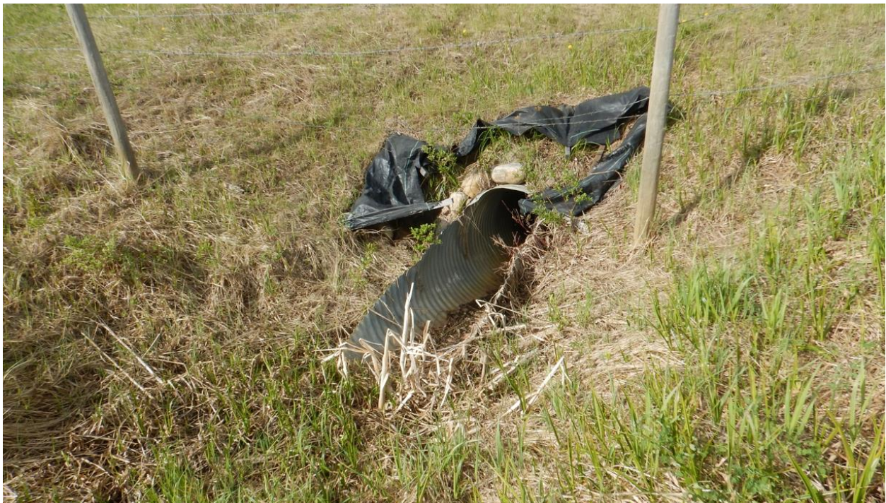
Photo No.6 – 700 mm diameter CSP culvert C3 inlet; culvert separated; minor flow noted in 2021
