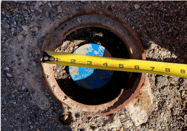
Photo 1 Flush-mounted casing protector installed in the south shoulder of Hwy 579:02 to protect the SI05-07.
