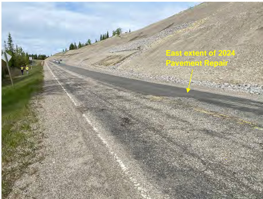
Photo 4: Pavement condition at east extent of site. Looking west.
