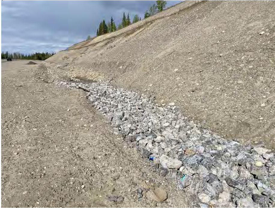
Photo 9: Transition from gabion mattress to riprap ditch at toe of new backslope. Looking southwest.
