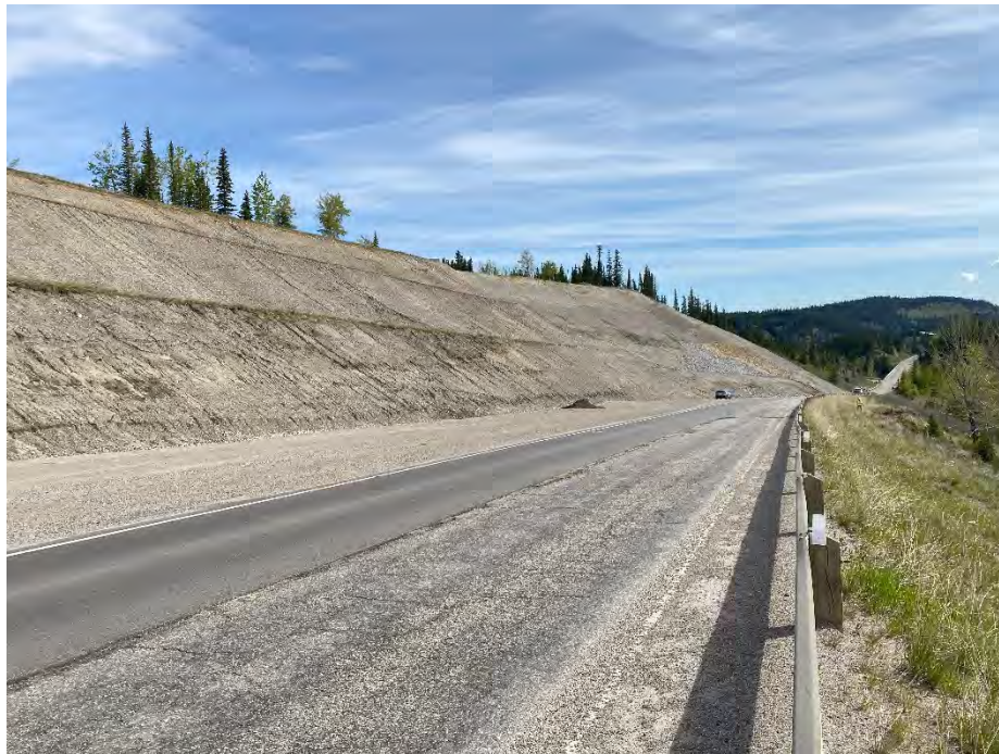
Photo 2: Pavement condition and benched backslope constructed for highway realignment, above south scarp area near west extent. Looking northeast.
