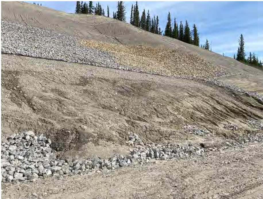
Photo 10: Erosion and seepage on recently completed backslope. Looking northeast.
