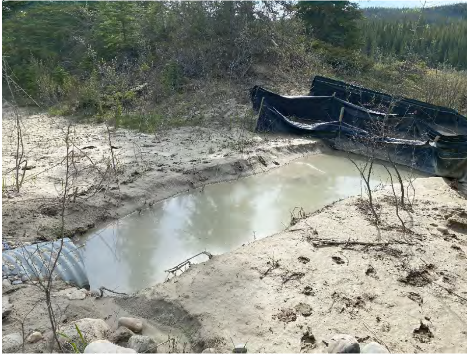
Photo 13: Ponded water and sedimentation at culvert outlet. Looking southeast.
