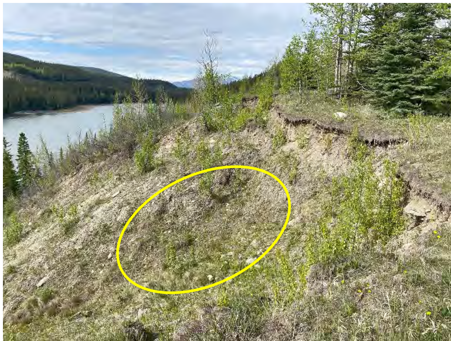
Photo 6: Seepage near middle of east landslide. Looking southwest.
