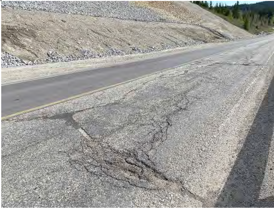
Photo 3: Pavement cracking in EBL north from half-culvert collector drain. Looking northeast.
