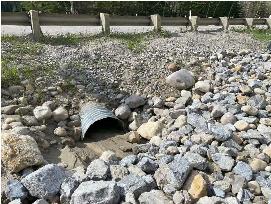
Photo 12: Culvert at east end of site, half filled with sediment. Looking south.
