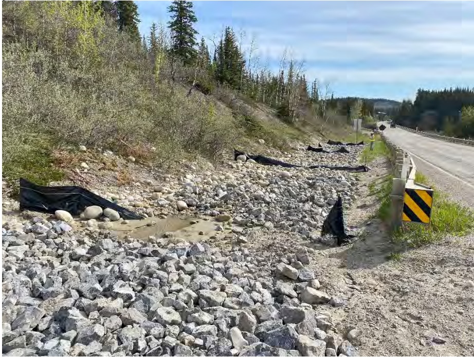
Photo 11: Sedimentation in riprap lined ditch east of slope repair. Silt fence in disrepair. Looking east.
