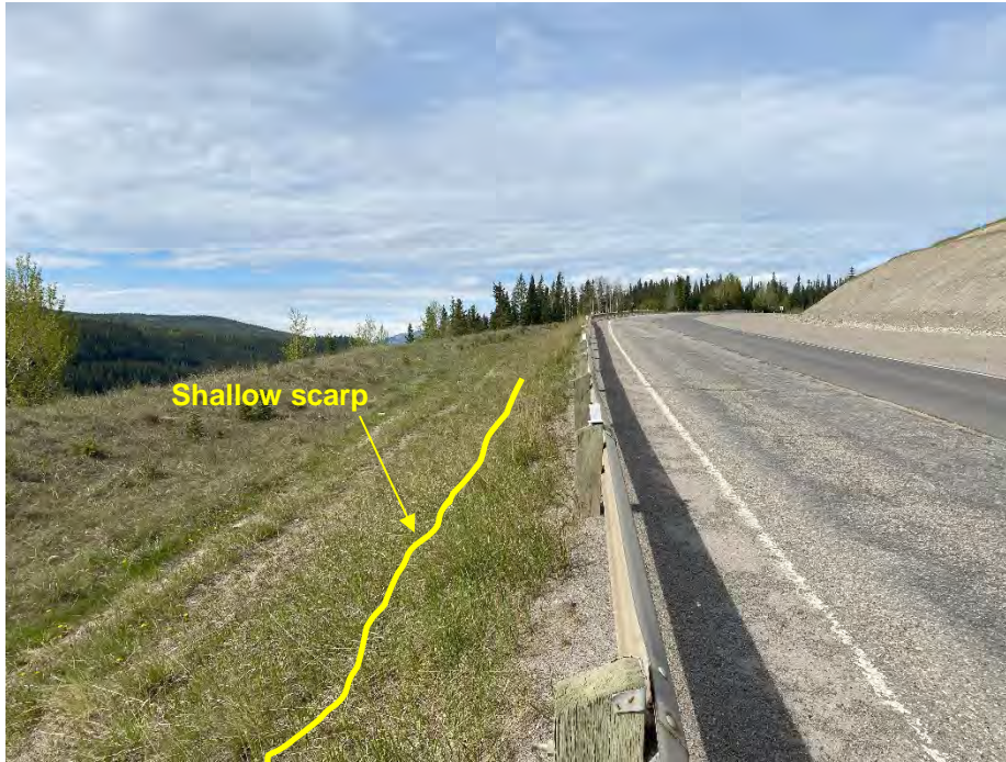
Photo 1: Pavement and upper south slope condition at west extent of east landslide scarp. Looking southwest.
