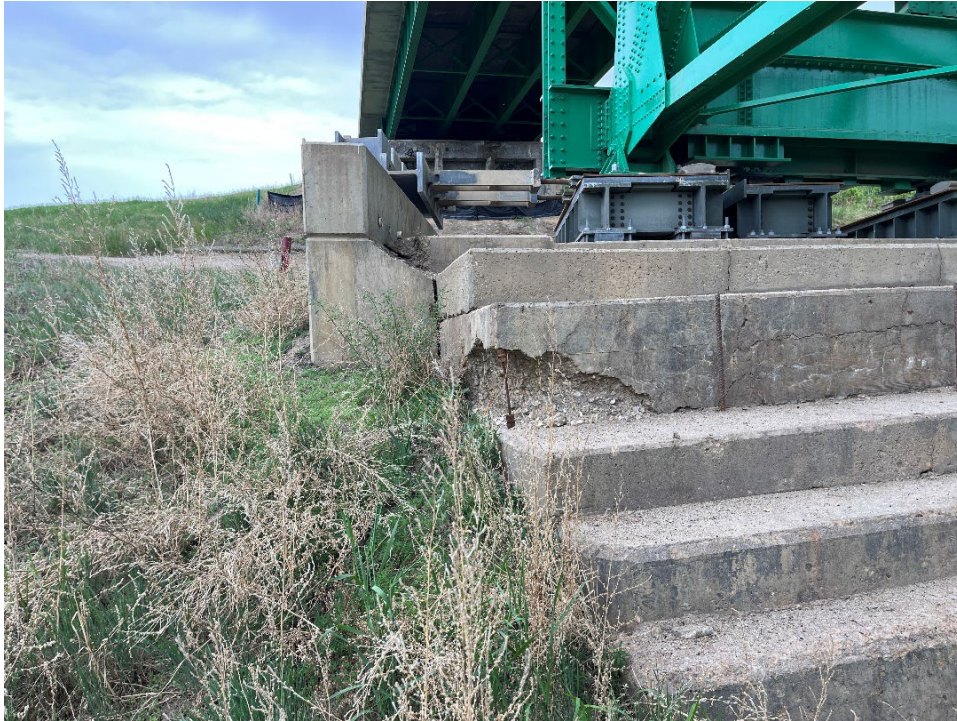
Photo 9 – Looking west at Pier 1 foundation which is tilted downward to the south. The angle from horizontal was 4° at the top and 7° at the bottom stage. Concrete has started to crack and spall.
