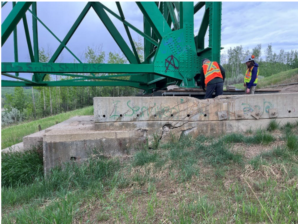
Photo 8 – Looking south at Pier 1 wingwall at arc-shaped compression crack pattern in foundation. Left-hand portion of foundation is pile supported; right-hand is on-grade.
