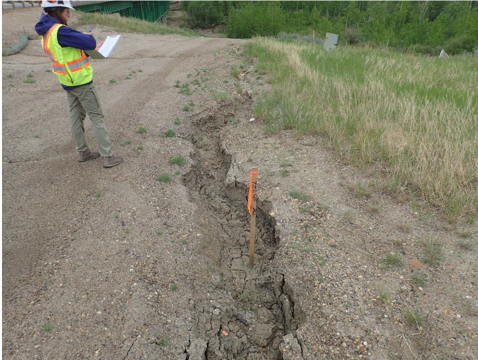
Photo 13 – Looking east at erosion gully formed along buried Telus cable trench.
