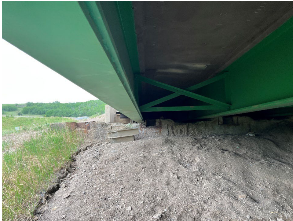
Photo 3 – Looking towards the West Abutment where portions of the old foundation concrete was removed to allow movement of the girders between the West Abutment and Abutment 1.
