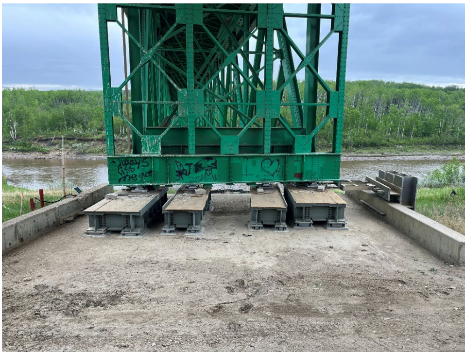
Photo 6 – New slide plates installed at Pier 1. TEC Bridge Department has been monitoring the movement of the slider plates.
