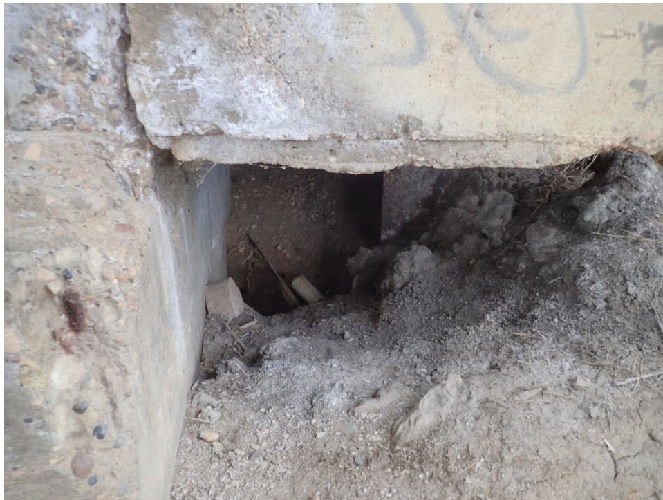
Photo 4 - Void underneath the northeast corner of the old Abutment 1.
