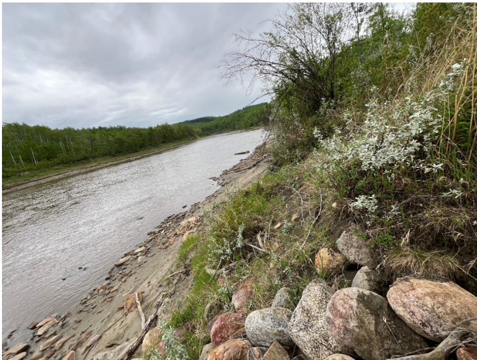
Photo 12 – Looking south at erosion along toe of riprap and riverbank.
