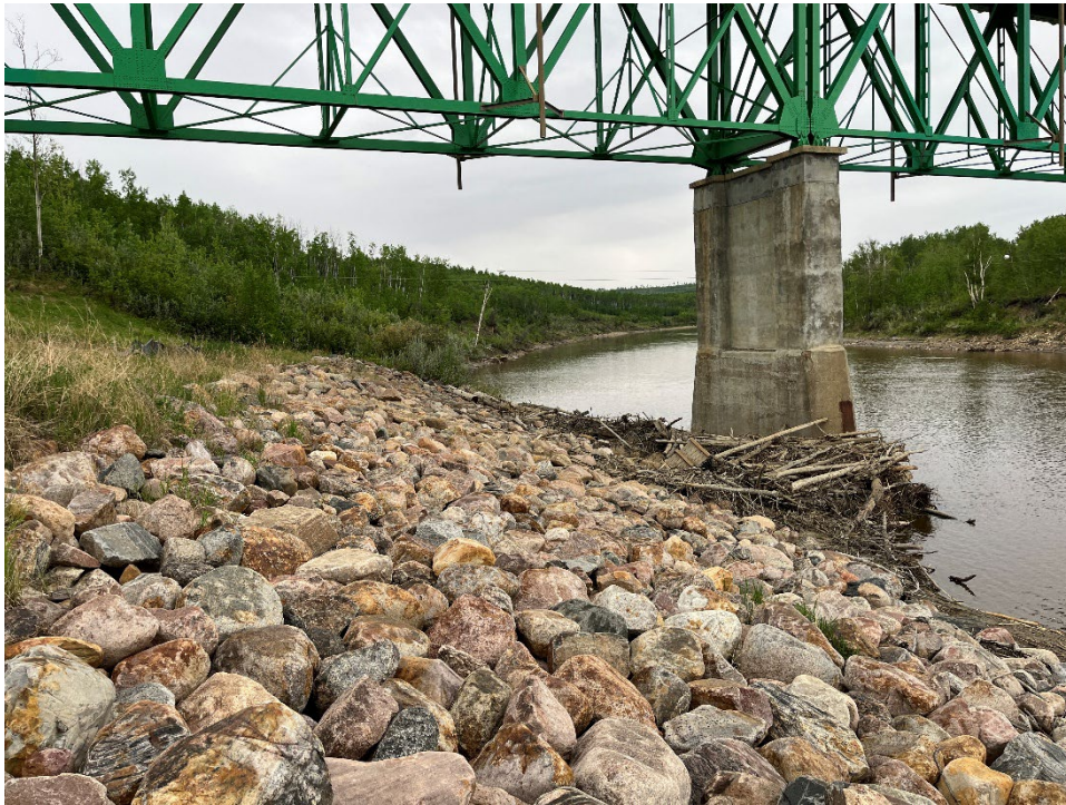
Photo 11 – Looking north at accumulated tree debris against Pier 2.
