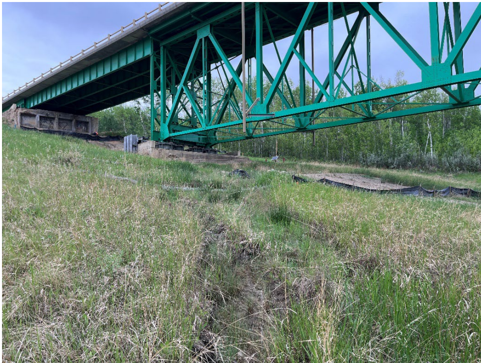
Photo 10 – Looking west toward Pier 1 at rutting and installed erosion control measures. Some of the area has vegetated since.
