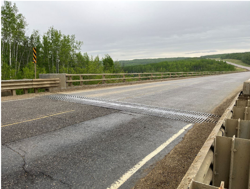
Photo 1 – Looking northeast at new finger joints and repaved approach (done since 2023 inspection).
