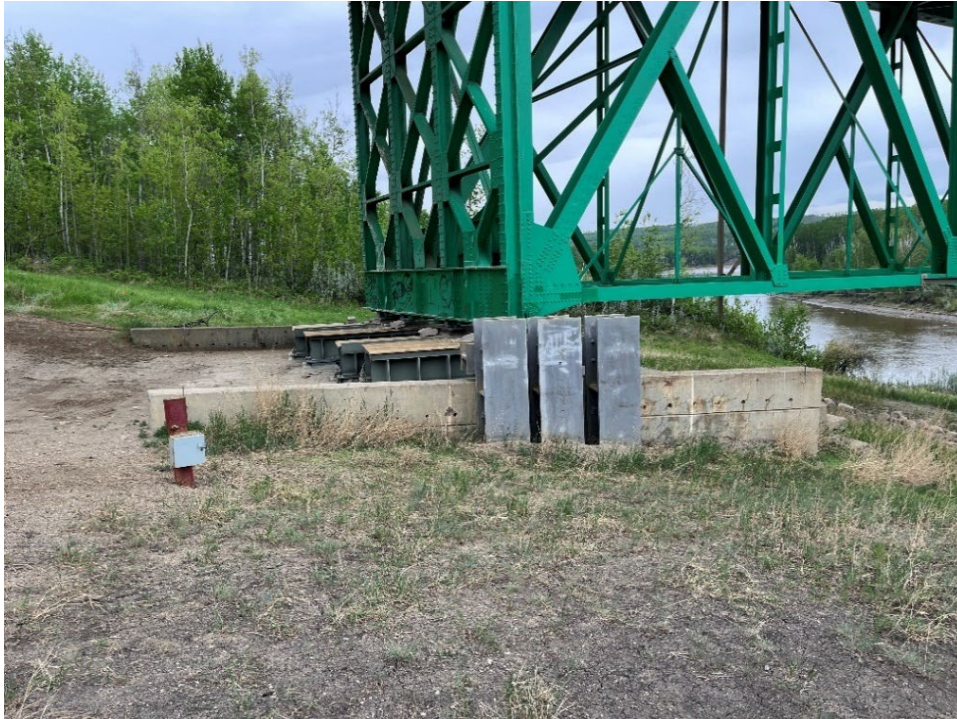
Photo 7 – Looking north at Pier 1 where sliding plates and lateral restraints were installed in 2023.
