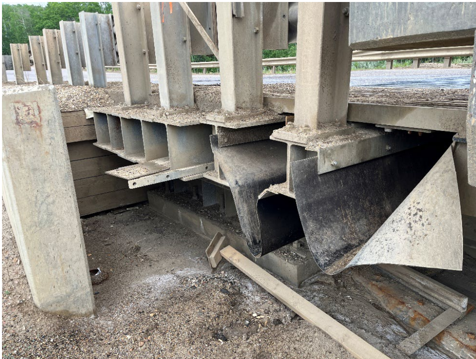
Photo 2 – Looking north at west bridge abutment. New I-beam added in 2025 (6 total) plus one below the finger joints. The tarps were added in 2024.
