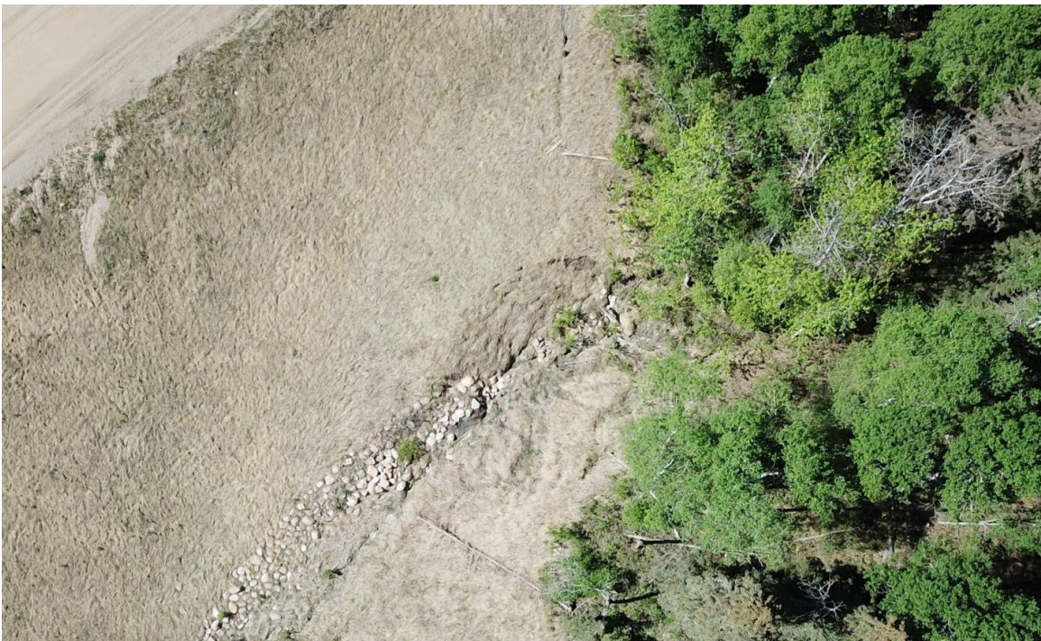
UAV 2023 UAV Image – Slumping at the north end of the of the riprap-lined channel on the east embankment.
