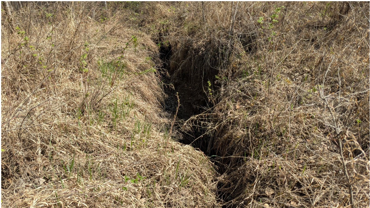
Photo 8 – 900 mm-dia. culvert outlet and gully at the north end of the site.
