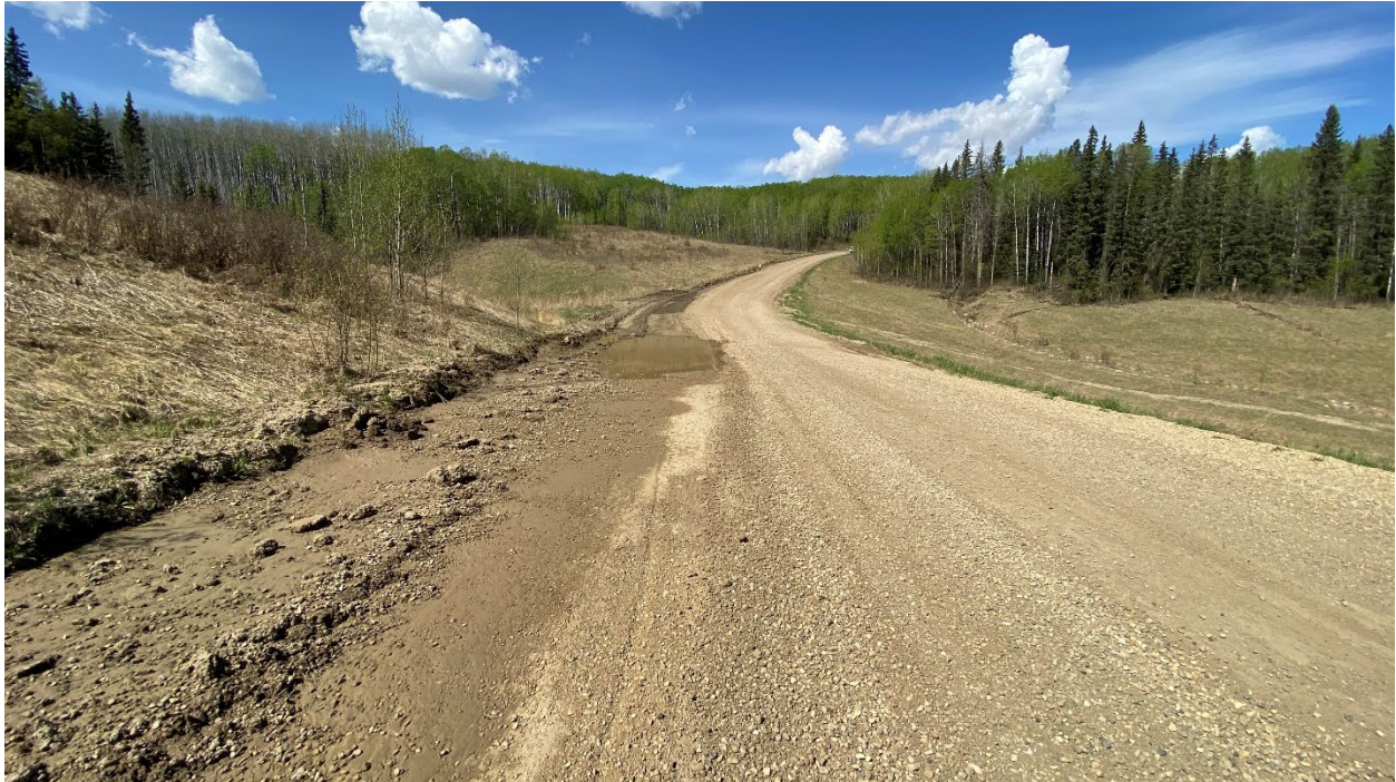
Photo 7 – Looking at seepage along west side of road near the south end of the site.
