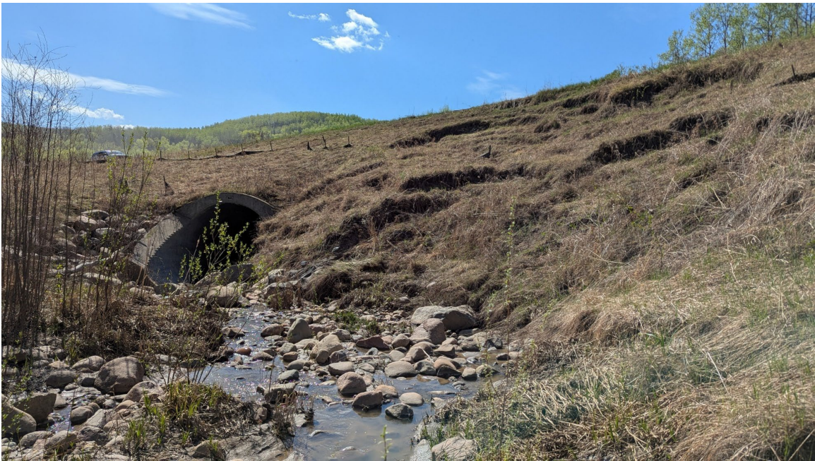
Site 1, Photo 2 – Looking southeast at creek bank slumping upstream of the culvert inlet.
