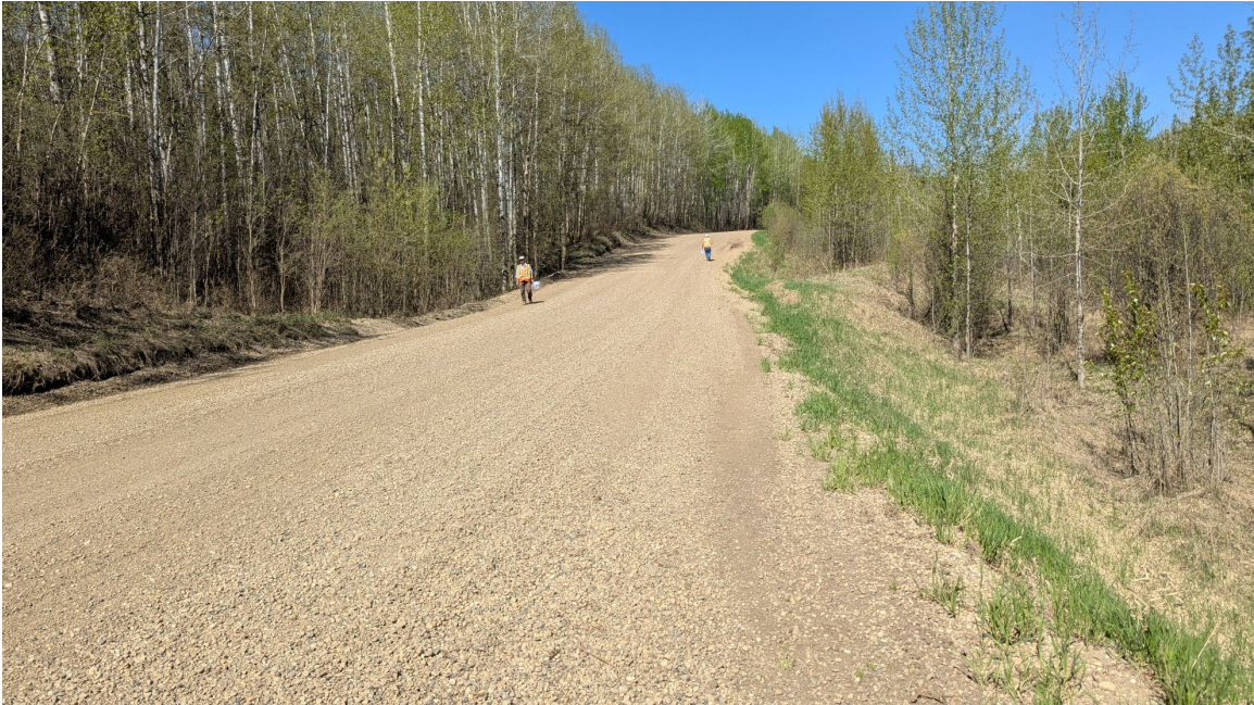
Site 2, Photo 1 – Looking northeast along highway where scarp cracks had previously been visible (since graded over).
