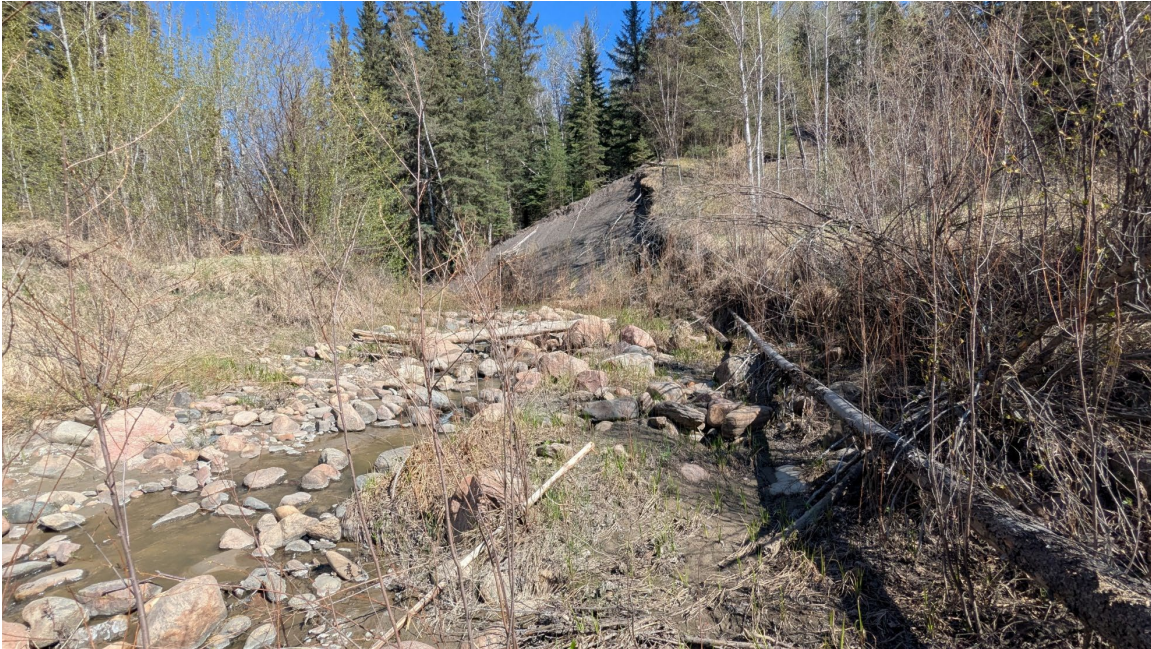
Site 1, Photo 3 – Looking north at creek bank slumping upstream of the culvert inlet.
