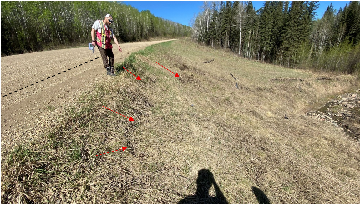
Site 1, Photo 4 – Looking west at the tension crack (red arrows) proximity to the shifted gravel edge (the dashed line is the approximate previous roadway edge).
