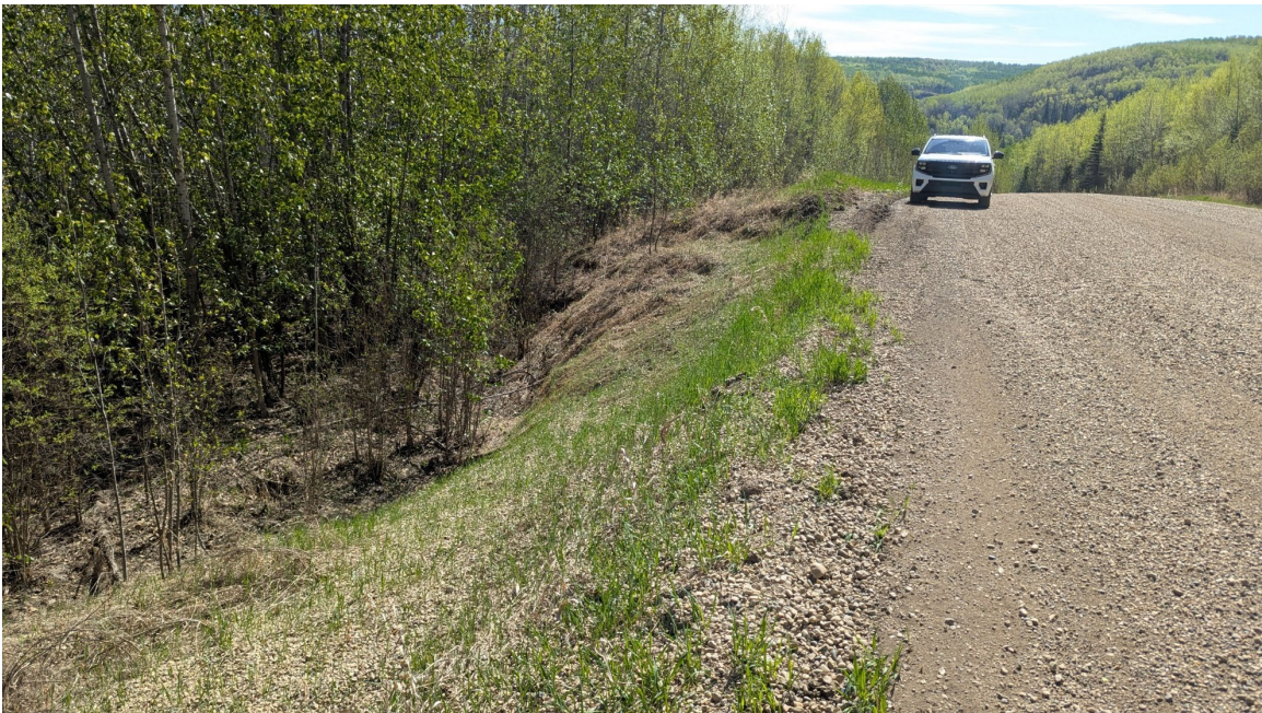
Site 2, Photo 2 – Looking southeast where scarp crack is visible on the east side of the highway.
