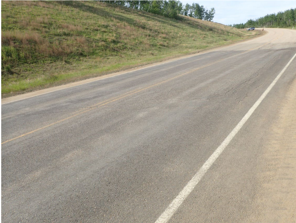
Photo 1 – Looking southeast at crack pattern on highway patch.
