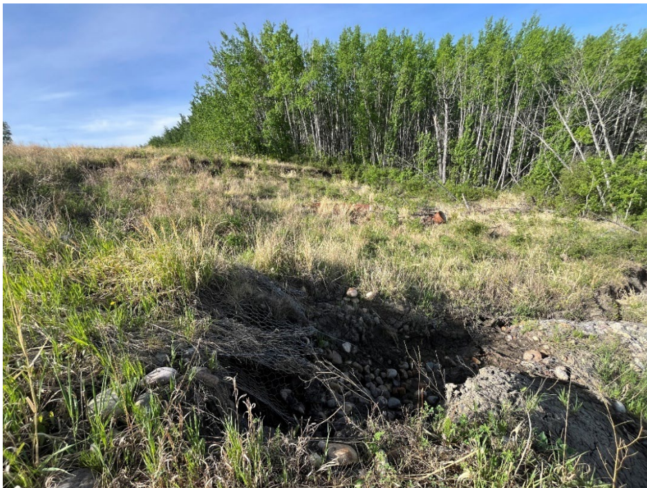
Photo 22 – Looking south at slide at km 14.45 located adjacent to south gabion basket swale.
