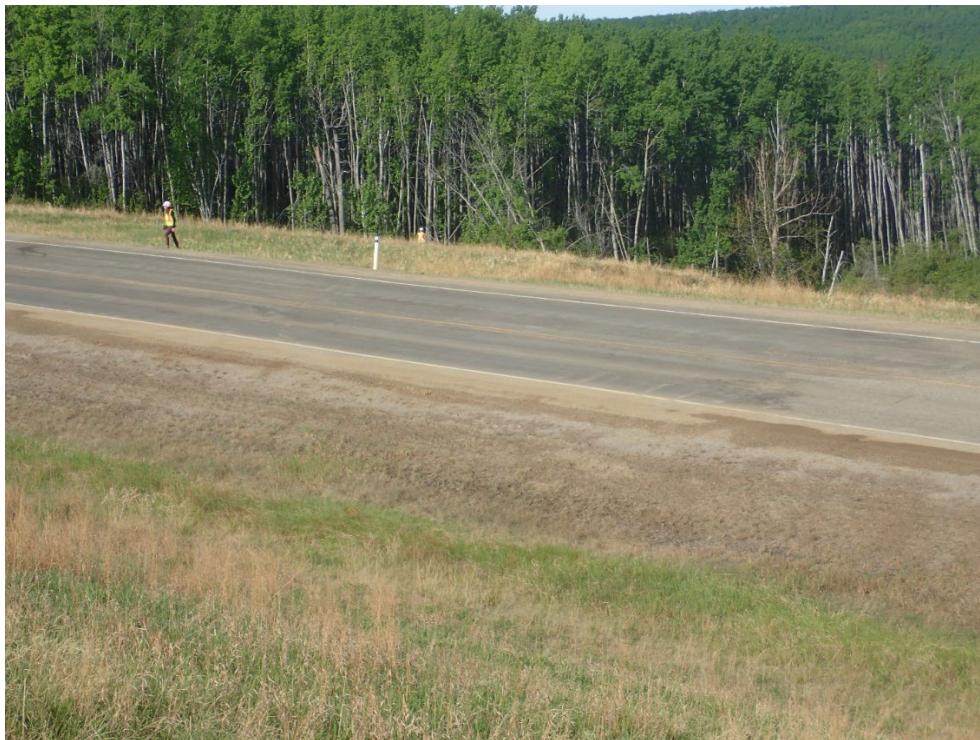
Photo 8 – Looking southwest at highway patch.
