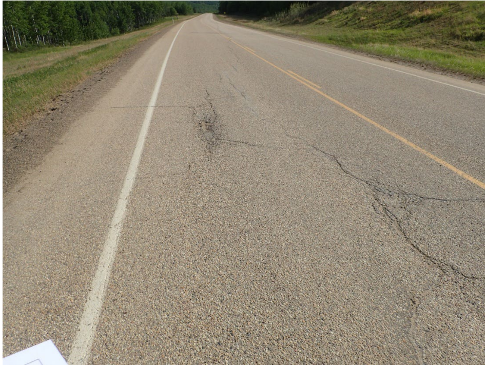
Photo 11 – Looking north at crack pattern and dip along SBL.
