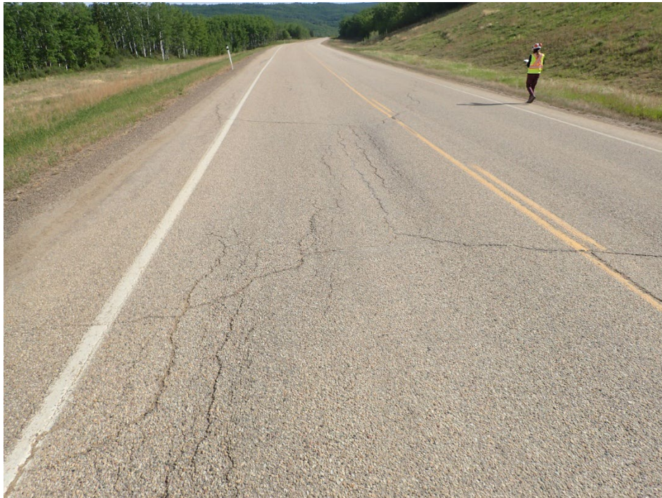
Photos 9 and 10 – Looking north at crack patterns along SBL.
