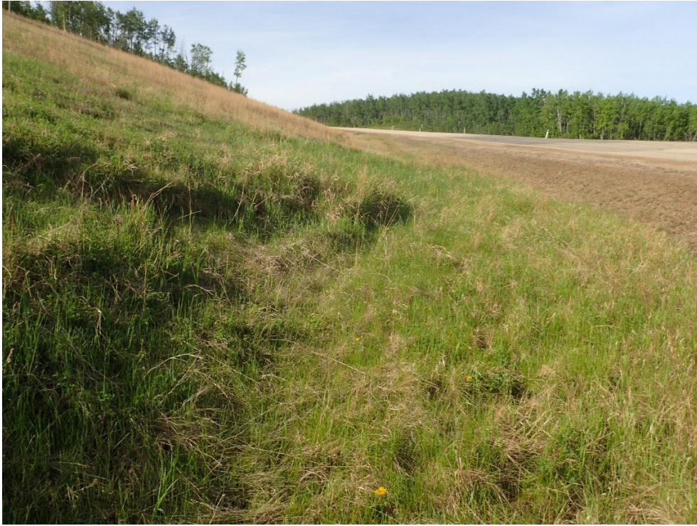
Photo 5 – Looking south at lower slump where vegetative growth was noted.
