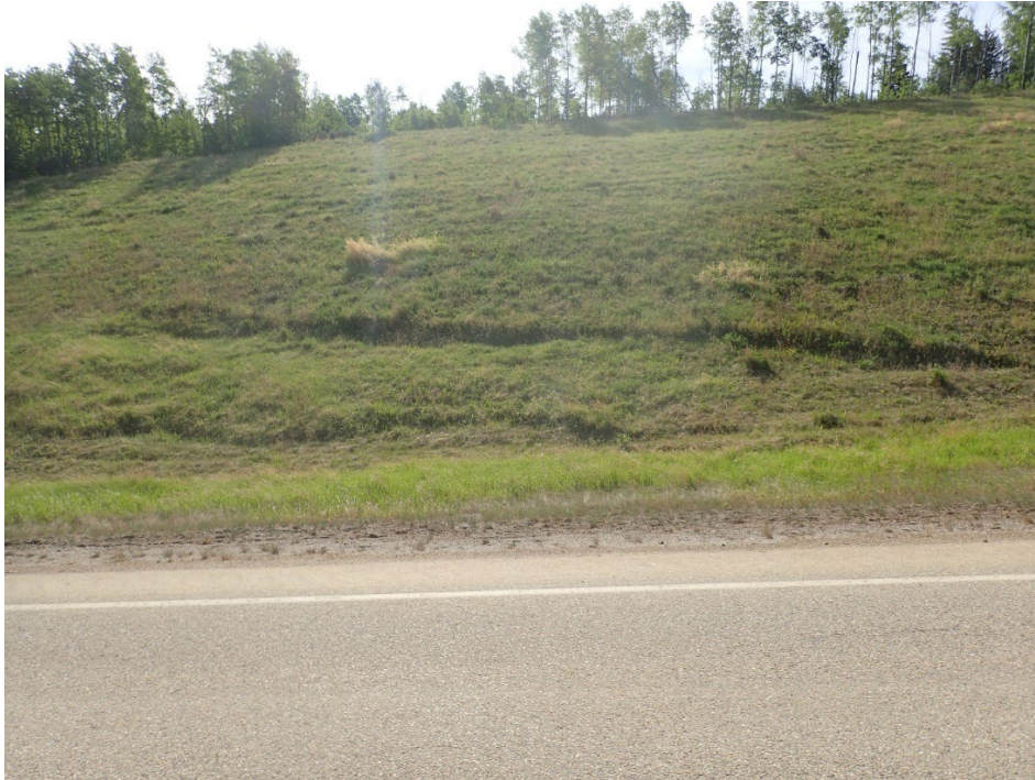
Photo 13 – Looking east at scarp crack at north end of site on east backslope.
