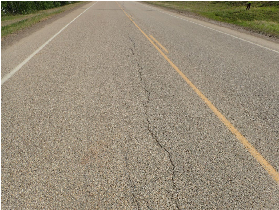
Photo 12 – Looking north at crack pattern along SBL at north end of site.
