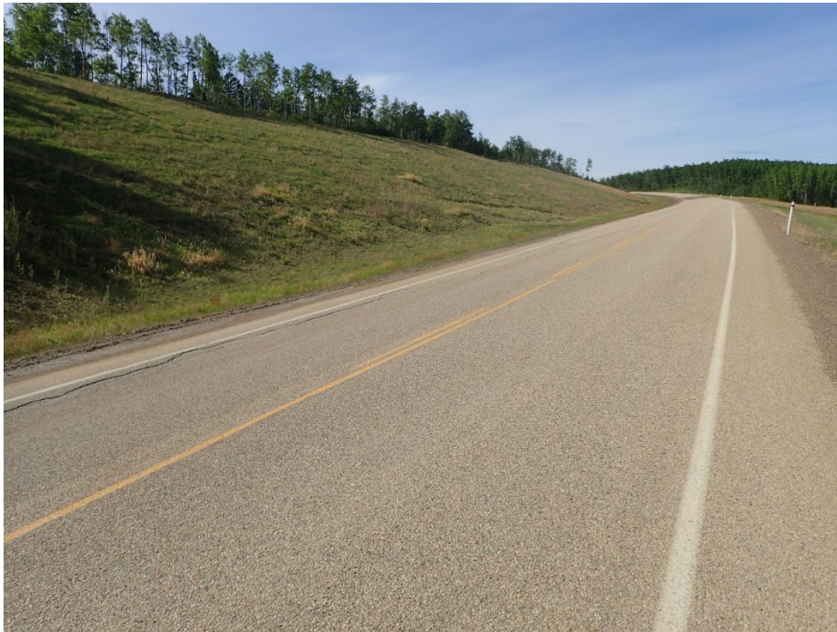
Photo 16 – Looking southeast at crack pattern along NBL at north end of site with backslope scarp in the background.
