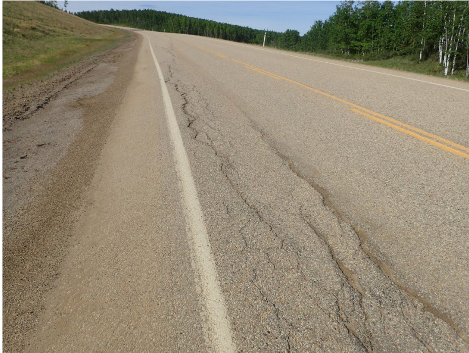
Photo 15 – Looking south at crack pattern along NBL at north end of site.
