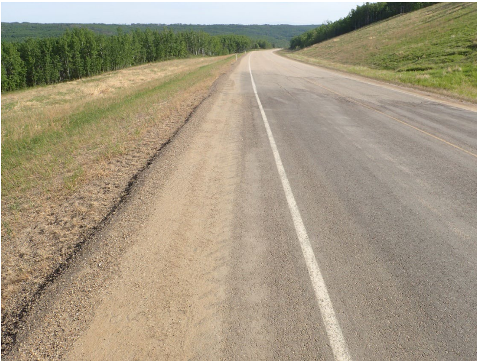
Photo 2 – Looking north at extended cracks along fog line and outside highway patch.
