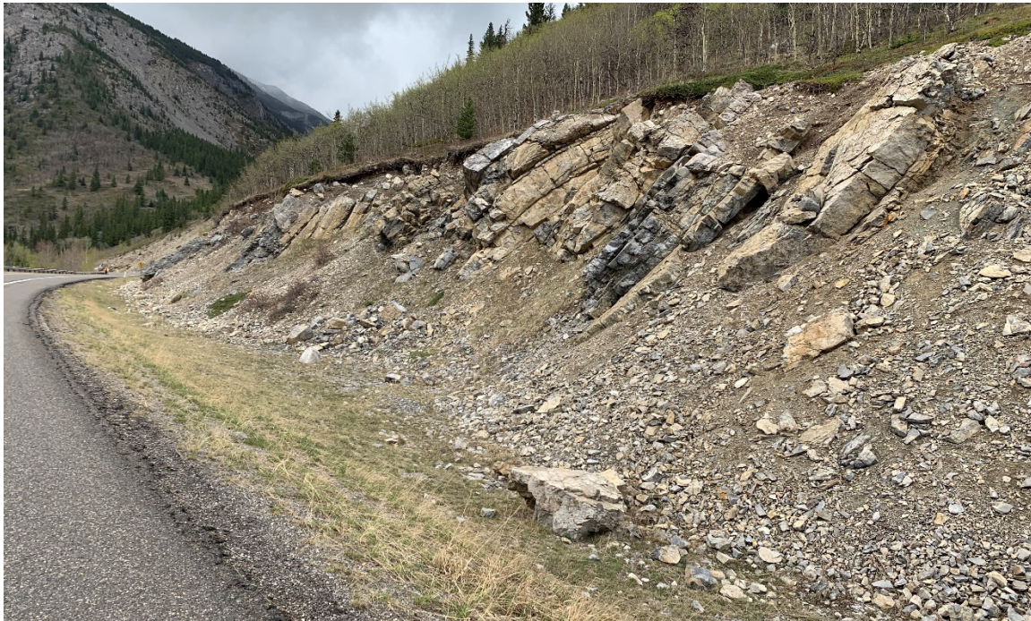
Photo 7 S070-III: Bedrock fracturing leading to future rockfall blocks. Large rock noted in ditch was there during the 2022 inspection. Photo taken facing north on May 9, 2023.
